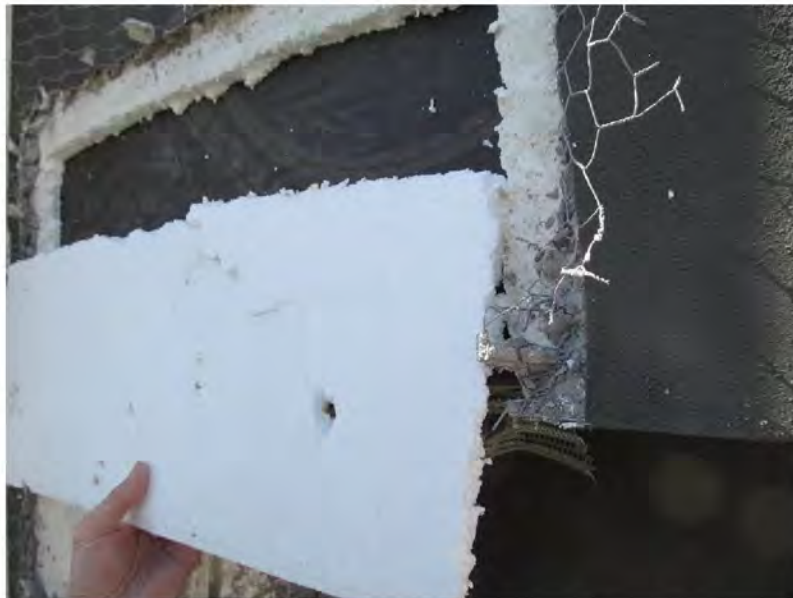
March 10, 2021, Disc IT7, Photograph 117, JJF, Building D, EPS foam board installed over WRB with vertical grooves generally missing at the back face.
