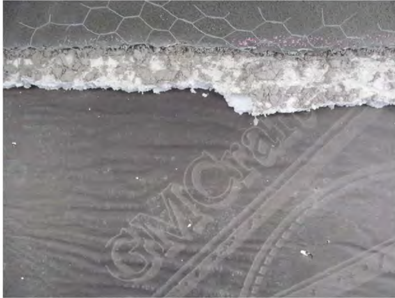
March 9, 2021, Disc IT6, Photograph 271, SSR, Building A, EPS foam board installed tight to GMCraft WRB and vertical grooves generally missing at the inner face.
