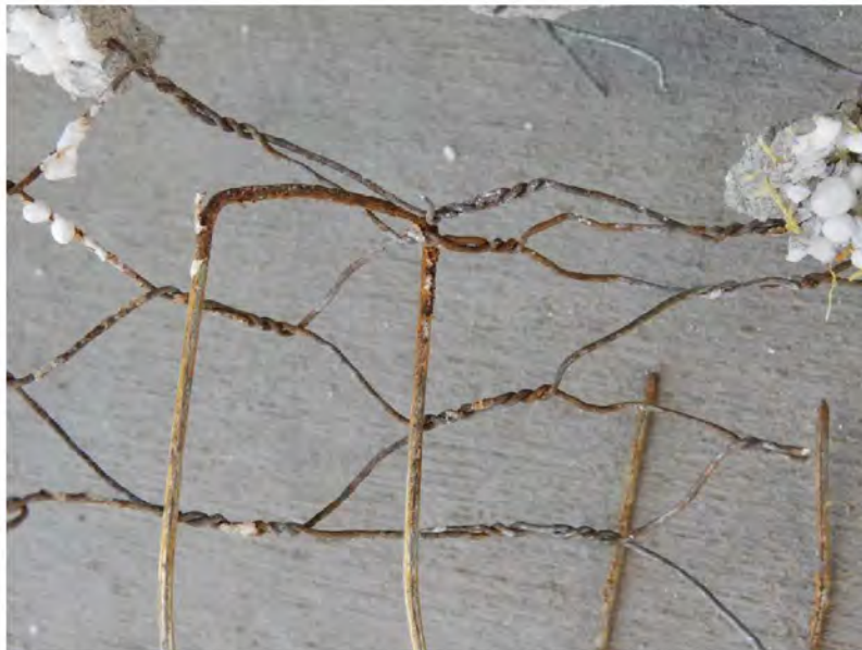
March 10, 2021, Disc IT9, Photograph 87, PER, Building C, rusted staples and lath
