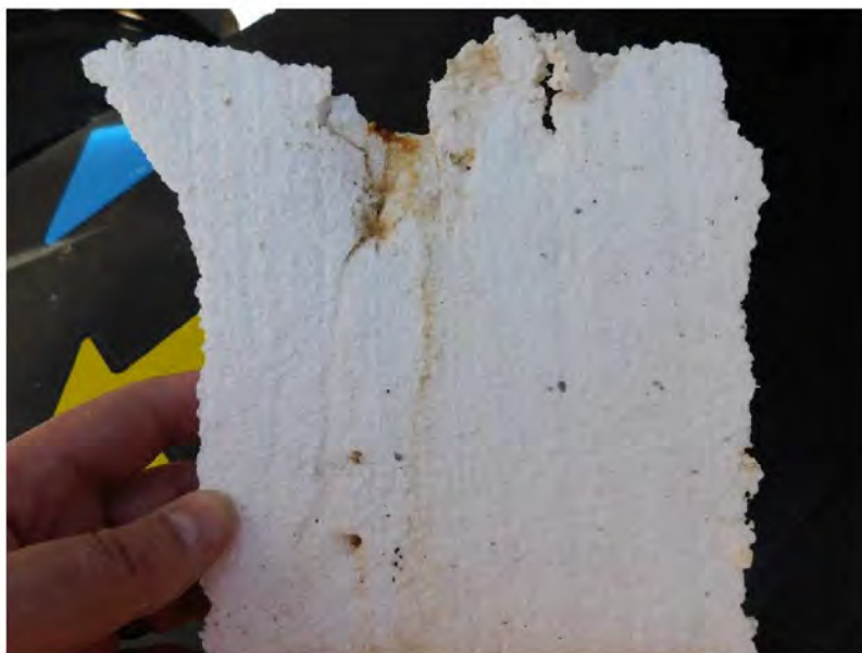
March 10, 2021, Disc IT9, Photograph 95, PER, Building C, EPS foam board installed tight to WRB and vertical grooves generally missing at the back face. Note corrosion from the nails on the EPS foam board.
