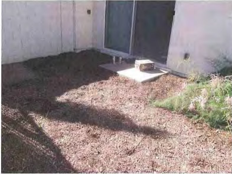
December 19, 2018, Disc OBS1, Photograph 80, JBF, east elevation of Building D - Unit 3111, poor slope of grade away from foundation.
