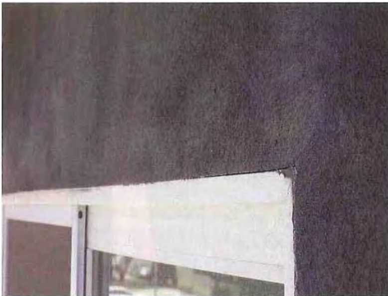
May 13, 2019, Disc IT2, Photograph 34, ELF, west elevation of Building D - Unit 3115, no sheet metal flashing at head of window opening.
