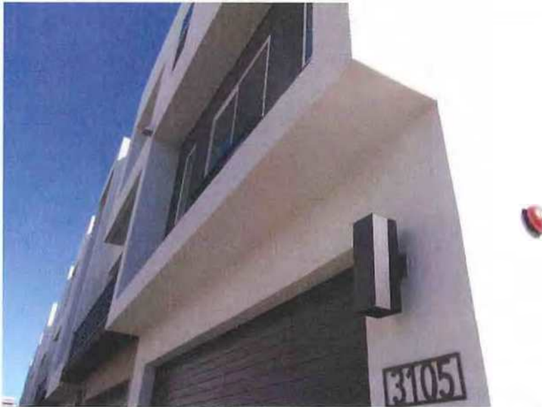
December 19, 2018, Disc OBS1, Photograph 18, JBF, west elevation of Building D - Unit 3105, no weep mechanism at base of stucco at soffit.
