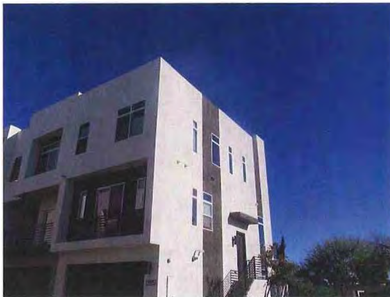
December 19, 2018, Disc OBS1, Photograph 5, JBF, south elevation of Building D, vertical control joint only provided at corners of windows. This was common of north and south elevations at all buildings.
