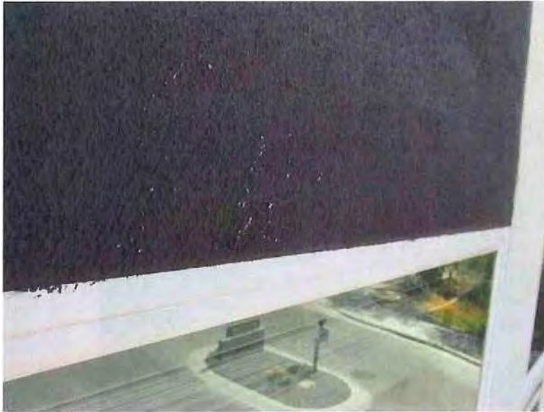
May 13, 2019, Disc IT1, Photograph 142, JBF, north elevation of Building C - Unit 3127, no sheet metal flashing at head of window opening.
