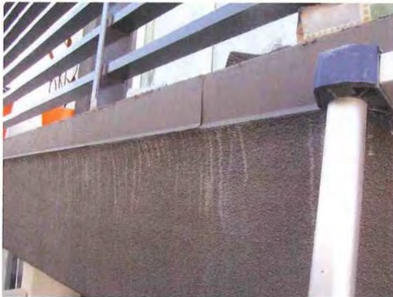
May 13, 2019, Disc IT1, Photograph 145, JBF, east elevation of Building C - Unit 3127, metal flashing at leading edge of balcony is inset from stucco. Stucco built up beyond flashing at this location.
