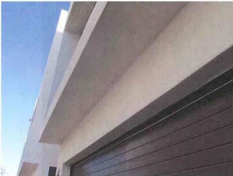
December 19, 2018, Disc OBS1, Photograph 40, JBF, west elevation of Building D - Unit 3115, no flashing or weep mechanism provided at top of garage door opening
