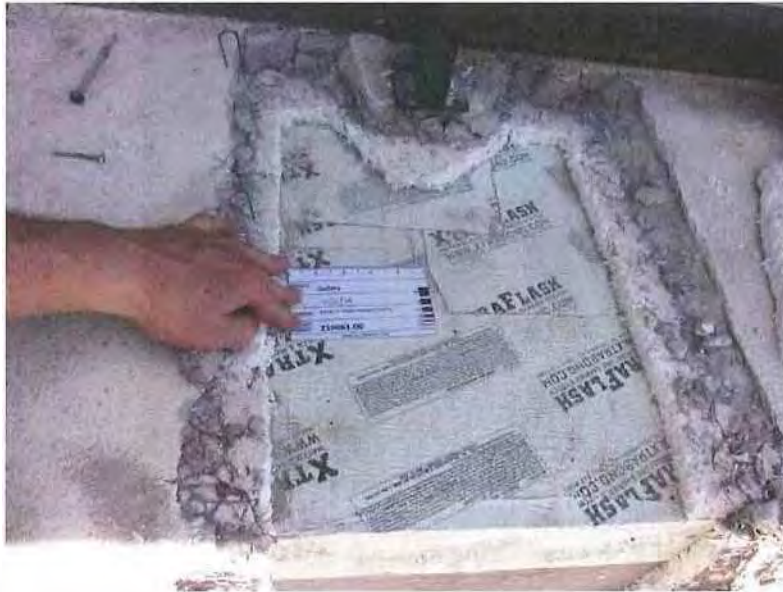
May 13, 2019, Disc II2, Photograph 21, ELF, west elevation of Building D - Unit 3115, XtraFlash membrane under stucco. Stain through holes in membrane.
