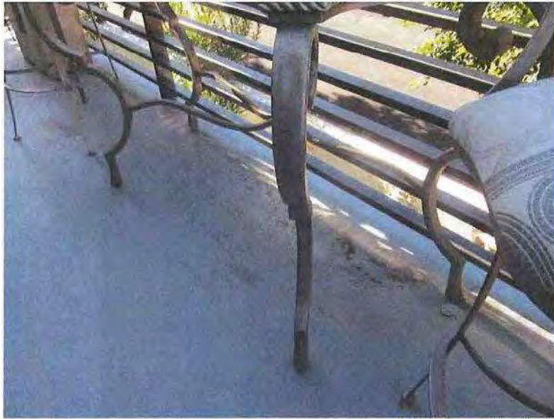
December 19, 2018, Disc OBS1, Photograph 167, JBF, Building A - Unit 3124, evidence of water ponding is present at leading edge of balcony.
