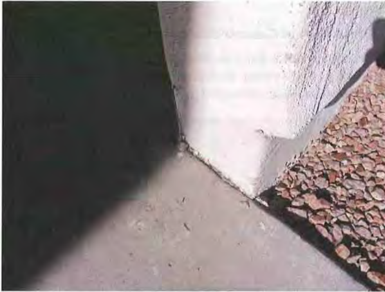
December 19, 2018, Disc OBS1, Photograph 137, JBF, east elevation of Building B - Unit 3116, no isolation joint between concrete flatwork and structural foundation.
