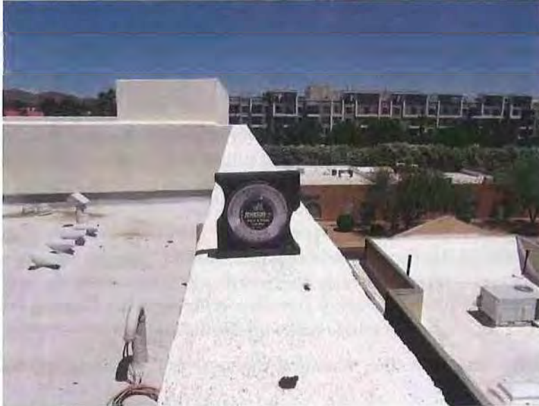
May 13, 2019, Disc IT1, Photograph 33, JBF, Building C - Unit 3125, stucco does not slope at parapet cap.
