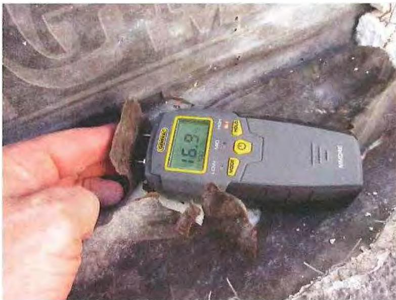
May 14, 2019, Disc II4, Photograph 13, ELF, west elevation of Building C - Unit 3123, high moisture content in building paper below stucco over self-adhered membrane.
