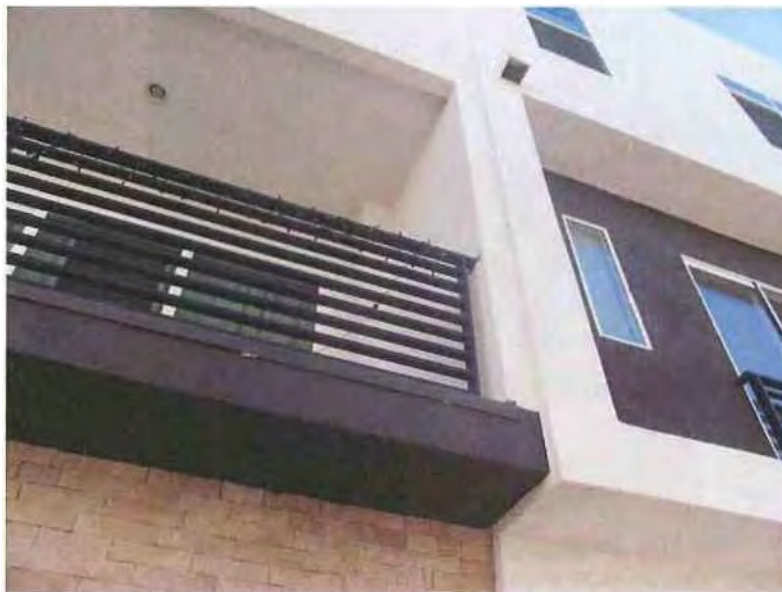
December 19, 2018, Disc OBS1, Photograph 24, JBF, west elevation of Building D - Units 3111 & 3113, no weep mechanism at base of stucco at soffits.
