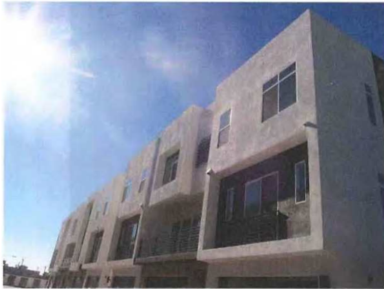
December 19, 2018, Disc OBS1, Photograph 110, JBF, east elevation of Buildings A and B, no control/movement joints provided.
