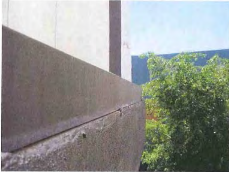
May 13, 2019, Disc IT1, Photograph 110, JBF, north elevation of Building B - Unit 3116, metal flashing at leading edge of roof is inset from stucco.
