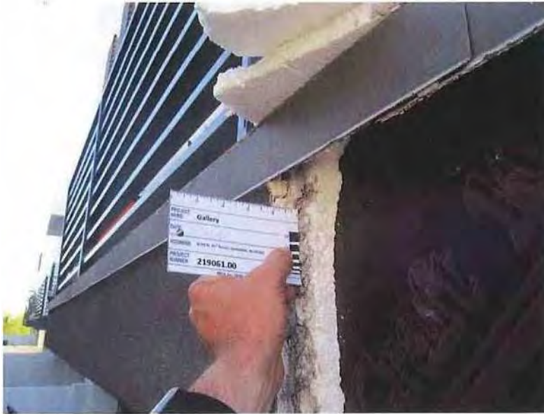
May 13, 2019, Disc IT1, Photograph 176, JBF, east elevation of Building C - Unit 3127, metal flashing at leading edge of balcony is inset from stucco. Stucco built up to approximately 1-inch thick beyond flashing at this location.
