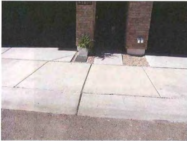
December 19, 2018, Disc OBS1, Photograph 154, JBF, east elevation of Building B, drainage adjacent to foundation bound by concrete flatwork.
