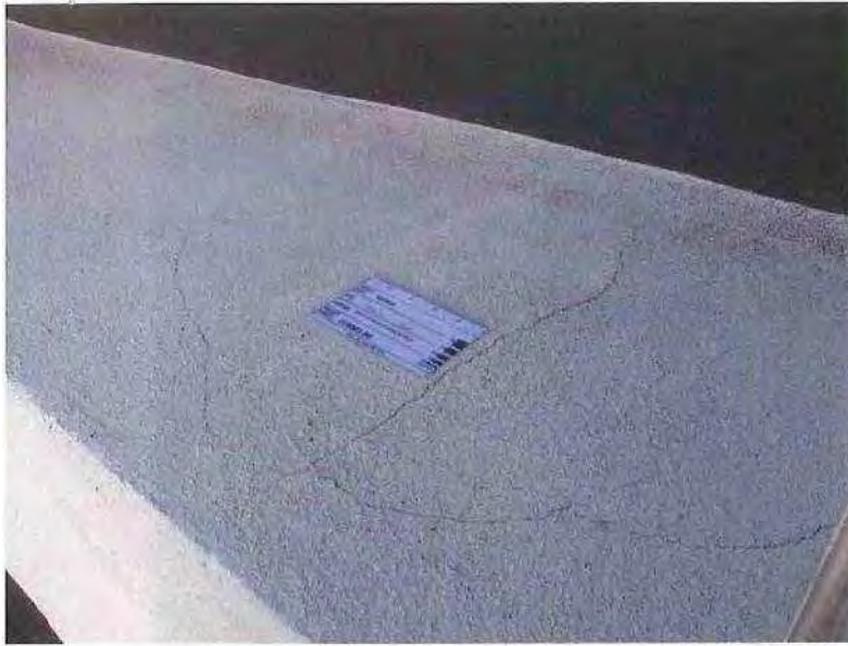
May 14, 2019, Disc IT4, Photograph 26, ELF, west elevation of Building C - Unit 3125, cracking of stucco on window shelf indicative of water entrapment.
