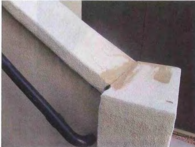
December 19, 2018, Disc OBS1, Photograph 45, JBF, east stairs between Buildings C and D, cracking and separation of stair wall indicative of differential movement.
