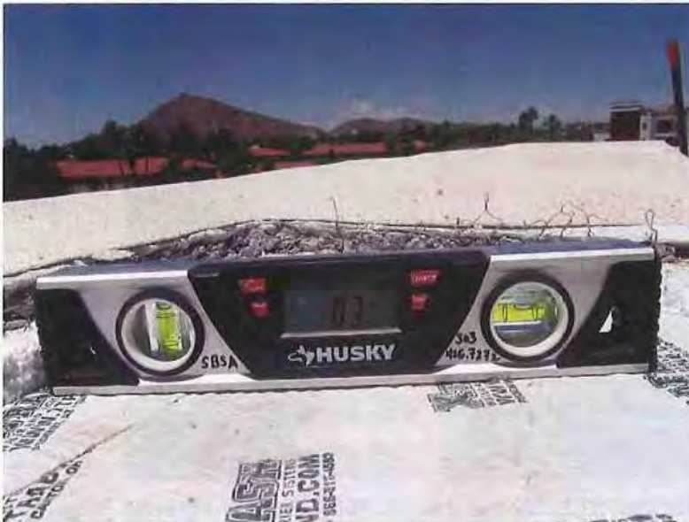
May 13, 2019, Disc IT1, Photograph 98, JBF, Building C - Unit 3125, stucco does not slope at parapet cap.
