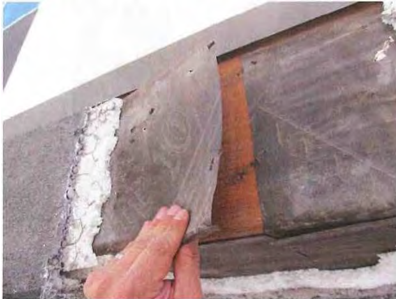
May 13, 2019, Disc IT1, Photograph 128, JBF, north elevation of Building B - Unit 3116, one layer of GMCraft 10 paper does not provide minimum water-resistance rating of 60-minutes in accordance with ESR-3529.
