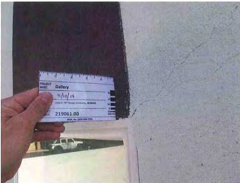
May 14, 2019, Disc IT3, Photograph 12, JBF, south elevation of Building B - Unit 3104, no expansion joints provided between stucco and window. A diagonal stucco crack is present at this location.
