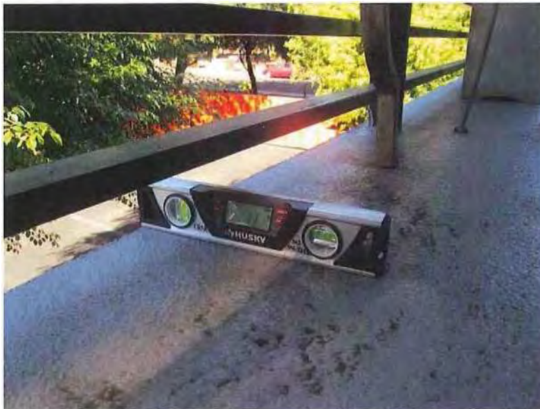
December 19, 2018, Disc OBS1, Photograph 163, JBF, Building A - Unit 3124, balcony slope measured to be 1.1-percent away from leading edge and evidence of water ponding is present.
