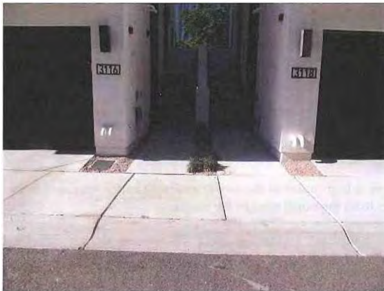
December 19, 2018, Disc OBS1, Photograph 156, JBF, west elevation between Buildings C and D, poor slope of grade between buildings.
