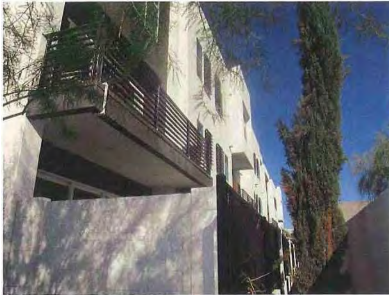
December 19, 2018, Disc OBS1, Photograph 13, JBF, east elevation of Buildings C and D, no control/movement joints provided.
