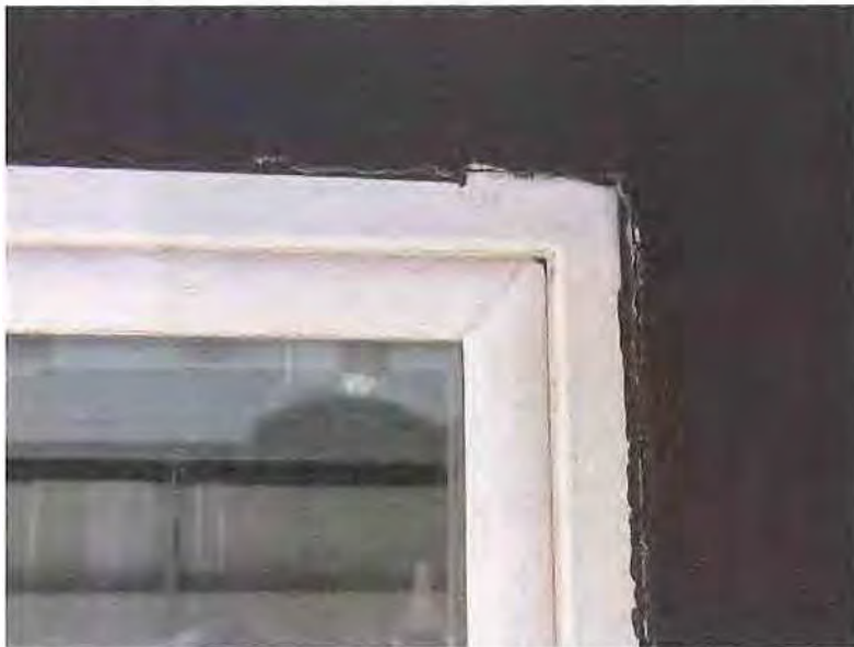
May 13, 2019, Disc IT2, Photograph 33, ELF, west elevation of Building D – Unit 3115, no expansion joints provided between stucco and window. Cracking is present at this interface.
