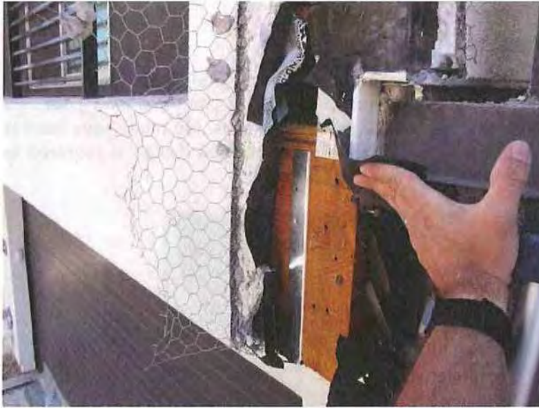
May 13, 2019, Disc II1, Photograph 50, JBF, west elevation of Building D - Unit 3113, open stud framing with no exterior sheathing.
