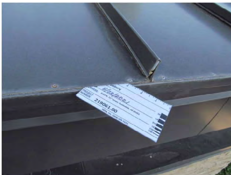
August 23, 2021, Disc OBS8, Photograph 16, JFF, pool cabana, unsealed edge.
