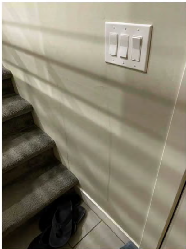
Burg Simpson provided photograph, Bates Number GALLERY-JONES_3104-000010, Unit 3104, water leak at front door light switch and hole in interior drywall.
