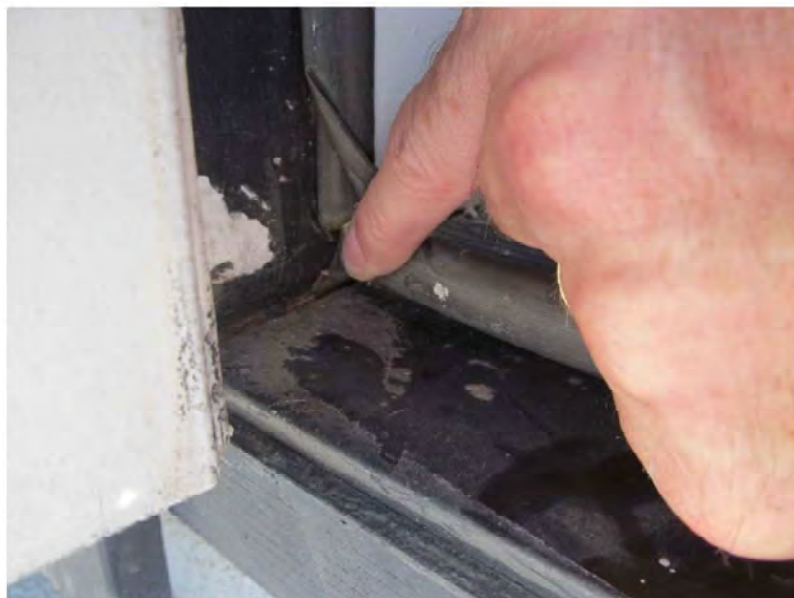
August 23, 2021, Disc OBS8, Photograph 29, JJF, Unit 3106, roof penthouse door, unsealed joint at door threshold to jamb.
