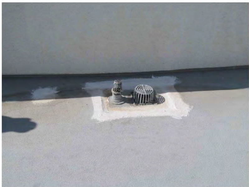
August 23, 2021, Disc OBS8, Photograph 86, JJF, Unit 3106, roof, temporary repair at perimeter of roof drain sump.
