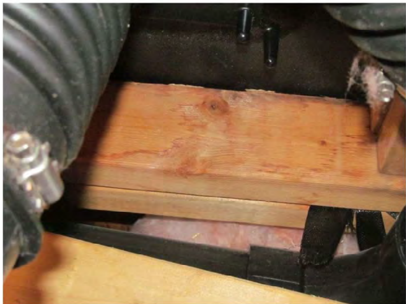
August 23, 2021, Disc OBS8, Photograph 72, JJF, Unit 3106, bedroom, water-stained wood blocking under perimeter edge of preformed drain sump nearest to parapet wall.
