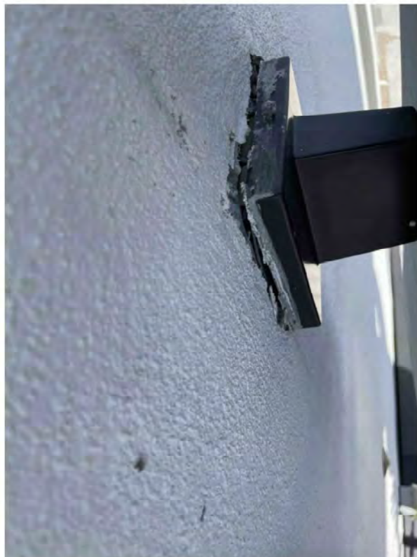
Nautilus-provided photograph, Bates Number GALLERY-NBC_004992, Unit 3104, light fixture protruding from stucco with openings around the perimeter.
