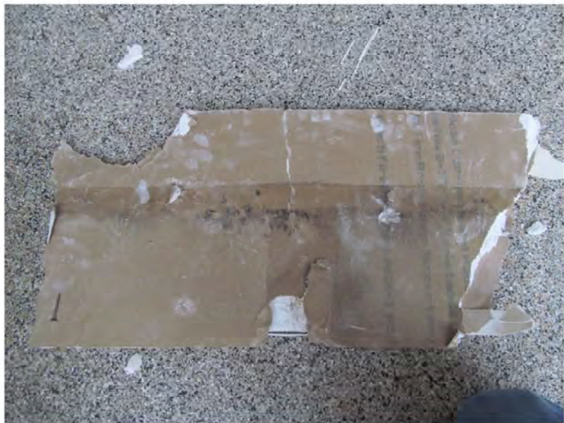
August 23, 2021, Disc OBS8, Photograph 51, JJF, Unit 3106, bedroom ceiling, water-damaged ceiling drywall. Refer to photograph above.
