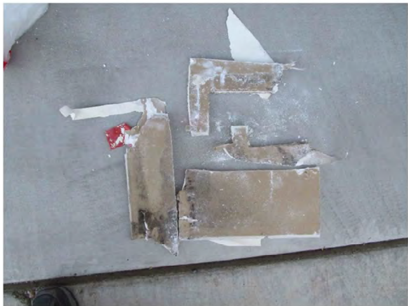
August 23, 2021, Disc OBS8, Photograph 48, JJF, Unit 3106, laundry room ceiling, water-damaged ceiling drywall around vent. Refer to photograph above.
