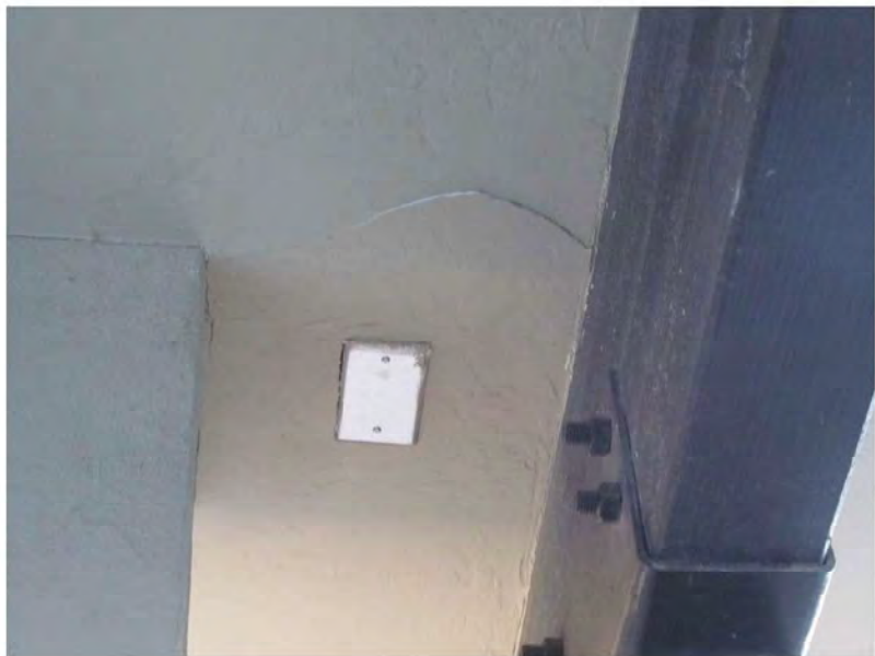
August 23, 2021, Disc OBS8, Photograph 3, JJF, pool cabana, cracked ceiling finish.
