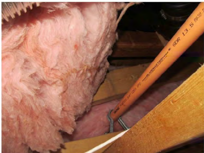
August 23, 2021, Disc OBS8, Photograph 76, JJF, Unit 3106, laundry room, water-stained batt insulation.
