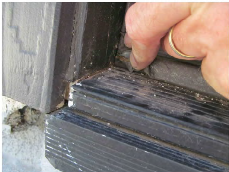
August 23, 2021, Disc OBS8, Photograph 187, JJF, Unit 3123, roof penthouse door, unsealed joint at door threshold to jamb.
