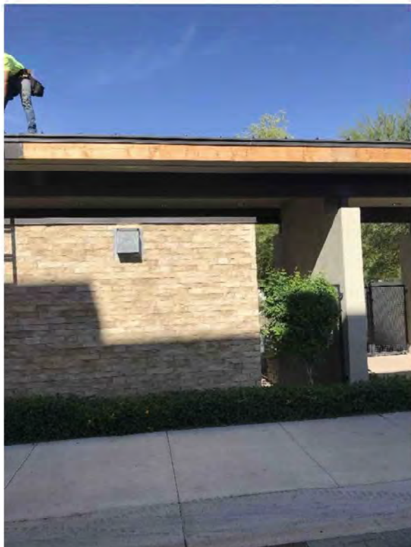
Nautilus-provided photograph, previous repair of pool cabana ceiling.
