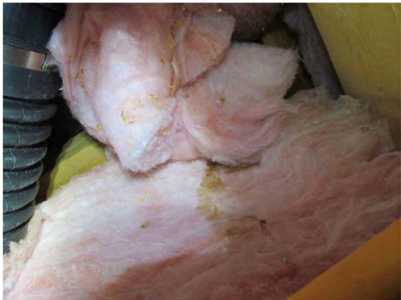
August 23, 2021, Disc OBS8, Photograph 65, JJF, Unit 3106, bedroom, water-stained batt insulation.
