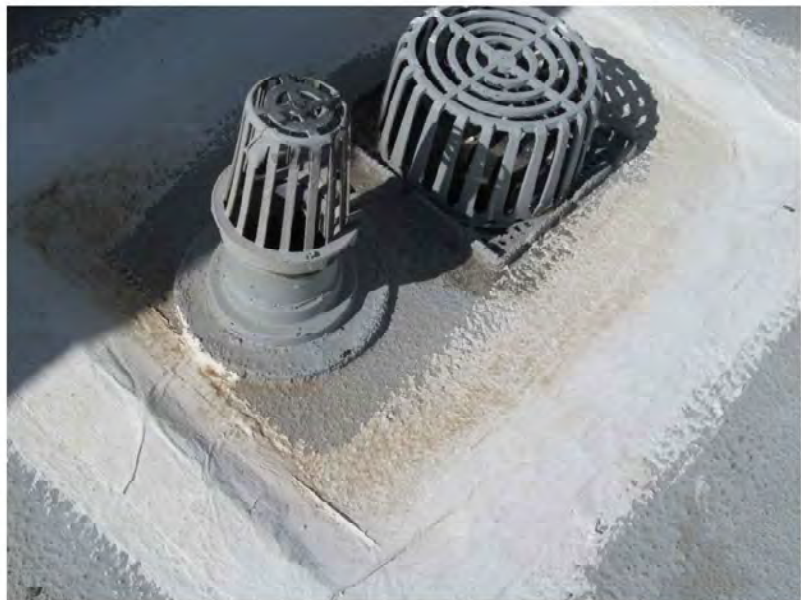
August 23, 2021, Disc OBS8, Photograph 88, JFF, Unit 3106, roof, temporary repair at perimeter of roof drain sump.
