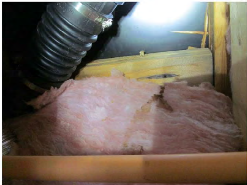
August 23, 2021, Disc OBS8, Photograph 68, JJF, Unit 3106, bedroom, water-stained batt insulation under nail.
