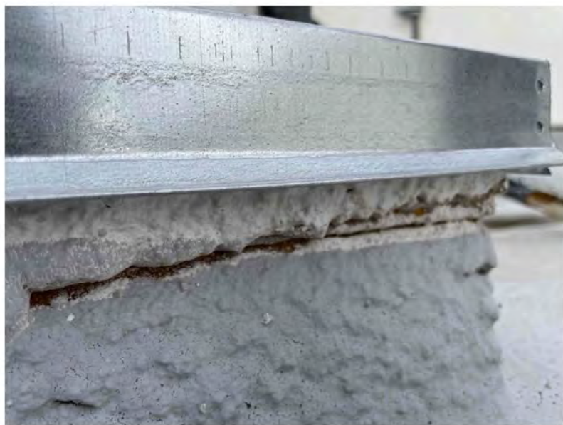
Nautilus-provided photograph, Bates Number GALLERY-NBC_005052, Unit 3112, previous repair failed to seal openings in the roof membrane.
