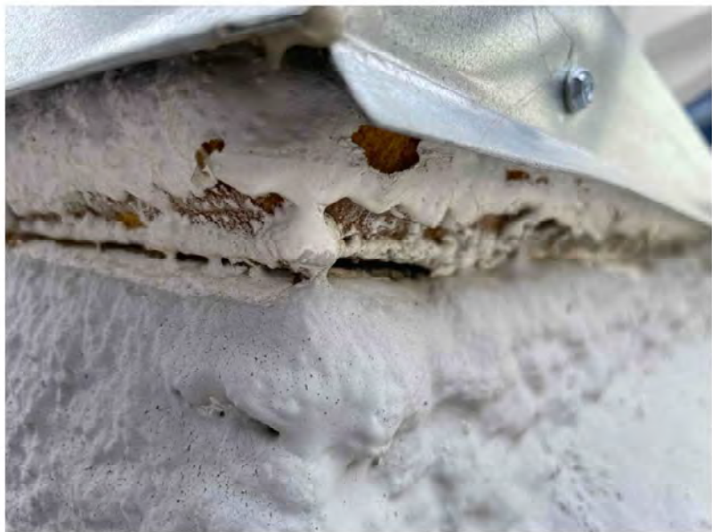
Nautilus-provided photograph, Bates Number GALLERY-NBC_005058, Unit 3112, previous repair failed to seal openings in the roof membrane.
