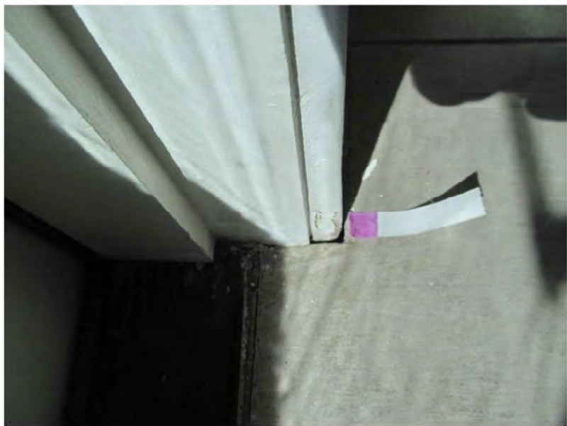
August 23, 2021, Disc OBS8, Photograph 101, JJF, Unit 3106, roof penthouse door, water infiltration under floor tile.
