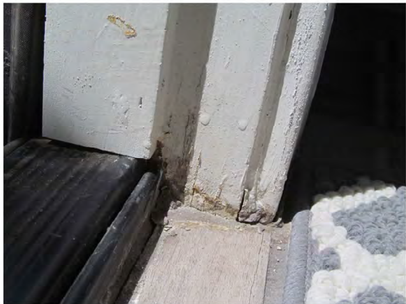
August 23, 2021, Disc OBS8, Photograph 188, JJF, Unit 3123, roof penthouse door, trim damage adjacent to door jamb.
