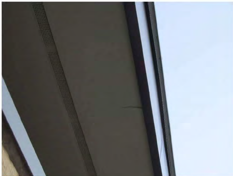
August 23, 2021, Disc OBS8, Photograph 9, JFF, pool cabana, cracked ceiling finish.
