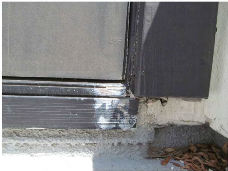
August 23, 2021, Disc OBS8, Photograph 180, JJF, Unit 3123, roof penthouse door, openings at door jamb.
