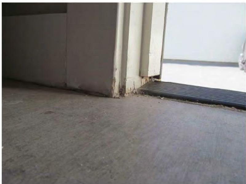
August 23, 2021, Disc OBS8, Photograph 32, JFF, Unit 3106, roof penthouse door, trim damage adjacent to door jamb.
