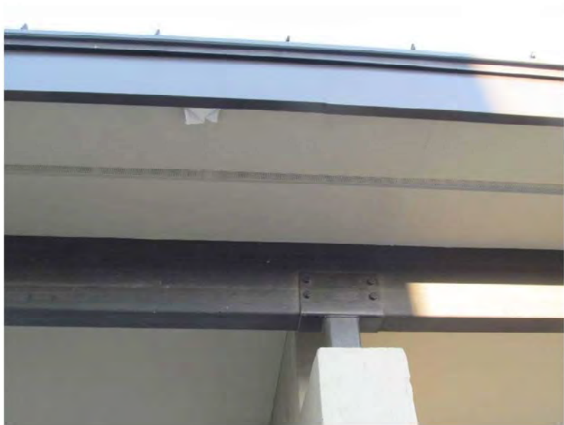
August 23, 2021, Disc OBS8, Photograph 10, JJF, pool cabana, peeling paint and cracked ceiling finish.
