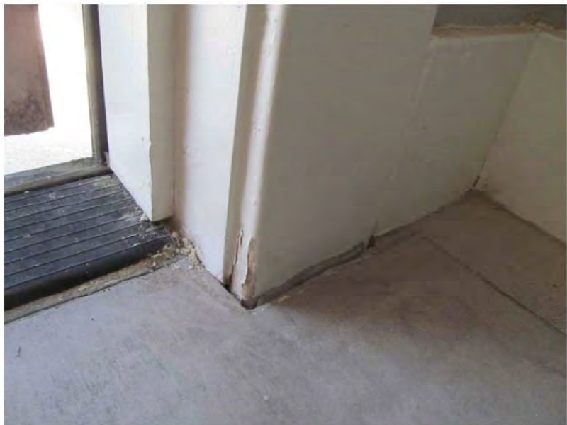
August 23, 2021, Disc OBS8, Photograph 27, JJF, Unit 3106, roof penthouse door, trim damage adjacent to door jamb.
