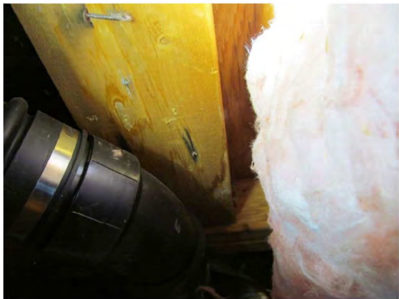
August 23, 2021, Disc OBS8, Photograph 70, JJF, Unit 3106, bedroom, water-stained wood blocking under perimeter edge of preformed drain pan farthest from parapet wall.
