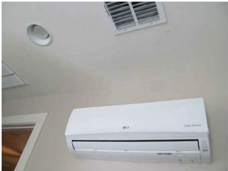
August 23, 2021, Disc OBS8, Photograph 108, JJJ, Unit 3104, hallway, ceiling stain and damage at bottom right of vent.
