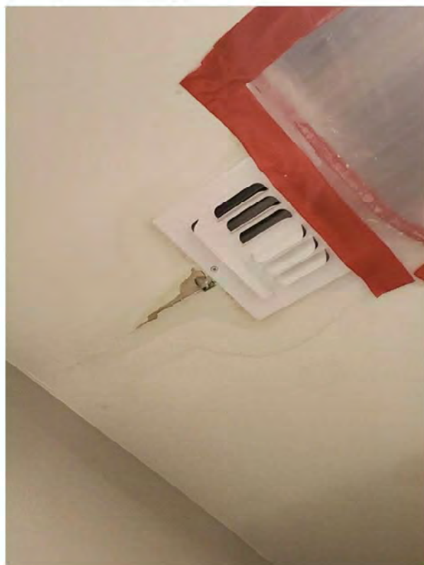
August 14, 2021, Homeowner-provided photograph, Unit 3106, upper floor laundry room, water leak near location of roof drain.
