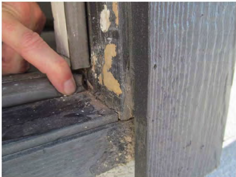
August 23, 2021, Disc OBS8, Photograph 34, JFF, Unit 3106, roof penthouse door, unsealed joint at door threshold to jamb. Paint delamination consistent with wetting and drying.
