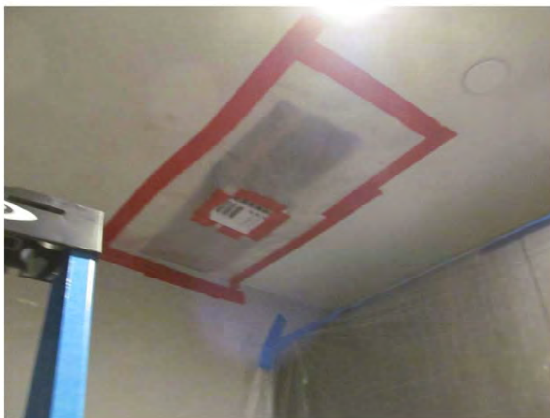
August 23, 2021, Disc OBS8, Photograph 54, JJF, Unit 3106, laundry room, portion of ceiling drywall removed by others.
