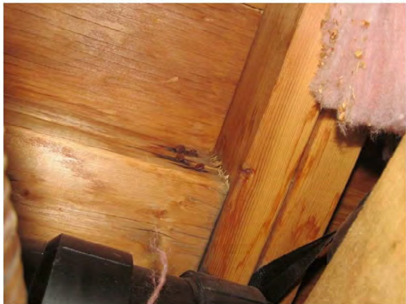
August 23, 2021, Disc OBS8, Photograph 84, JJF, Unit 3106, laundry room, rusted nails and water-stained wood blocking and top chord of roof truss.
