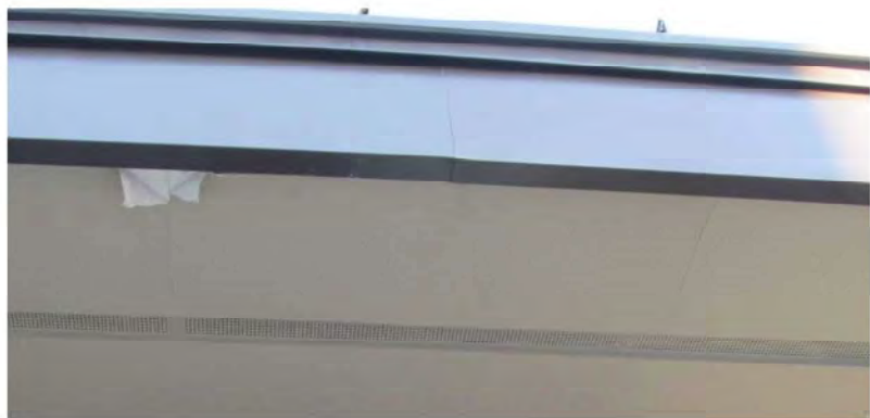
August 23, 2021, Disc OBS8, Photograph 10 (Enlarged), JJF, pool cabana, peeling paint and cracked ceiling finish. Zoomed in from photograph above.
