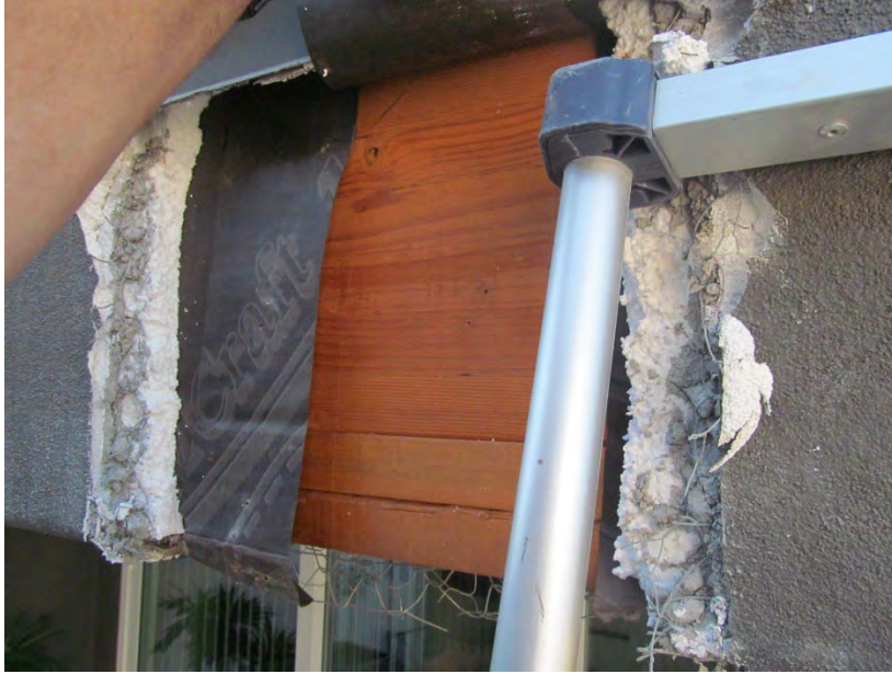
Building C – Rear Elevation, 180 Disc IT1 (No sheathing; however, wood framing with one layer of building paper)
