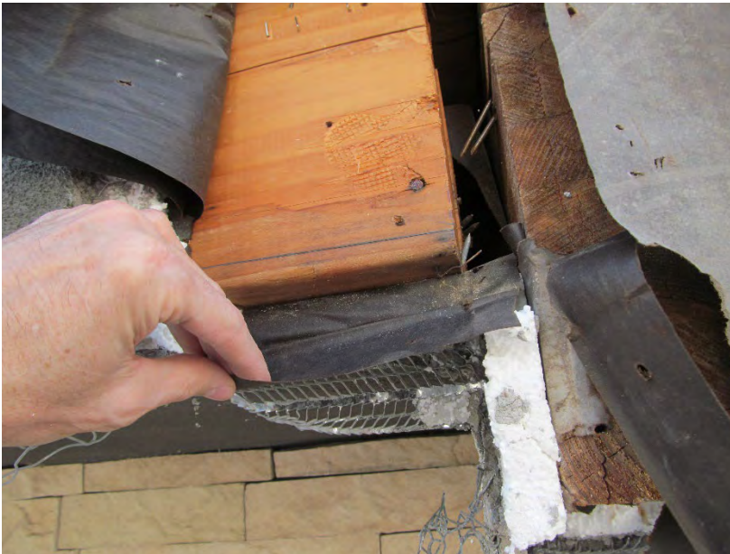
Building B – Front Elevation, 81D Disc IT5 (No sheathing; however, at this location wood framing and deck beam requires 2 layers of building paper which is missing at right beam – Unit 3112)
