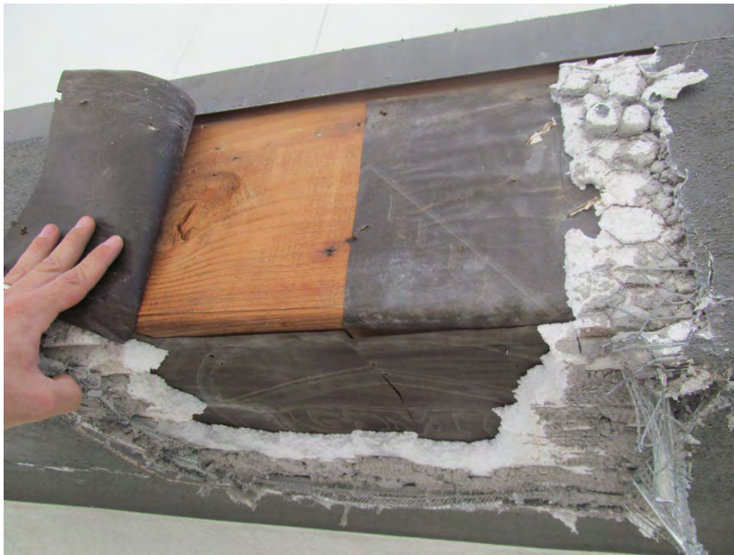
Building B – Right Elevation, 129 Disc IT1 (No sheathing; however, wood framing with one layer of building paper)
