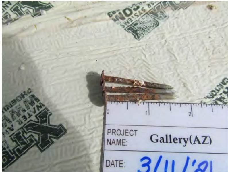
March 11, 2021, Disc IT10, Photograph 132, SSR, Building A, top plate under SAM has stains and rusted fasteners.
