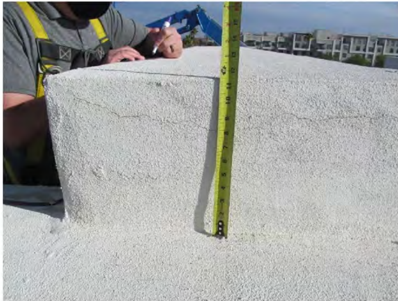
March 11, 2021, Disc IT10, Photograph 3, SSR, Building A, roof parapet wall stucco cracks.
