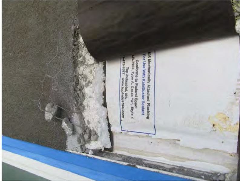
March 9, 2021, Disc IT6, Photograph 286, SSR, Building A, missing flashing at sliding door head.
