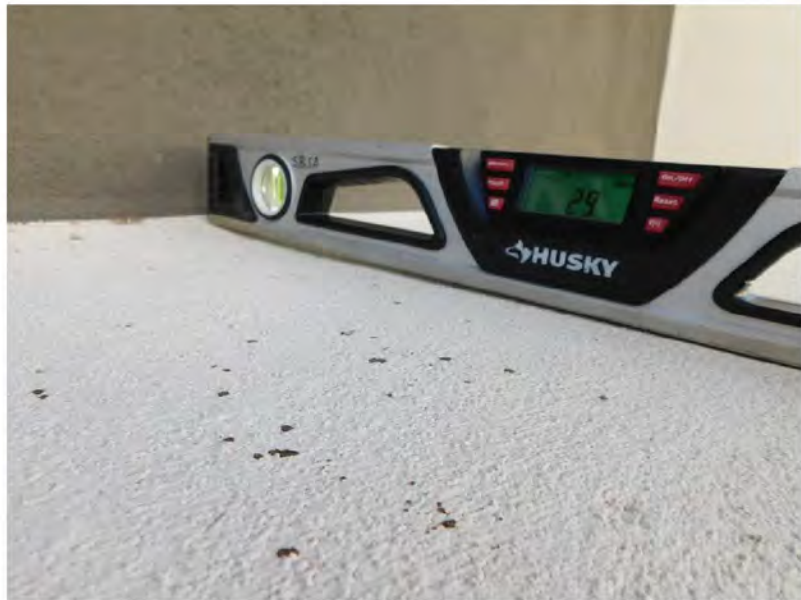
March 10, 2021, Disc IT9, Photograph 25, PER, Building C, stucco pop-out box slopes 2.9-degrees (5-percent) outward.
