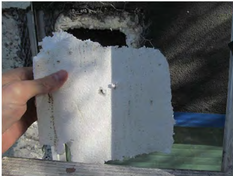
March 10, 2021, Disc IT7, Photograph 20, JJF, Building B, EPS foam board installed over WRB with vertical grooves generally missing at the back face.
