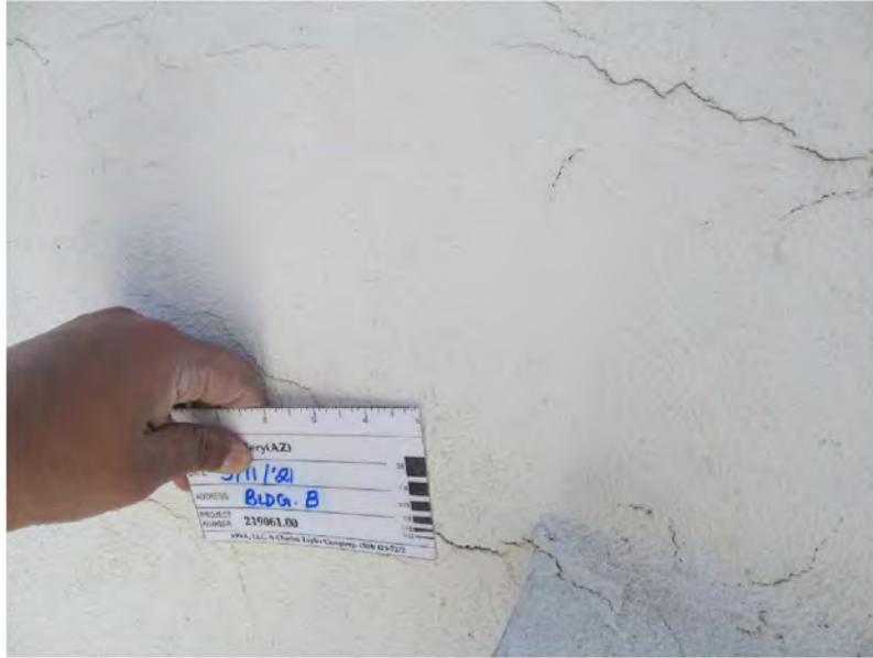
March 11, 2021, Disc IT10, Photograph 170, SSR, Building B, roof parapet wall stucco cracks.
