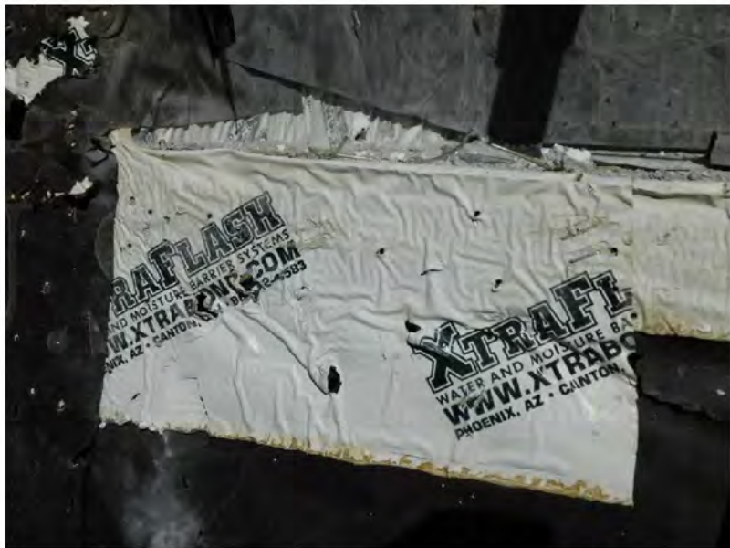
March 10, 2021, Disc IT9, Photograph 185, PER, Building C, holes and stains in Xtraflash SAM allow moisture intrusion.
