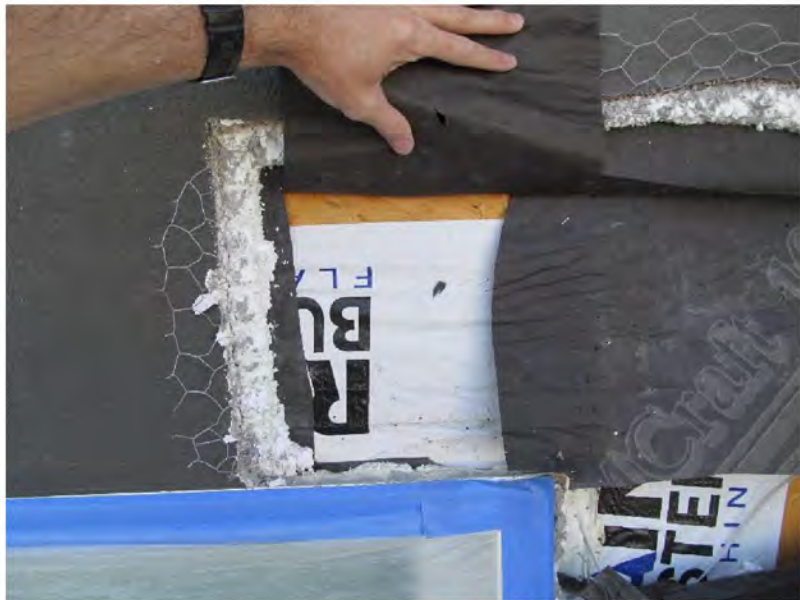
March 10, 2021, Disc IT7, Photograph 212, JJF, Building C, missing flashing at sliding door head.
