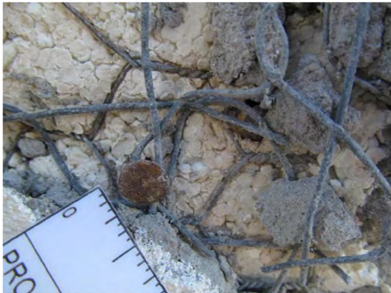
March 10, 2021, Disc IT8, Photograph 96, SSR, Building D, rusted fastener head at EPS foam board.
