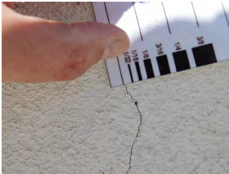
March 11, 2021, Disc OBS7, Photograph 301, PER, Building D, roof parapet wall cracks.
