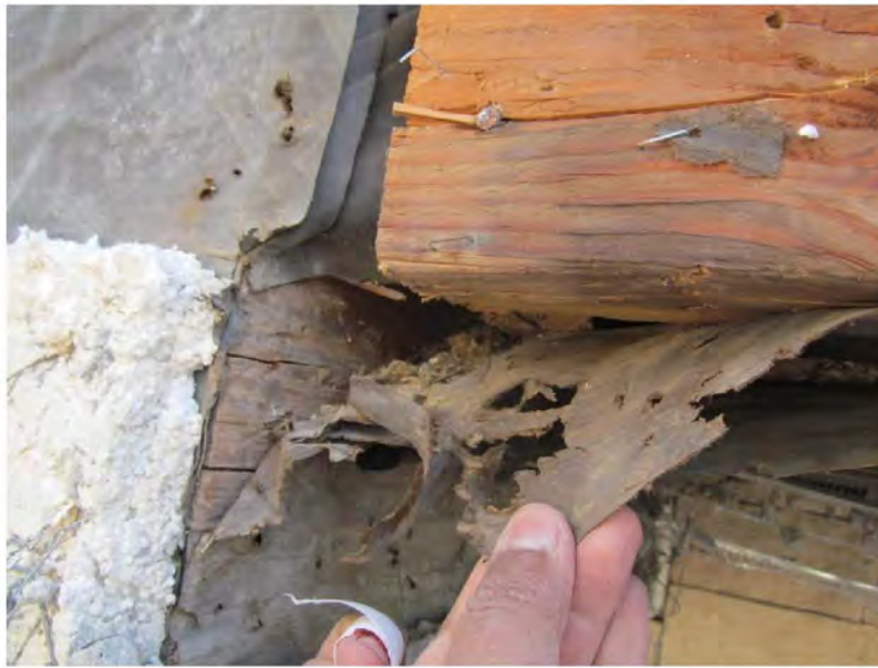
March 10, 2021, Disc IT8, Photograph 120, SSR, Building D, deteriorated WRB over framing with visible stains.
