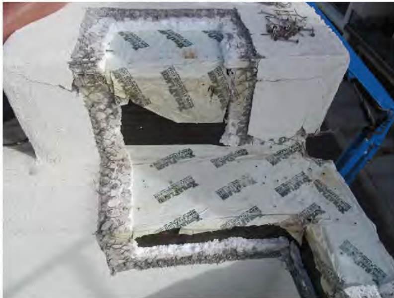
March 11, 2021, Disc IT10, Photograph 102, SSR, Building A, holes and stains in Xtraflash SAM allow moisture intrusion.
