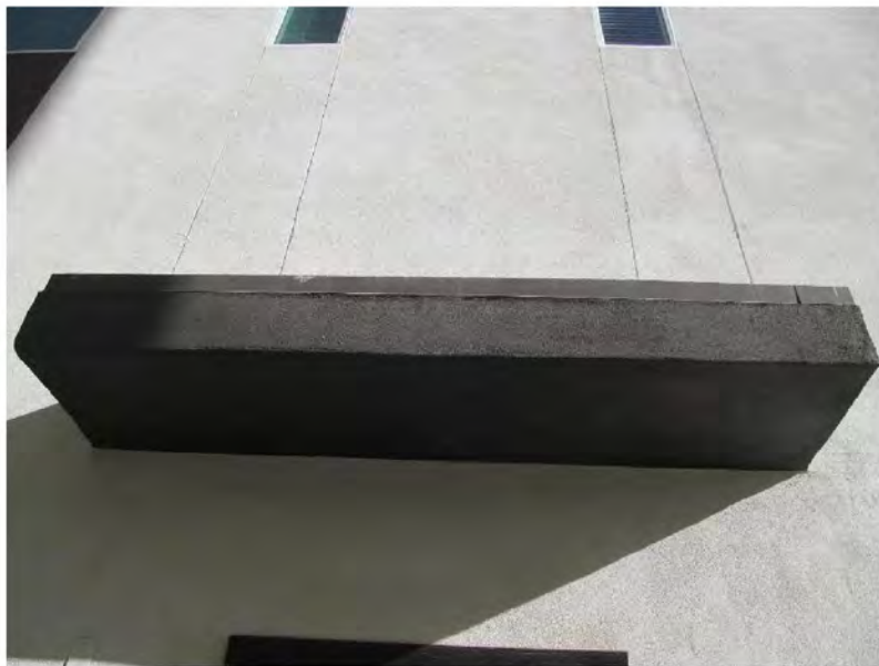
March 11, 2021, Disc OBS6, Photograph 21, JJF, Building C, awning edge flashing inset at stucco.
