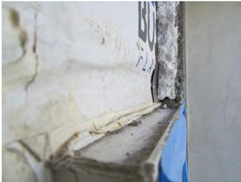
March 9, 2021, Disc IT6, Photograph 280, SSR, Building A, no weep mechanism at stucco termination above window head.
