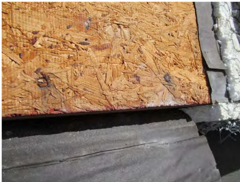
March 9, 2021, Disc IT5, Photograph 164, JJF, Building B, visible stains at sheathing edge and rusted fasteners.
