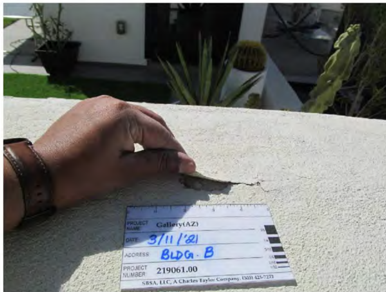
March 11, 2021, Disc IT10, Photograph 244, SSR, Building B, cracks at parapet wall allow stucco to peel off due to the elements and have allowed moisture intrusion.
