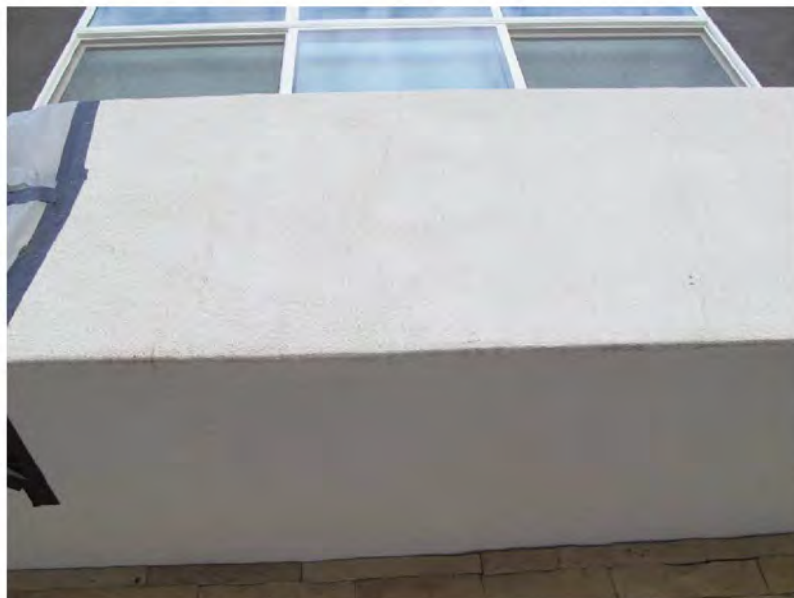
March 11, 2021, Disc OBS6, Photograph 48, JFF, Building C, no weep mechanism at stucco soffits.
