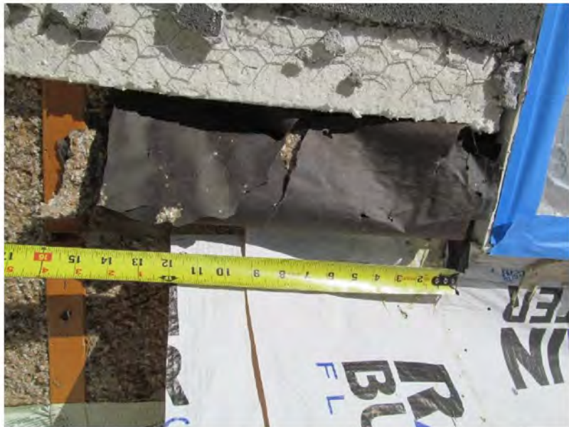
March 10, 2021, Disc IT8, Photograph 248, SSR, Building D - Unit 3111, missing OSB sheathing at existing stud framing.
