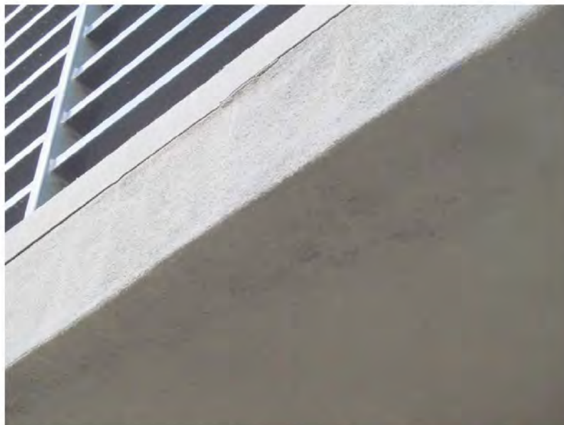
March 11, 2021, Disc OBS6, Photograph 58, JFF, Building C, deck edge flashing inset at stucco.
