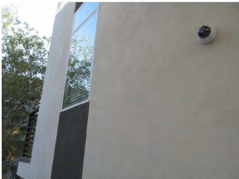
March 10, 2021, Disc OBS 5, Photograph 28, SSR, Building A, horizontal stucco crack. See below photo for close-up view of damage.
