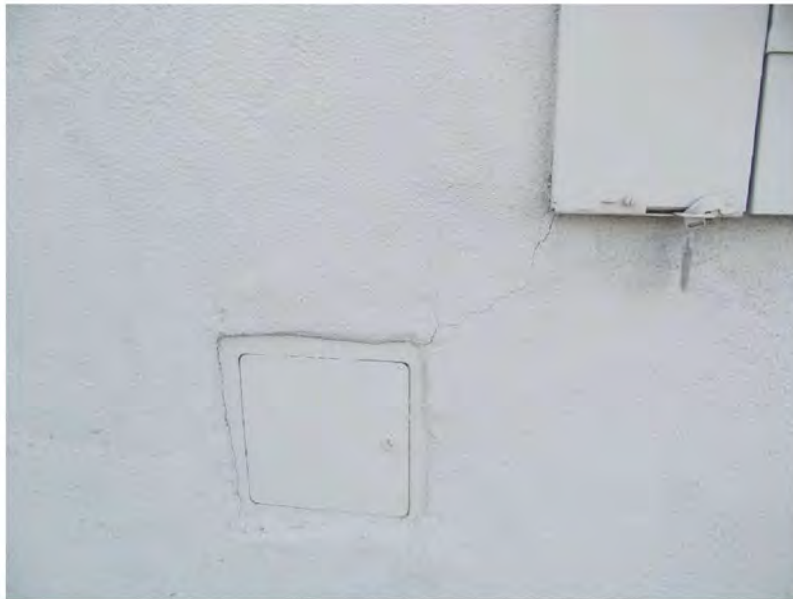
March 10, 2021, Disc OBS5, Photograph 91, SSR, Building B, non-compliant isolation joint at utility box to stucco with diagonal stucco racks.
