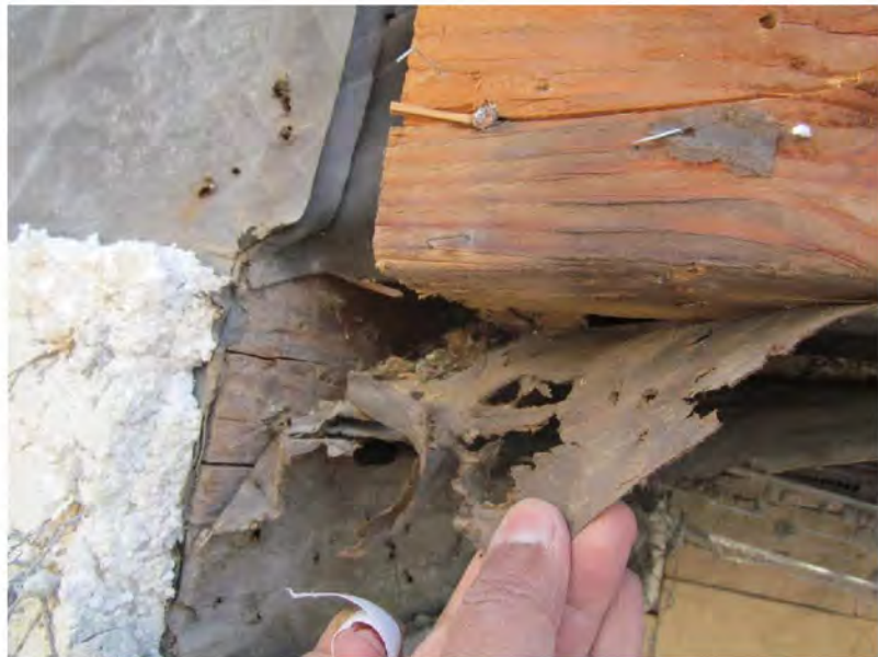
March 10, 2021, Disc IT8, Photograph 120, SSR, Building D, deteriorated WRB over framing with visible stains.
