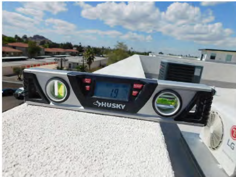
March 11, 2021, Disc OBS7, Photograph 292, PER, Building D, roof parapet wall slopes 1.9-percent inward.
