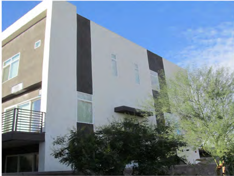
March 11, 2021, Disc OBS 6, Photograph 11, JJF, Building C, missing horizontal movement joints at floorlines.
