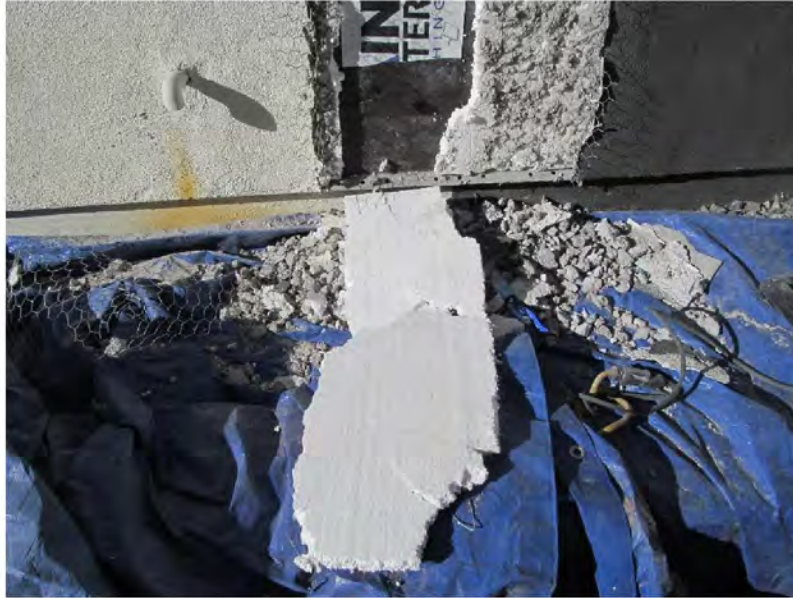
March 10, 2021, Disc IT7, Photograph 279, JJF, Building C, EPS foam board installed over WRB with vertical grooves generally missing at the back face.
