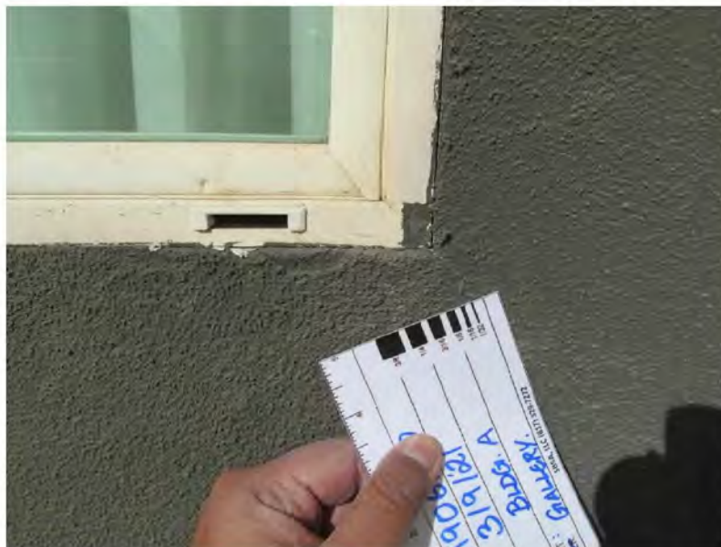
March 9, 2021, Disc IT6, Photograph 81, SSR, Building A, non-compliant isolation joint at window to stucco interface with a diagonal crack at bottom right corner of window.
