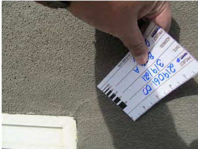
March 9, 2021, Disc IT6, Photograph 39, SSR, Building A, non-compliant isolation joint at sliding door to stucco interface with a diagonal crack at top right corner of sliding door.
