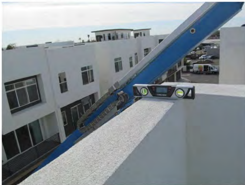
March 11, 2021, Disc IT10, Photograph 136, SSR, Building A, roof parapet wall slopes 0.6-percent outward.
