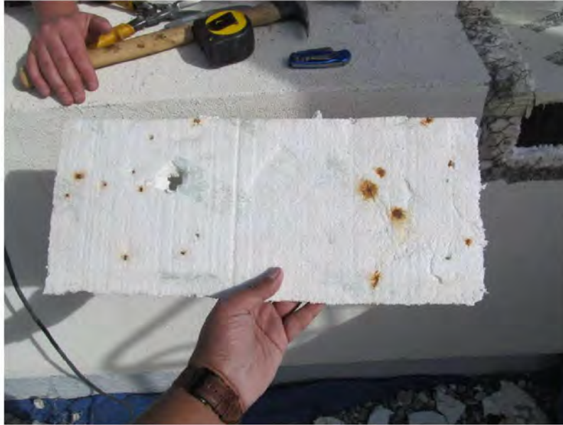
March 11, 2021, Disc IT10, Photograph 103, SSR, Building A, reverse side of EPS foam board shows stains due to corrosion of fasteners.
