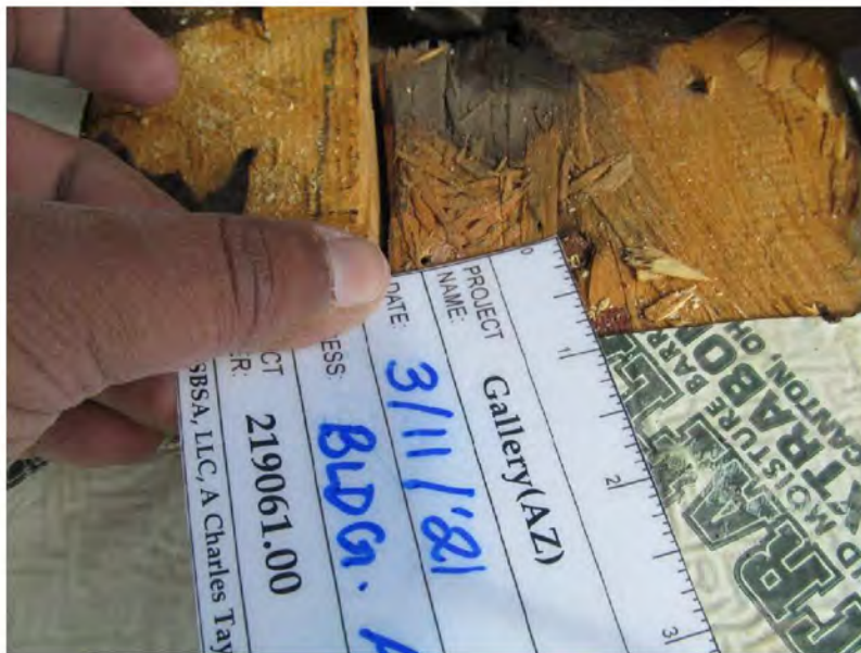
March 11, 2021, Disc IT10, Photograph 125, SSR, Building A, top plate under SAM has stains and rusted fasteners.
