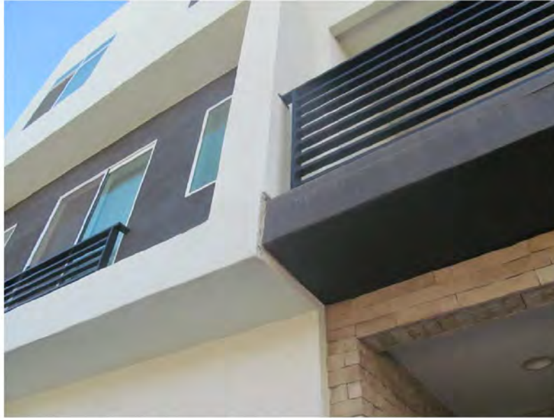
December 19, 2018, Disc OBS1, Photograph 61, JBF, Building C, no weep mechanism at stucco soffits.
