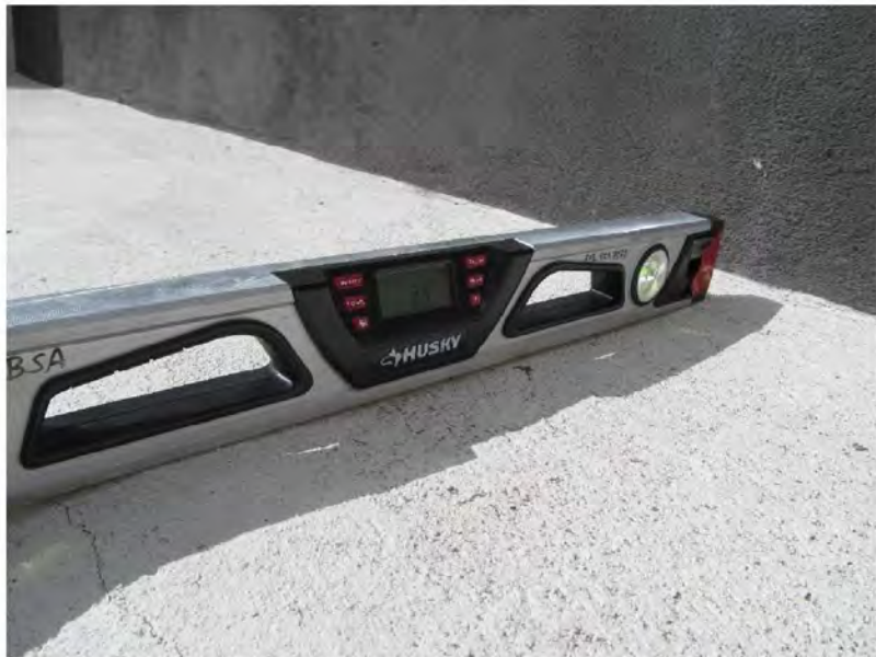
March 9, 2021, Disc IT5, Photograph 313, JJF, Building B, stucco parapet box slopes 3.3-percent outward.
