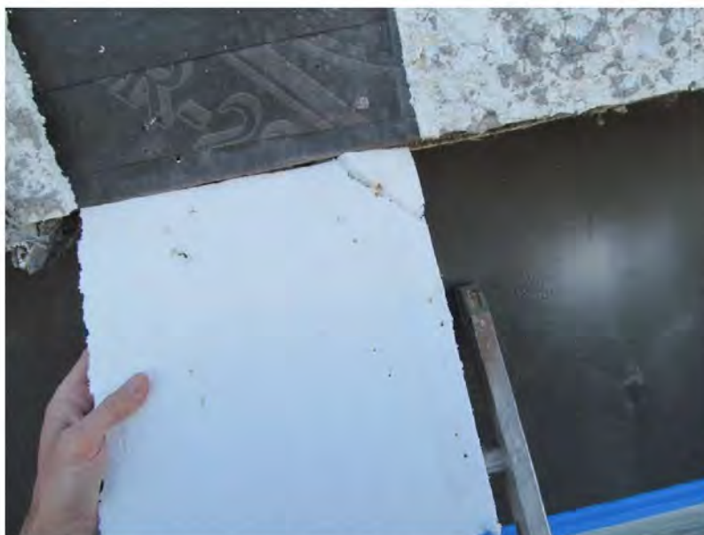
March 10, 2021, Disc IT7, Photograph 226, JJF, Building D, EPS foam board installed over WRB with vertical grooves generally missing at the back face.
