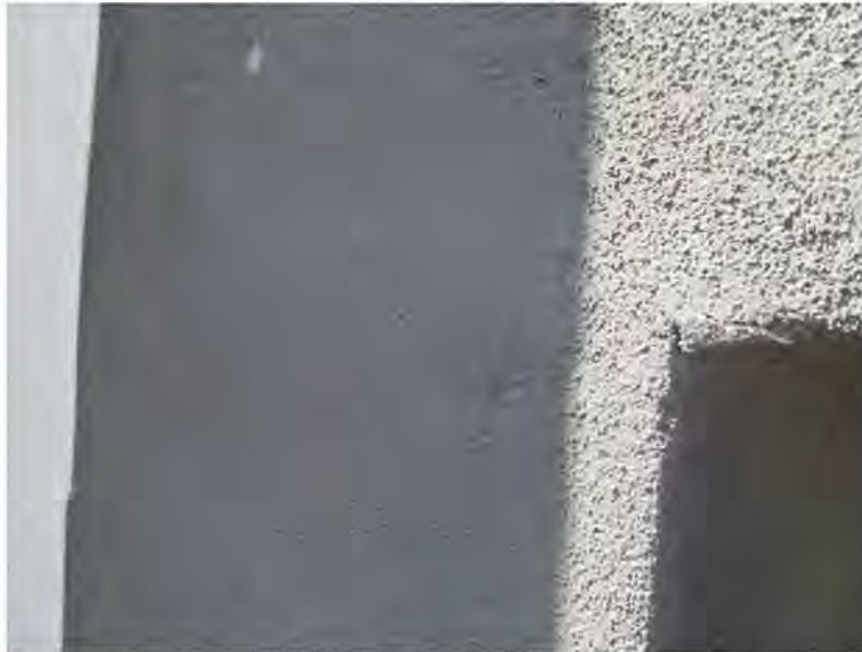
March 10, 2021, Disc IT7, Photograph 97, JFF, Building D, missing control joint and horizontal crack in stucco at floorline.
