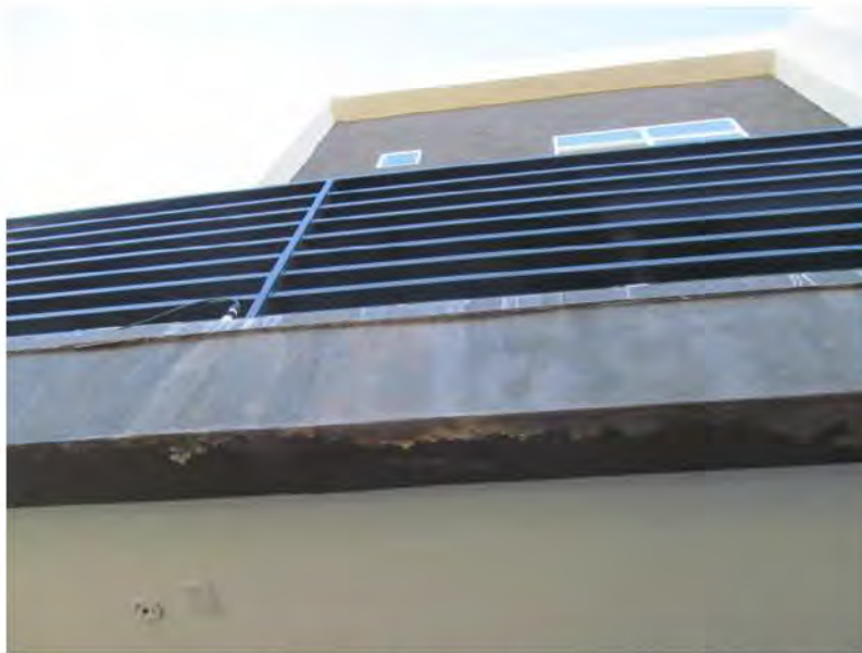
October 14, 2019, Disc OBS3, Photograph 389, SSR, Building D, deck edge flashing inset at stucco and stains visible.
