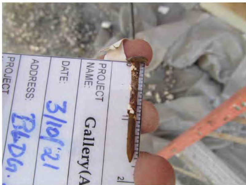
March 10, 2021, Disc IT8, Photograph 172, SSR, Building D, full-depth rusted fasteners.
