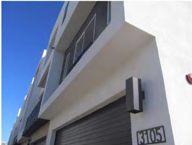
December 19, 2018, Disc OBS1, Photograph 18, JBF, Building D, no weep mechanism at stucco soffit.
