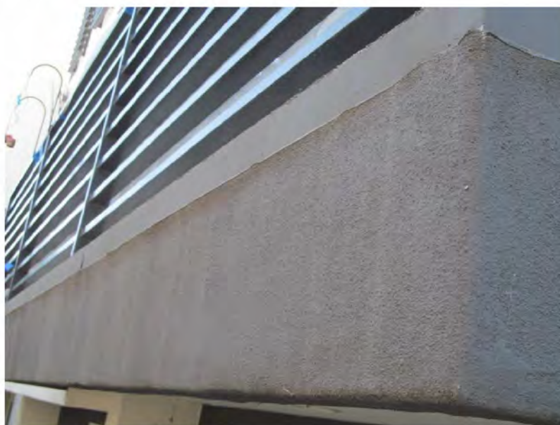
March 10, 2021, Disc IT7, Photograph 182, JFF, Building C, deck edge flashing inset at stucco.
