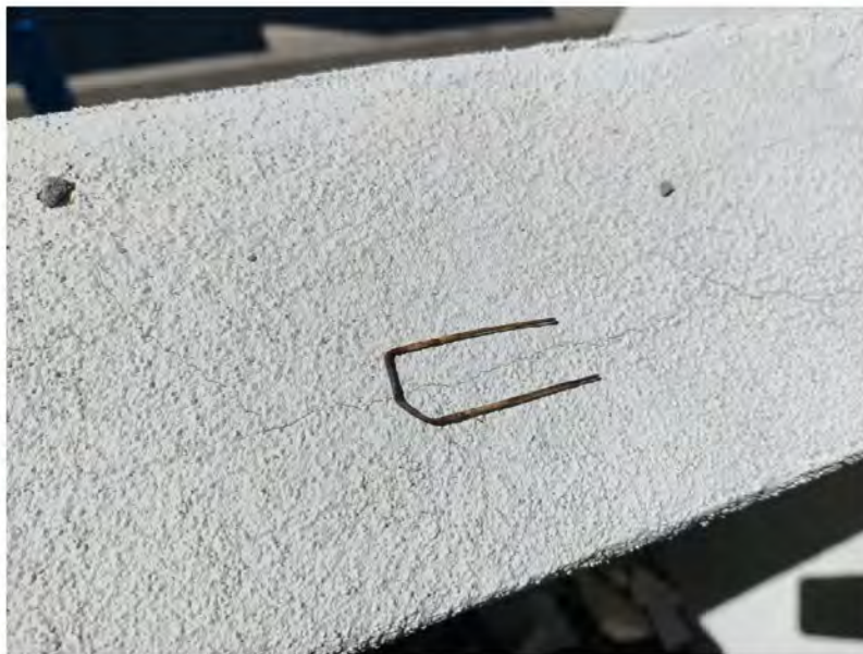
March 11, 2021, Disc IT10, Photograph 374, SSR, Building D, rusted staple.
