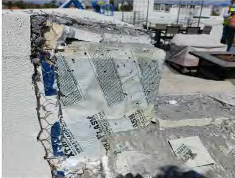
March 11, 2021, Disc IT10, Photograph 378, SSR, Building D, puncture holes in SAM allow moisture intrusion.
