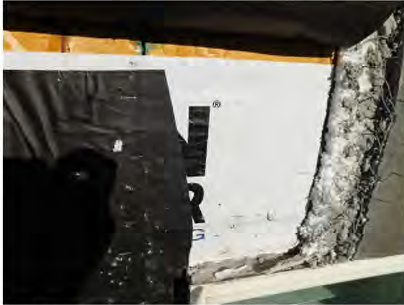
March 10, 2021, Disc IT9, Photograph 269, PER, Building C, missing flashing at window head.
