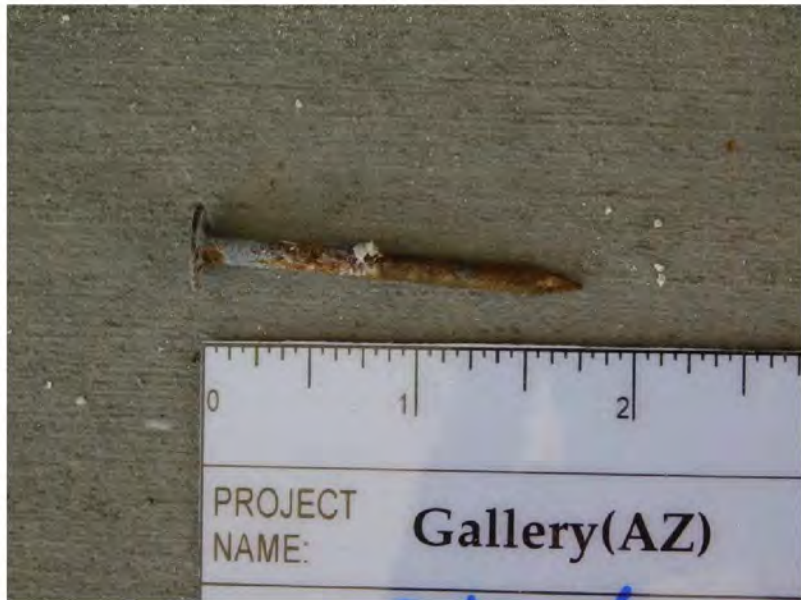
March 10, 2021, Disc IT8, Photograph 93, PER, Building C, deteriorated WRB over framing.
