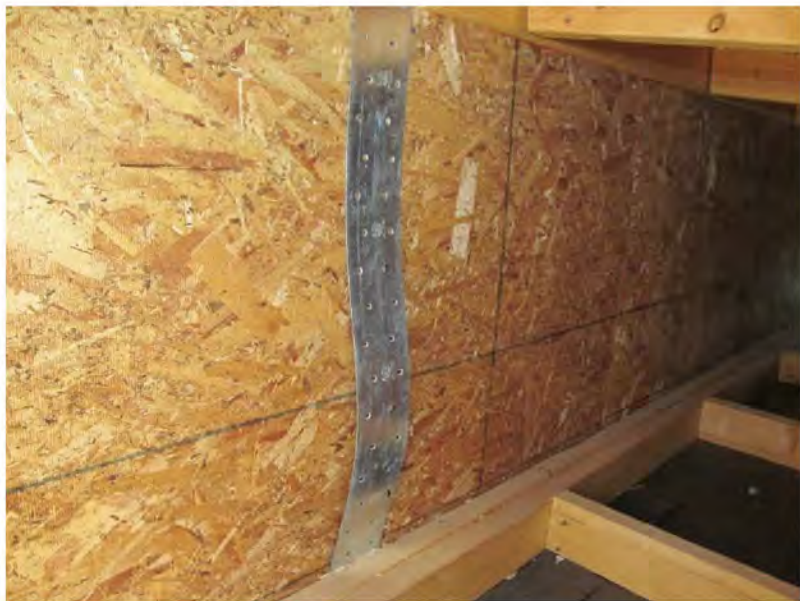
March 10, 2021, Disc IT8, Photograph 278, SSR, Building D - Unit 3111, CS-16 metal strap is disengaged and buckled.
