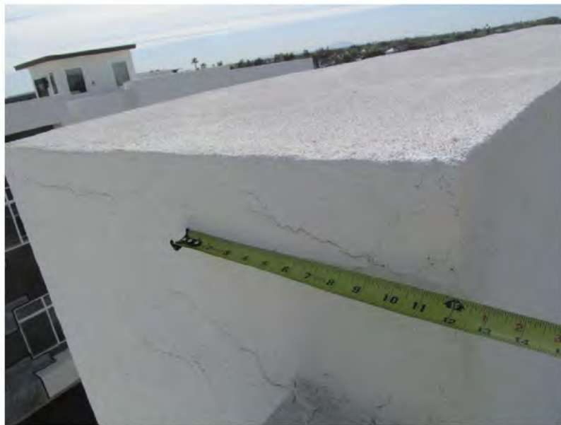
March 11, 2021, Disc IT10, Photograph 172, SSR, Building B, stucco cracks at parapet wall junction.
