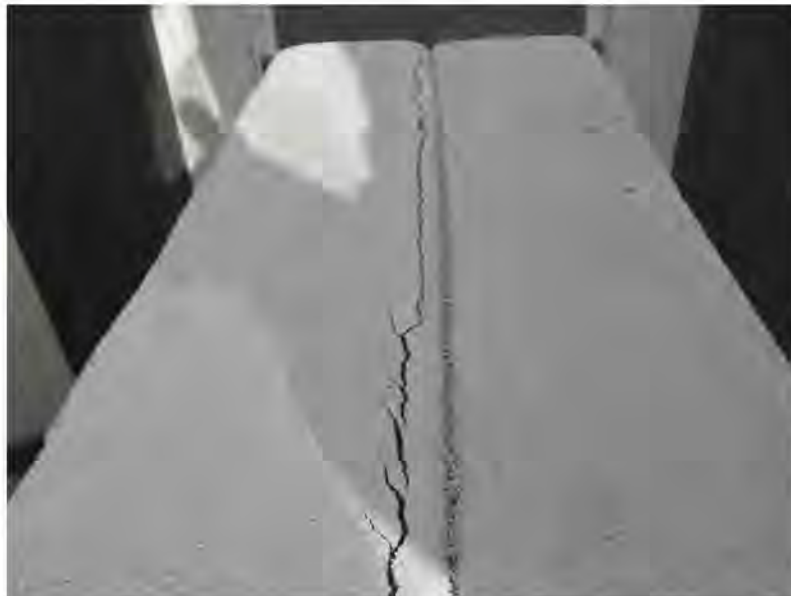
March 11, 2021, Disc OBS6, Photograph 28, JBF, stairs between Buildings C and D, cracking and separation of stair wall. SBSA understands builder performed repairs at this location.
