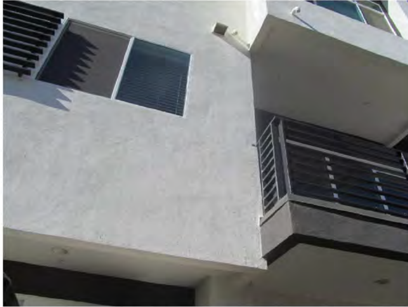
December 19, 2018, Disc OBS1, Photograph 82, JBF, Building B, no weep mechanism at stucco soffits.
