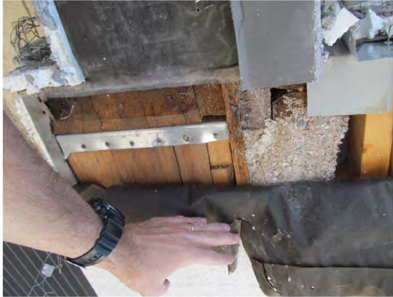
March 9, 2021, Disc IT5, Photograph 72, JJF, Building B, one layer of WRB over framing.
