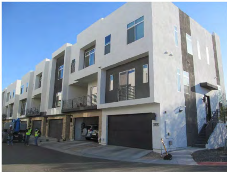
March 10, 2021, Disc IT 8, Photograph 6, SSR, Building D, missing horizontal movement joints at floorlines.
