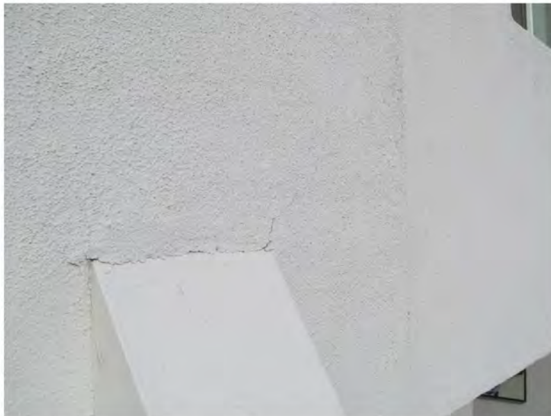
March 9, 2021, Disc IT6, Photograph 27, SSR, Building A, non-compliant isolation joint at penetration to stucco interface with a diagonal crack at top right corner of dryer vent.
