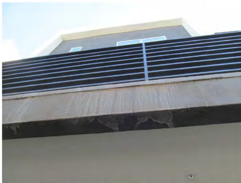
October 14, 2019, Disc OBS2, Photograph 125, SSR, Building B, deck edge flashing inset at stucco and stains visible.
