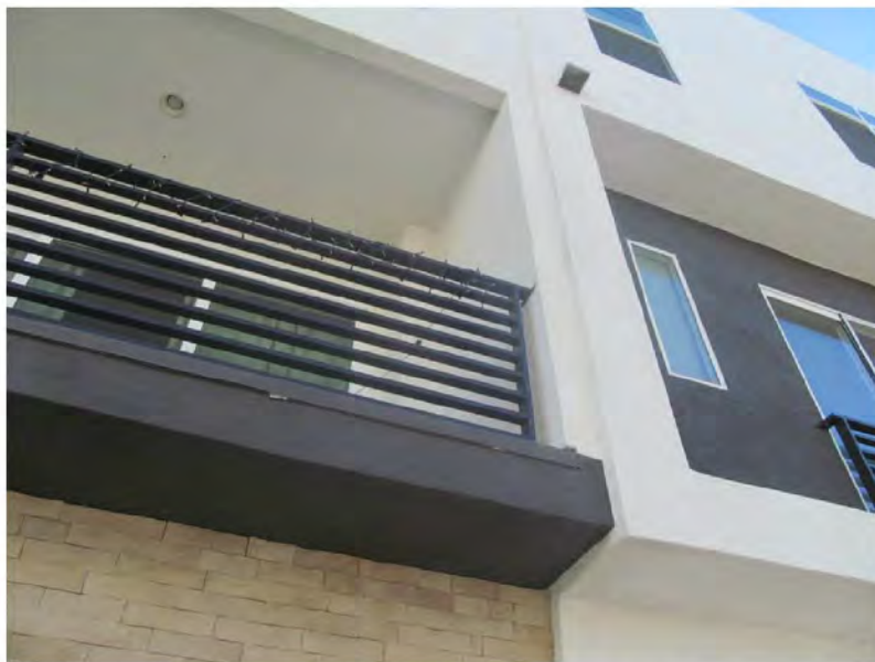
December 19, 2018, Disc OBS1, Photograph 24, JBF, Building D, no weep mechanism at stucco soffits.
