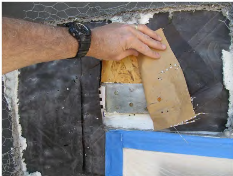
March 10, 2021, Disc IT7, Photograph 139, JJF, Building D, missing flashing at sliding door head.
