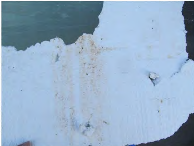
March 10, 2021, Disc IT7, Photograph 210, JJF, Building C, EPS foam board installed tight to WRB and vertical grooves generally missing at the back face.
