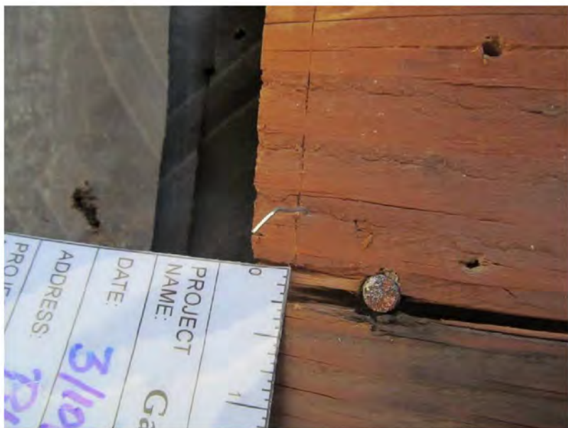
March 10, 2021, Disc IT8, Photograph 96, SSR, Building D, rusted fastener head at framing.
