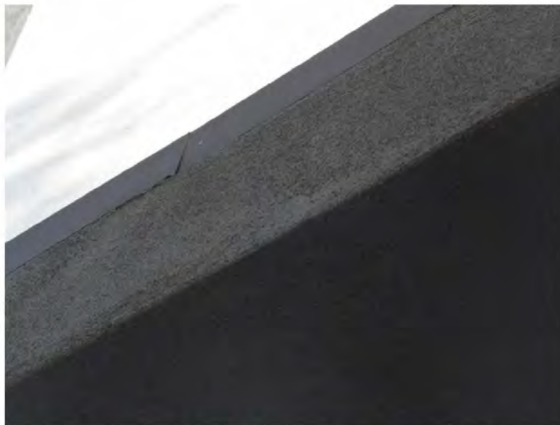
March 10, 2021, Disc OBS5, Photograph 23, SSR, Building. A, awning edge flashing inset at stucco.
