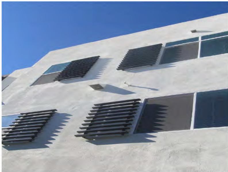
December 18, 2019, Disc OBS 1, Photograph 71, JJF, Building C, missing horizontal movement joints at floorline.
