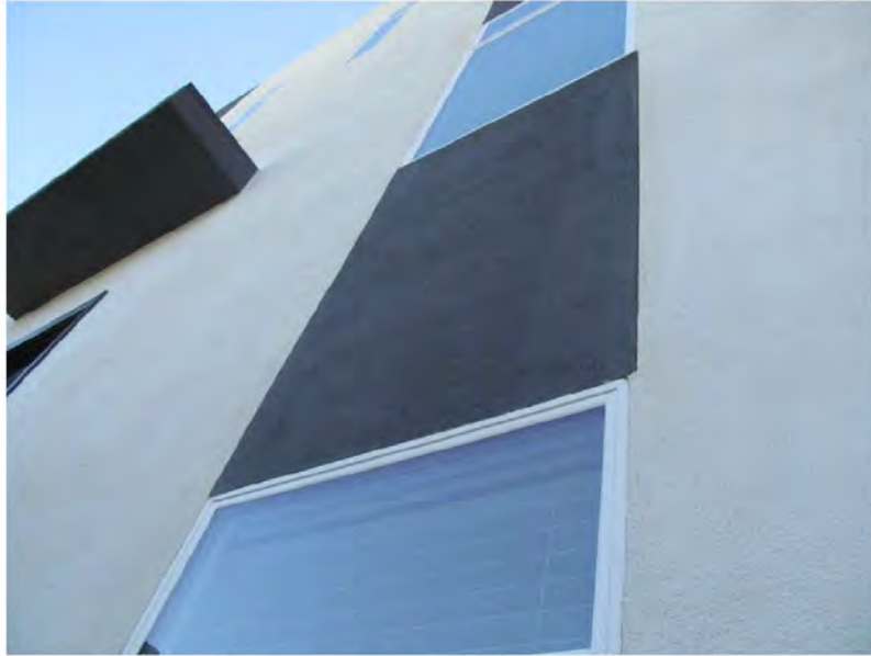
December 19, 2018, Disc OBS1, Photograph 129, JBF, Building A, no weep mechanism at window head.
