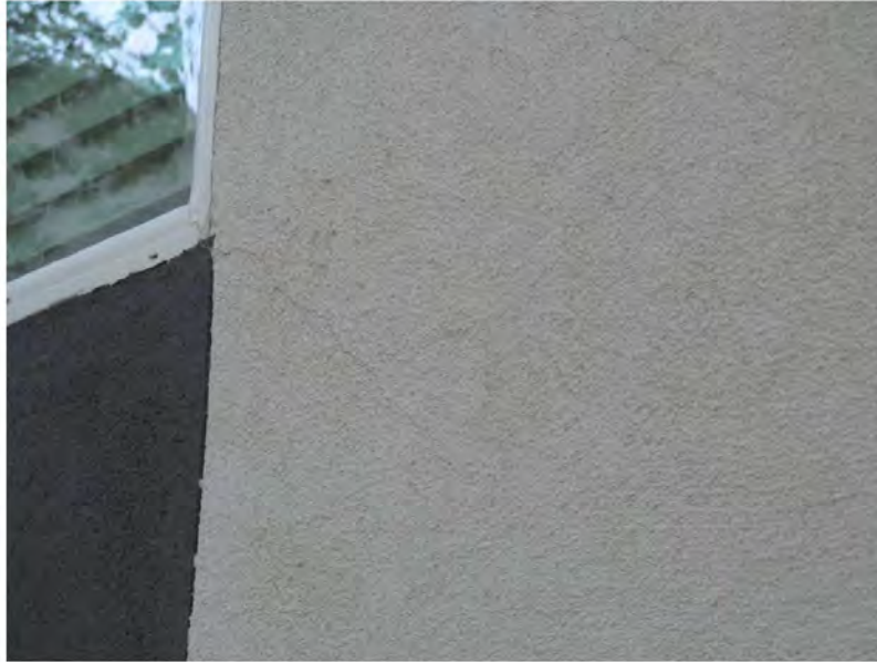
March 10, 2021, Disc OBS 5, Photograph 29, SSR, Building A, horizontal stucco crack.
