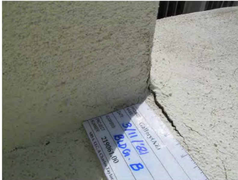
March 11, 2021, Disc IT10, Photograph 241, SSR, Building B, stucco cracks at parapet wall junction.
