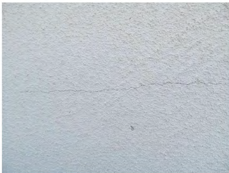
March 11, 2021, Disc OBS 6, Photograph 75, JJF, Building C, stucco cracks.
