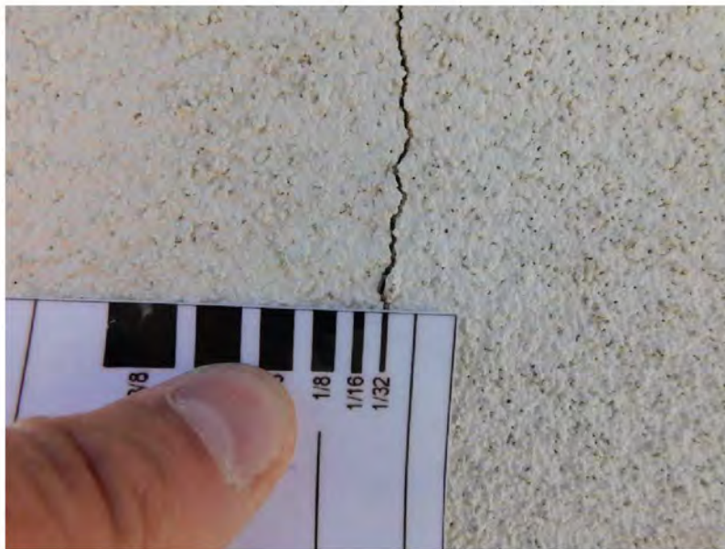
March 11, 2021, Disc OBS7, Photograph 421, PER, Building C, roof parapet wall cracks.
