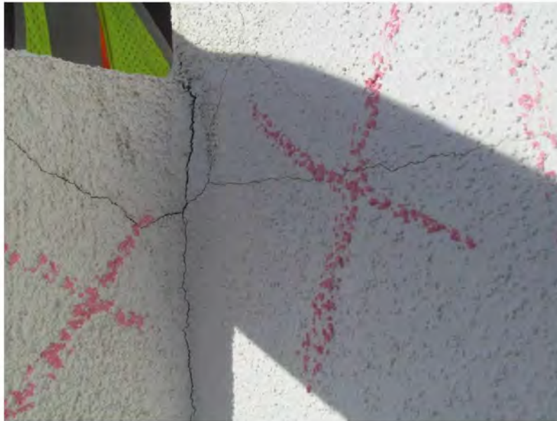
March 11, 2021, Disc IT10, Photograph 19, SSR, Building A, stucco cracks at parapet wall junction.
