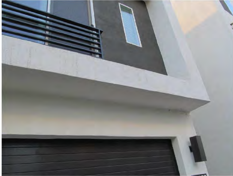
March 10, 2021, Disc OBS5, Photograph 72, SSR, Building B, missing isolation joint at stucco siding to stucco soffit
