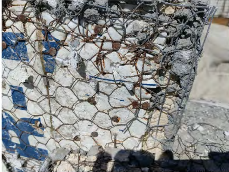
March 11, 2021, Disc IT10, Photograph 372, SSR, Building D, rusted nails and lath indicate moisture intrusion through stucco.
