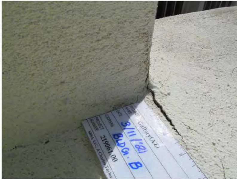
March 11, 2021, Disc IT10, Photograph 241, SSR, Building B, roof parapet wall stucco cracks.
