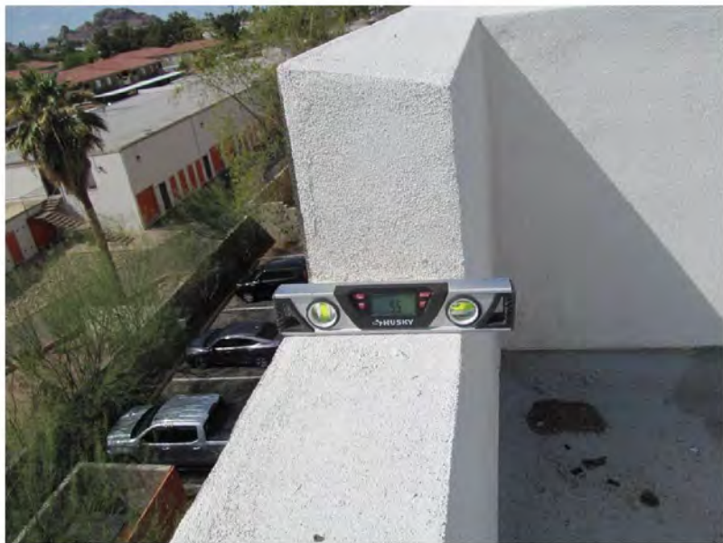
March 11, 2021, Disc IT10, Photograph 313, SSR, Building B, roof parapet wall slopes 5.5-percent inward.
