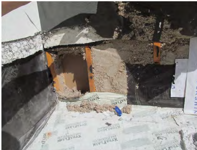
March 10, 2021, Disc IT8, Photograph 237, SSR, Building D - Unit 3111, missing OSB sheathing at existing stud framing.
