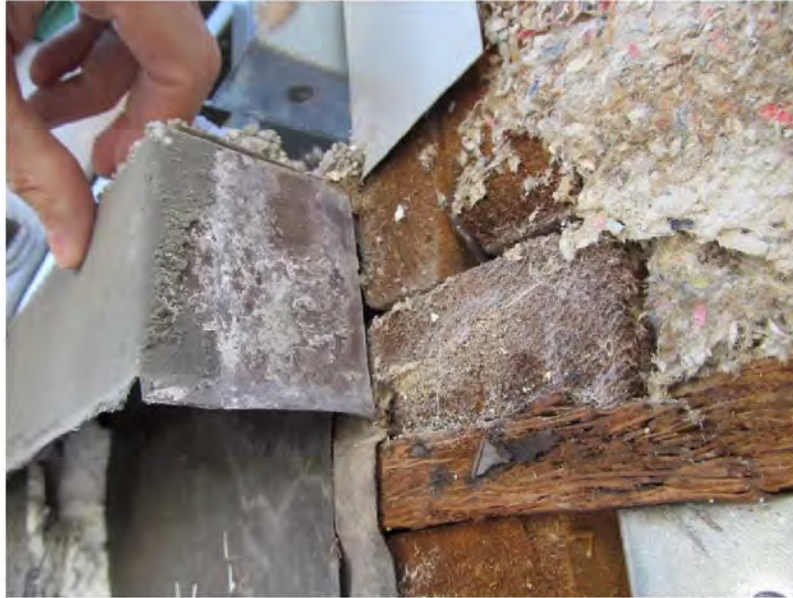
March 9, 2021, Disc IT5, Photograph 73, JJF, Building B, visible stains at sheathing edge and deterioration.
