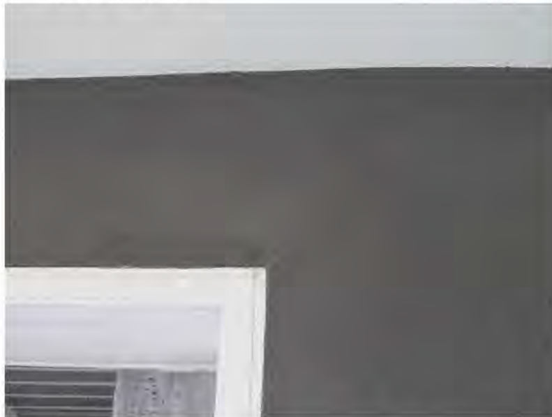
March 9, 2021, Disc IT5, Photograph 3, JJF, Building A, missing flashing at sliding door head.
