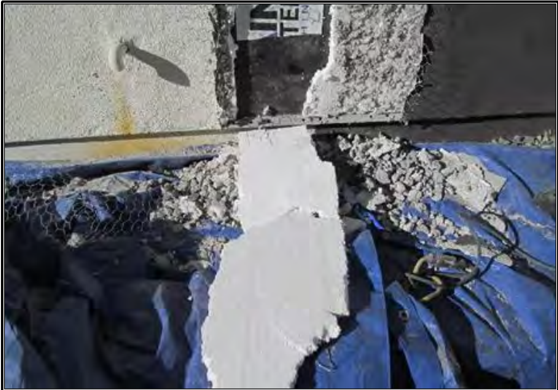
Photo #4 (Pltff Photo Disc IT7 Photo 279): EPS foam board exposed during DT.
