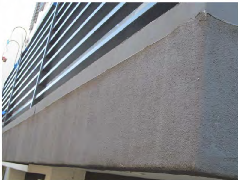
March 10, 2021, Disc IT7, Photograph 182, JJF, Building C, deck edge flashing inset at stucco.
