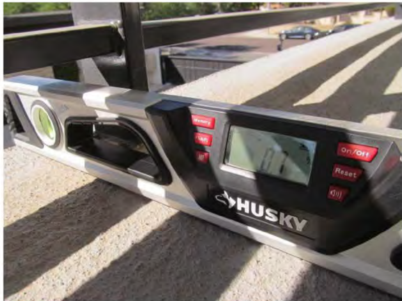
October 15, 2019, Disc OBS3, Photograph 277, SSR, Building C - Unit 3125, 0.7-percent slope at the deck edge and stains of water ponding at the edge.
