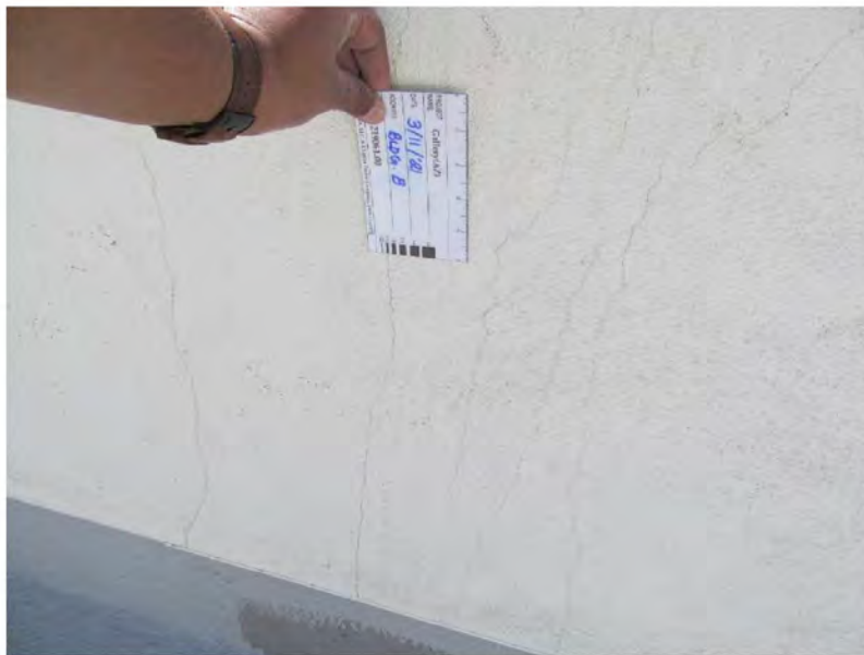
March 11, 2021, Disc IT10, Photograph 207, SSR, Building B, roof parapet wall stucco cracks.
