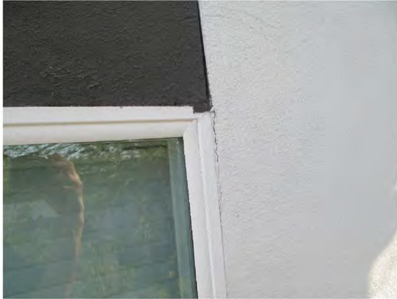
March 10, 2021, Disc IT7, Photograph 7, JJF, Building D, non-compliant isolation joint at window to stucco interface and resulting separation at window.
