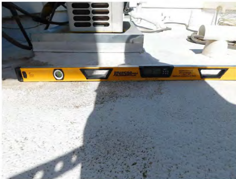
March 11, 2021, Disc OBS7, Photograph 365, PER, Building C, no crickets at upslope locations of rooftop equipment. Note stains indicate ponding water.
