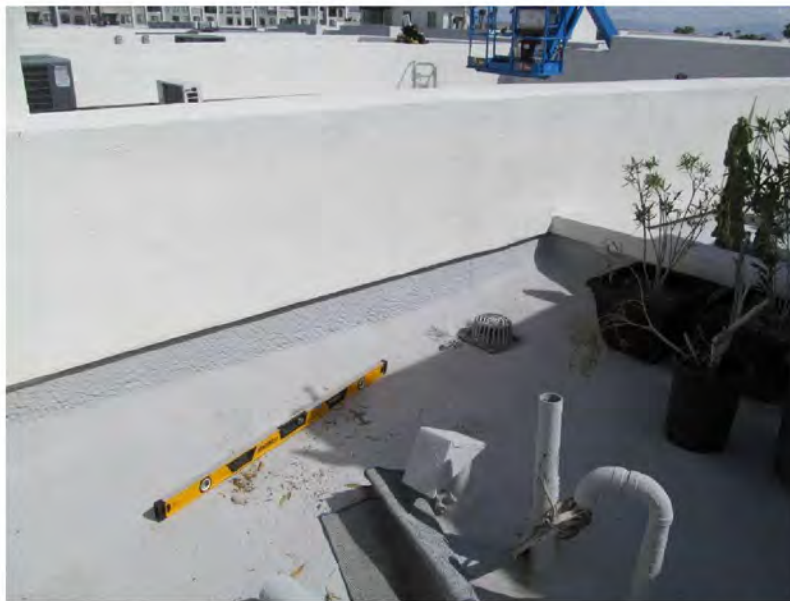
March 11, 2021, Disc IT10, Photograph 264, SSR, Building B, 0-inch-per-foot slope at cricket towards point of drainage.
