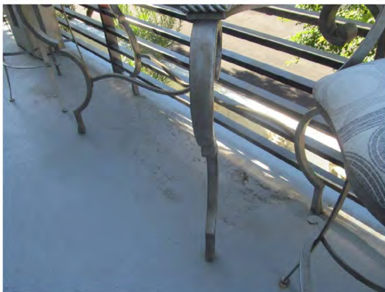
December 19, 2018, Disc OBS1, Photograph 167, JBF, Building A - Unit 3124, stains indicate ponding water at the deck edge.
