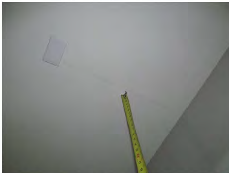
March 10, 2021, Disc IT8, Photograph 302, SSR, Building B - Unit 3110, stains at ceiling under the roof.
