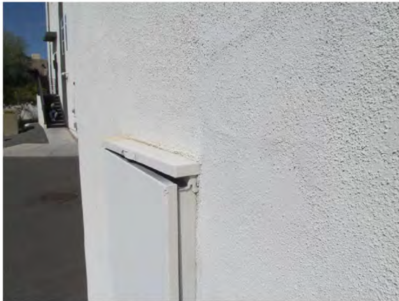
March 10, 2021, Disc OBS6, Photograph 176, JJF, Building C, non-compliant isolation joint at utility box to stucco interface.
