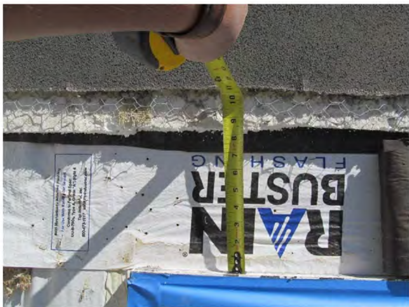
March 10, 2021, Disc IT8, Photograph 219, SSR, Building D, missing flashing at window head.
