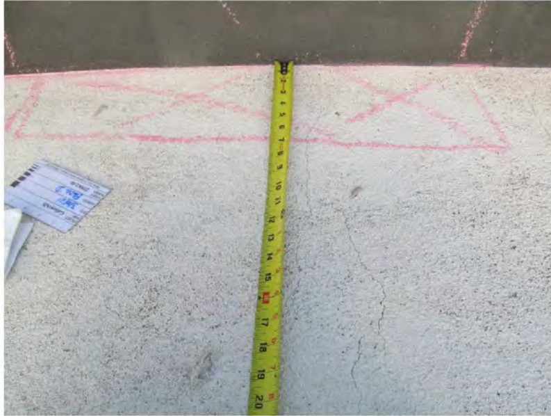
March 10, 2021, Disc IT8, Photograph 54, SSR, Building D, pop-out box stucco cracks.
