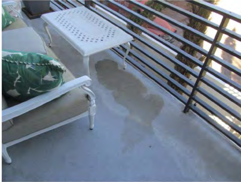
October 15, 2019, Disc OBS3, Photograph 401, SSR, Building D - Unit 3105, stains of water ponding at the edge.
