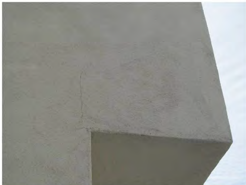
March 11, 2021, Disc OBS 6, Photograph 209, JJF, Building C, stucco cracks.
