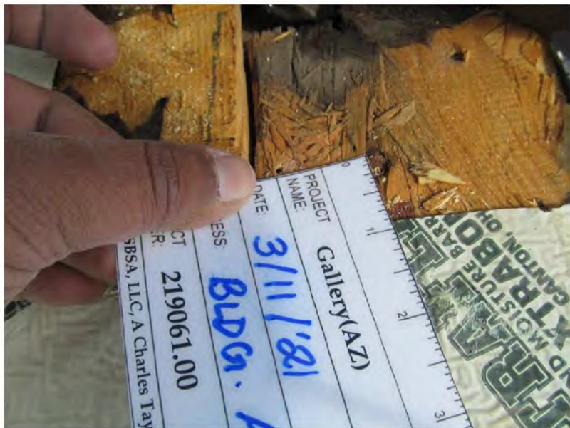
March 11, 2021, Disc IT10, Photograph 125, SSR, Building A, top plate under SAM has stains and rusted fasteners.
