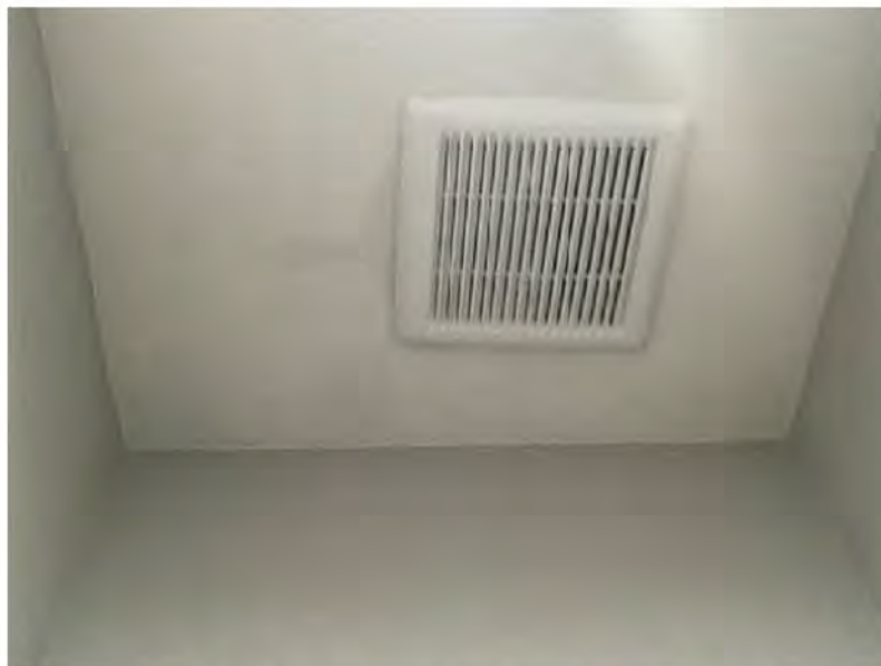
Homeowner-disclosed photo, disclosed on June 18, 2021, Building B - Unit 3110, Bates Number GALLERY-LINE 3110-000004, water stains at vent due to previous roof leak event.
