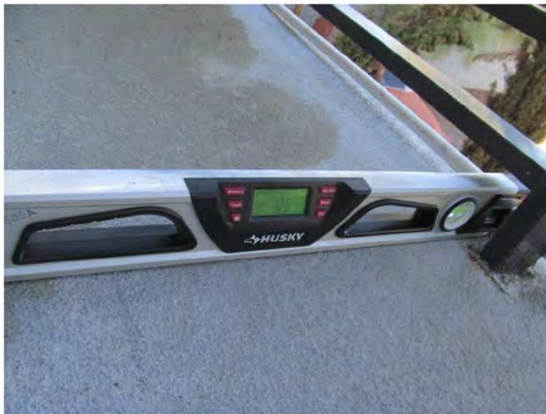
October 15, 2019, Disc OBS3, Photograph 414, SSR, Building D - Unit 3105, 0.3-percent slope at the deck edge and stains of water ponding at the edge.
