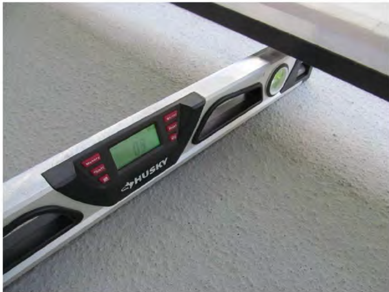
October 14, 2019, Disc OBS2, Photograph 462, SSR, Building A - Unit 3122, 0.9-percent slope at the deck edge.
