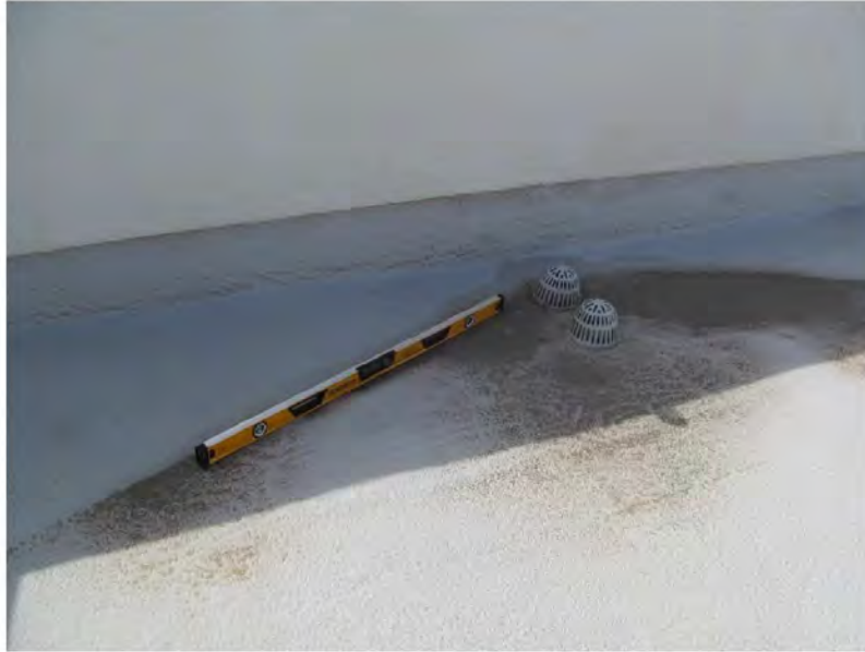
March 11, 2021, Disc IT10, Photograph 157, SSR, Building A, 0-inch-per-foot slope at cricket towards point of drainage. Note stains indicate ponding water.
