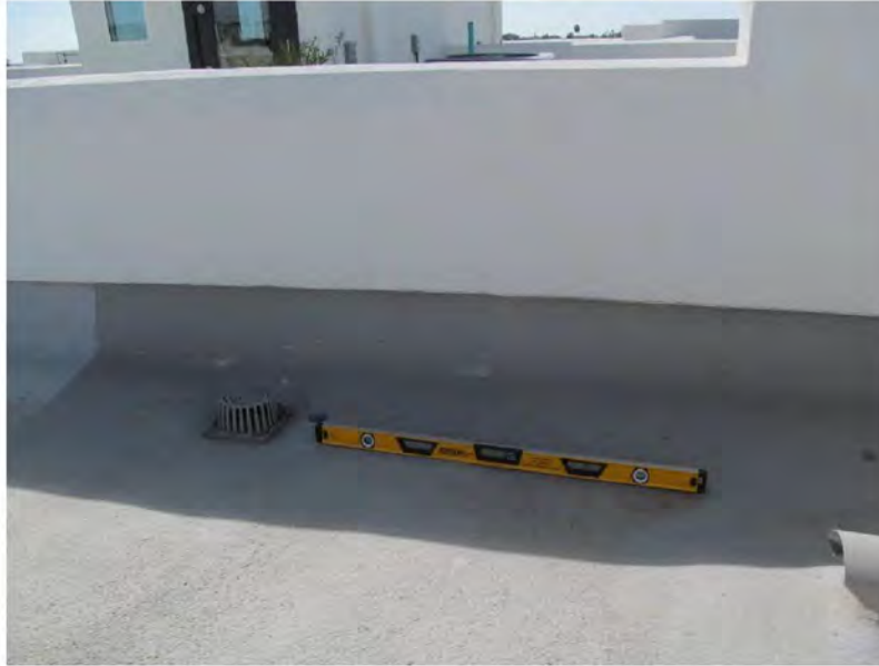
March 11, 2021, Disc IT10, Photograph 236, SSR, Building B, 0-inch-per-foot slope towards point of drainage. Note stains indicate ponding water.
