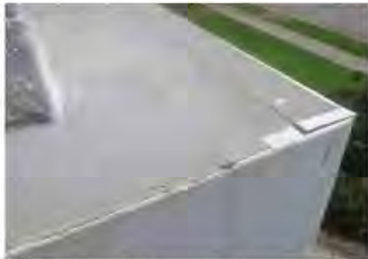
Figure 7. Component thickness prevents free drainage.
