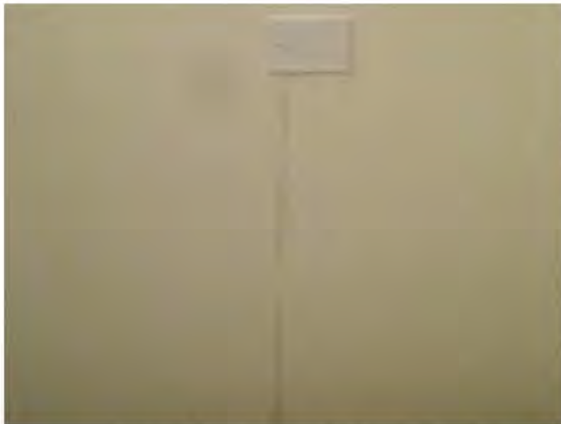
Homeowner-disclosed photo, disclosed on June 18, 2021, Building B - Unit 3110, Bates Number GALLERY-LINE 3110-000002, water stains at ceiling due to previous roof leak event.
