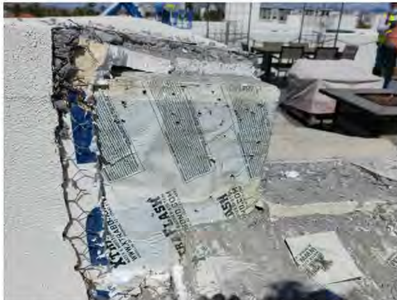
March 11, 2021, Disc IT10, Photograph 378, SSR, Building D, puncture holes in SAM allow moisture intrusion.
