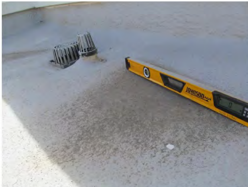
March 11, 2021, Disc IT10, Photograph 287, SSR, Building B, 0-inch-per-foot slope at cricket towards point of drainage. Note stains indicate ponding water.
