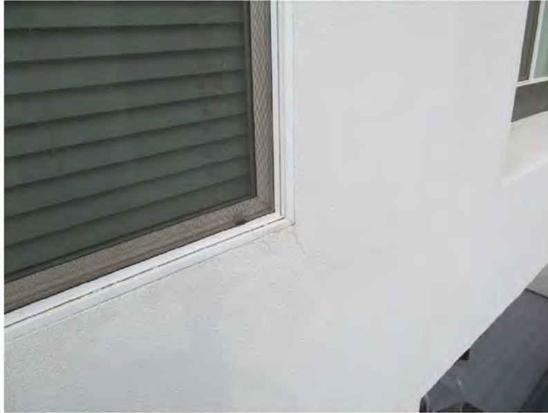
March 9, 2021, Disc IT6, Photograph 14, SSR, Building A, non-compliant isolation joint at window to stucco interface with a diagonal crack at bottom right corner of window.
