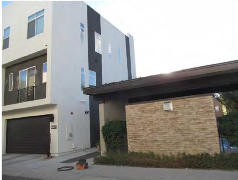
March 10, 2021, Disc OBS 5, Photograph 2, SSR, Building A, missing horizontal movement joints at floorlines.
