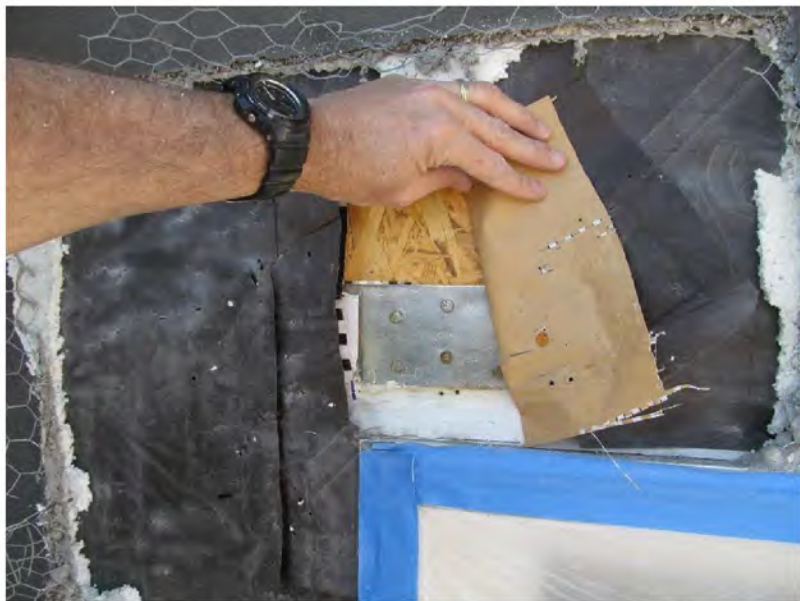
March 10, 2021, Disc IT7, Photograph 139, JJF, Building D, missing flashing at sliding door head.
