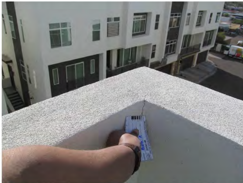
March 11, 2021, Disc IT10, Photograph 37, SSR, Building A, stucco cracks at parapet wall junction.
