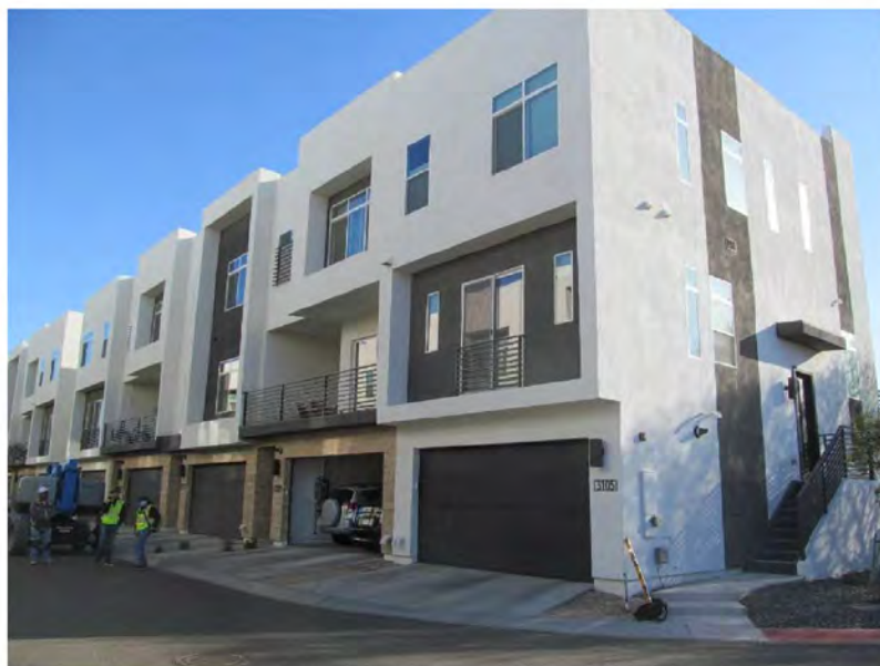
March 10, 2021, Disc IT 8, Photograph 6, SSR, Building D, missing horizontal movement joints at floorlines.
