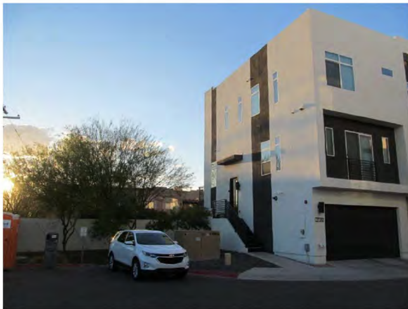
March 10, 2021, Disc OBS 5, Photograph 63, SSR, Building B, missing horizontal movement joints at floorlines.
