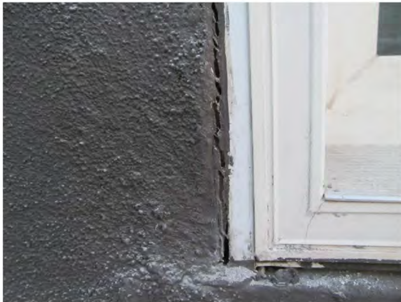
March 10, 2021, Disc IT7, Photograph 149, JJF, Building D, failed sealant joint at door to stucco interface; no backer rod visible.
