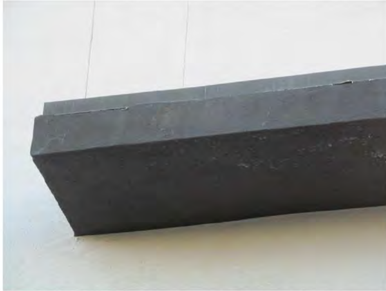
March 10, 2021, Disc OBS5, Photograph 94, SSR, Building B, awning edge flashing inset at stucco.
