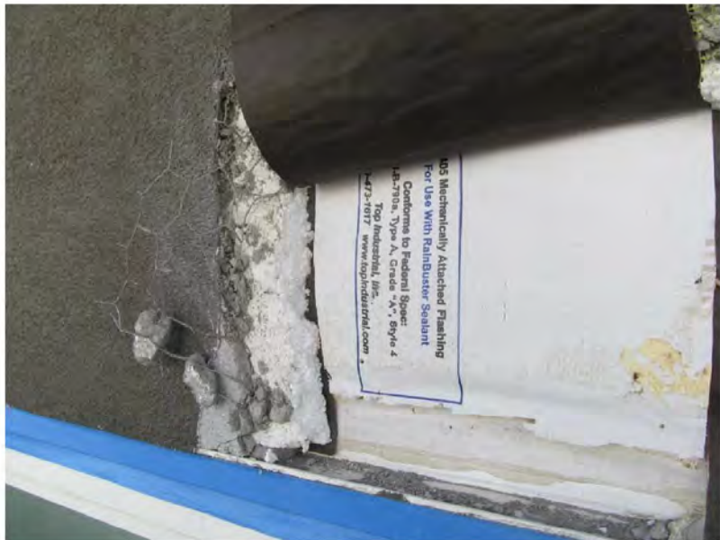
March 9, 2021, Disc IT6, Photograph 286, SSR, Building A, missing flashing at sliding door head.
