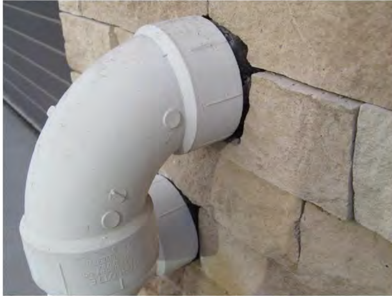
March 11, 2021, Disc OBS6, Photograph 41, JJF, Building C, non-compliant isolation joint at pipe to AMV interface.
