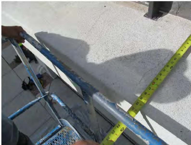
March 9, 2021, Disc IT6, Photograph 56, SSR, Building A, pop-out box stucco cracks.
