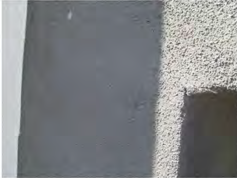
March 10, 2021, Disc IT7, Photograph 97, JF, Building D, missing control joint and horizontal crack in stucco at floorline.
