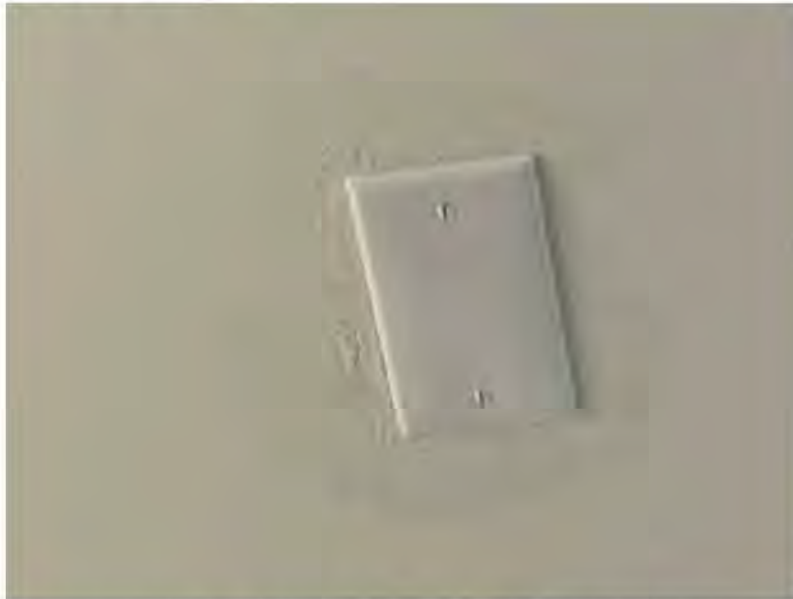
Homeowner-disclosed photo, disclosed on June 18, 2021, Building B - Unit 3112, Bates Number GALLERY-CHANG 3112-000006, water stains at ceiling due to previous roof leak event.
