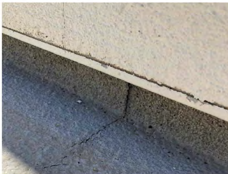
Nautilus-disclosed photo, disclosed on June 16, 2021, Building B - Unit 3110, Photo Number 6, tear and split of roof surface adjacent to drains.
