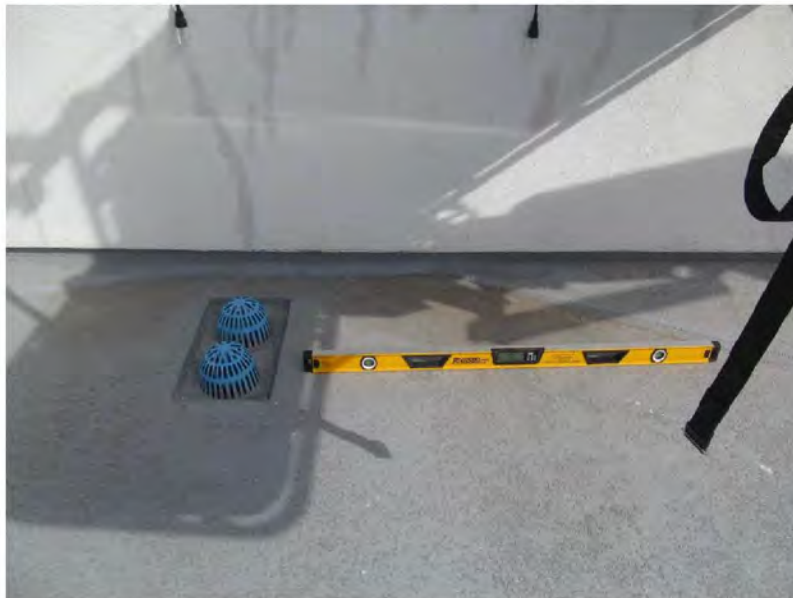
March 11, 2021, Disc IT10, Photograph 99, SSR, Building A, 0-inch-per-foot slope at cricket towards point of drainage. Note stains indicate ponding water.
