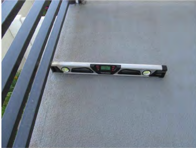
October 15, 2019, Disc OBS3, Photograph 175, SSR, Building B - Unit 3106, 0.4-percent slope at the deck edge and stains of water ponding at the edge.
