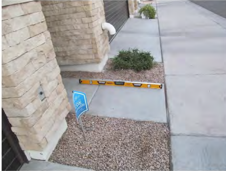
March 10, 2021, Disc OBS5, Photograph 108, SSR, Building B, east side, longitudinal slope of sidewalk is 11.5-percent, exceeding maximum allowable of 8.33-percent for a ramp.
