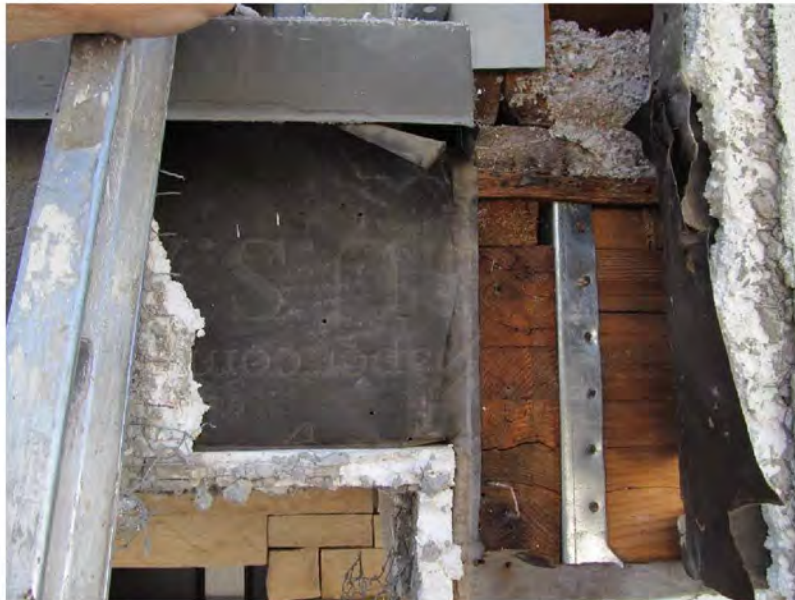
March 9, 2021, Disc IT5, Photograph 75, JJF, Building B, damaged framing due to water intrusion.
