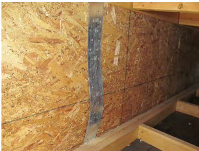
March 10, 2021, Disc IT8, Photograph 278, SSR, Building D - Unit 3111, CS-16 metal strap is disengaged and buckled.
