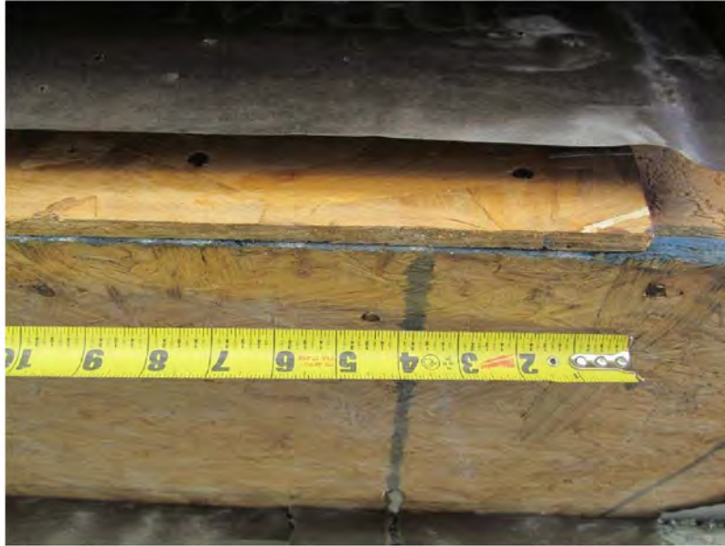
March 9, 2021, Disc IT6, Photograph 266, SSR, Building A, sheathing bottom edge stained at wall-soffit junction.
