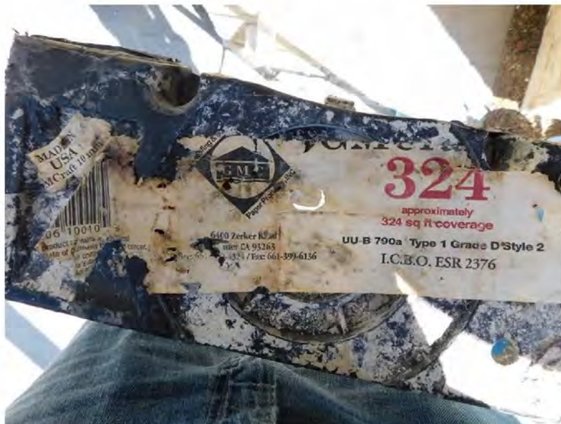
March 10, 2021, Disc IT9, Photograph 124, SSR, Building C, manufacturer's label shows the building paper is Type 1, Grade D, Style 2 building paper with 10-minute water resistance and references ESR 2376.
