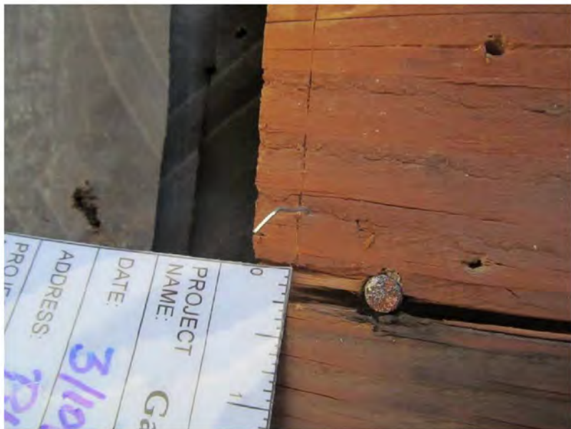
March 10, 2021, Disc IT8, Photograph 96, SSR, Building D, rusted fastener head at framing.
