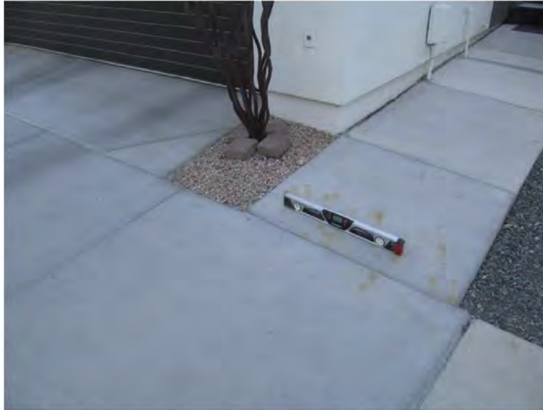
March 10, 2021, Disc OBS5, Photograph 44, SSR, Building A, east side, cross-slope of sidewalk is 4.1-percent, exceeding maximum allowable of 1.5-percent per MAG Detail 230.
