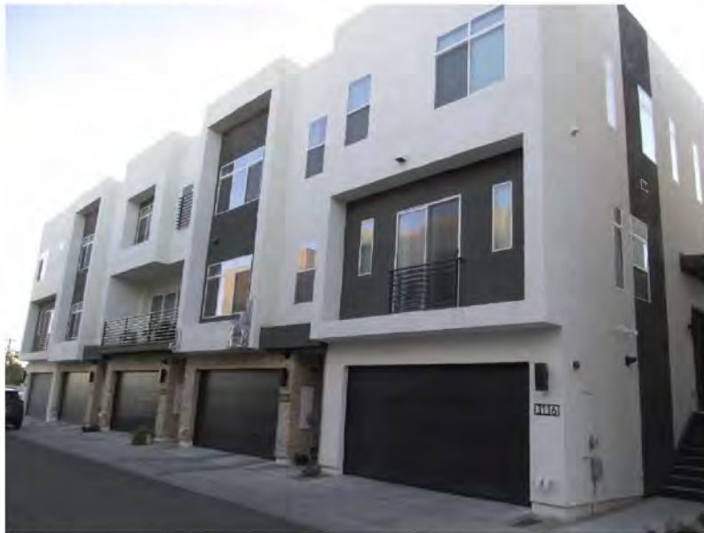
March 10, 2021, Disc OBS5, Photograph 61, SSR, Building B, east side, roof drains discharge into undrained landscaped islands next to foundation at multiple locations.
