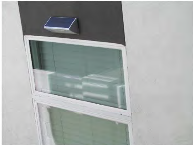
March 11, 2021, Disc OBS6, Photograph 222, JJF, Building D, no weep mechanism at window heads.
