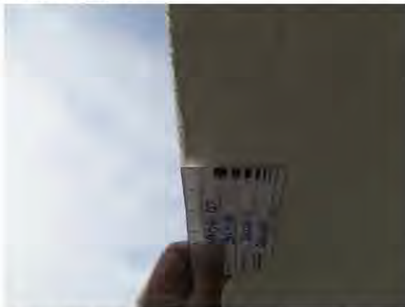
March 9, 2021, Disc IT6, Photograph 32, SSR, Building A, no weep mechanism at soffit and stucco crack along the edge.
