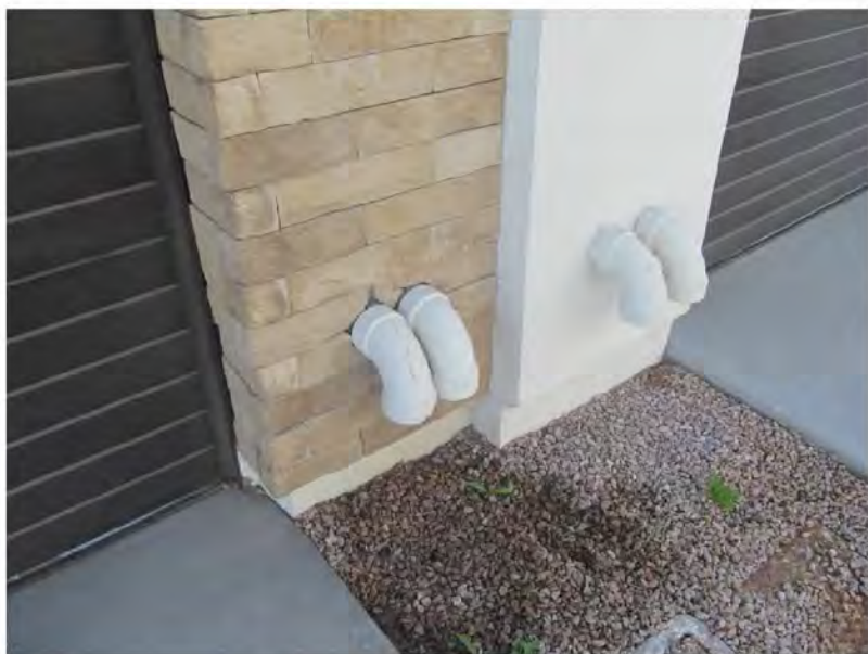
December 19, 2018, Disc OBS1, Photograph 52, JBF, Building C, condensate from high efficiency units drain water adjacent to foundation bound by concrete flatwork into the electrical vault.
