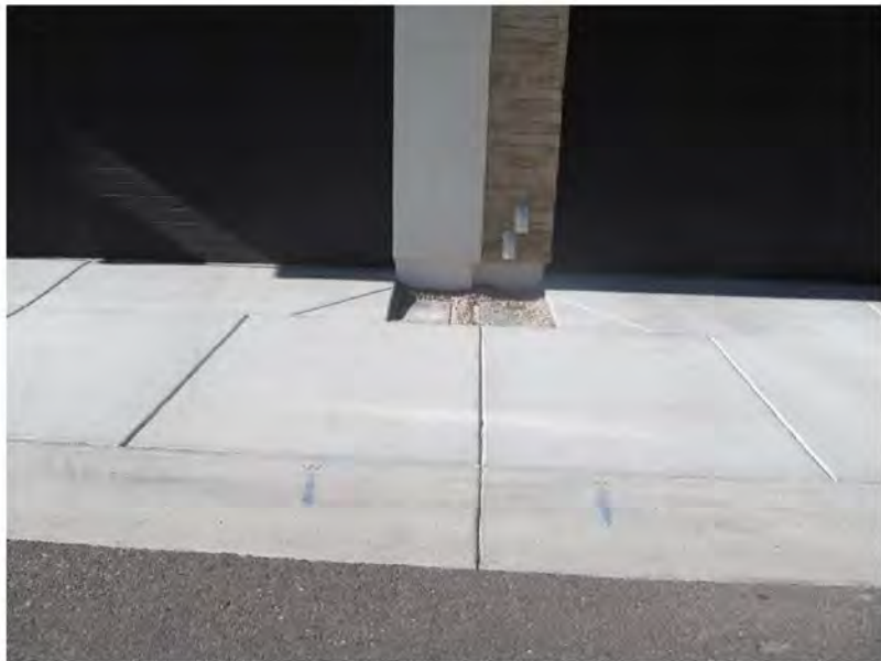
December 19, 2018, Disc OBS1, Photograph 157, JBF, east elevation of Building A, undrained landscaped islands next to foundation are bounded by concrete flatwork. Roof drains discharge into this area also and flow into the electrical vault.
