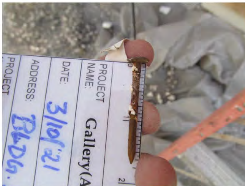
March 10, 2021, Disc IT8, Photograph 172, SSR, Building D, full-depth rusted fasteners.
