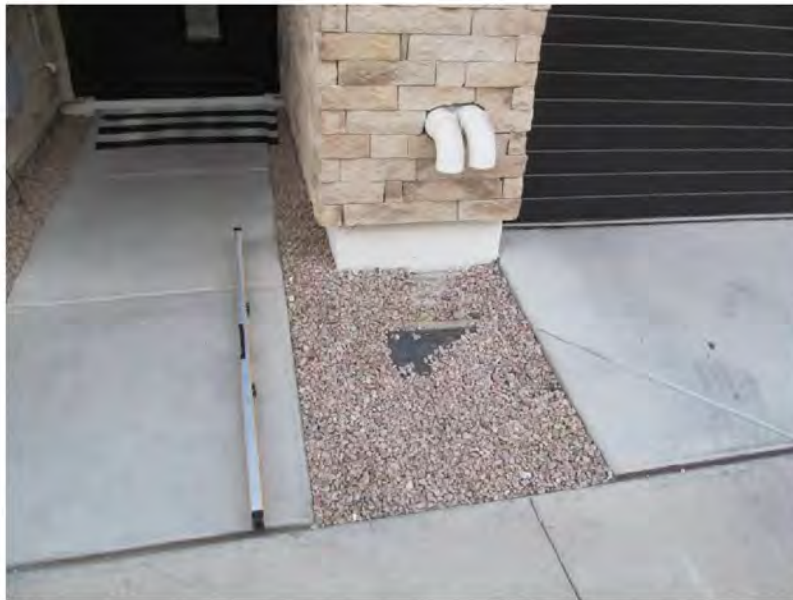
March 10, 2021, Disc OBS5, Photograph 107, SSR, Building B, east side, main and overflow roof drains discharge into undrained landscaped islands next to foundation between entrance to unit and driveway.
