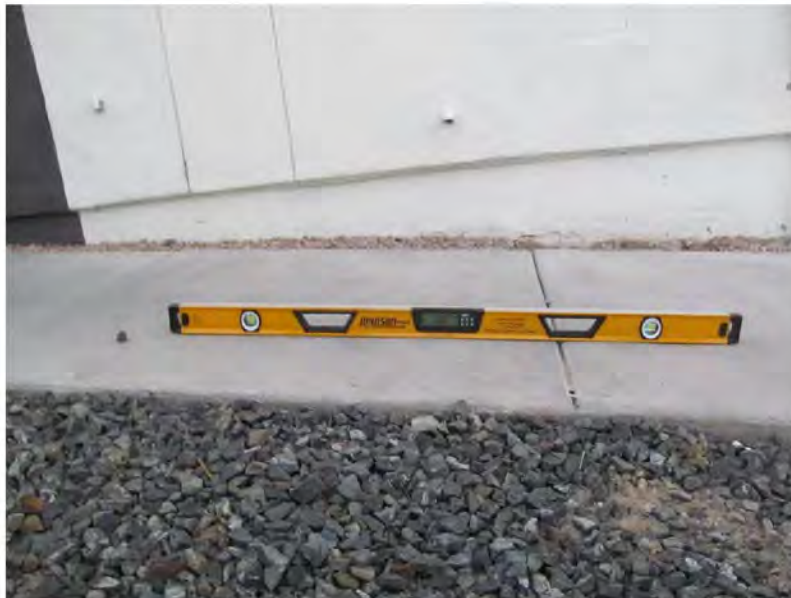
March 10, 2021, Disc OBS5, Photograph 112, SSR, Building B, south side, longitudinal slope of sidewalk is 10.0-percent, exceeding maximum allowable of 8.33-percent for a ramp.
