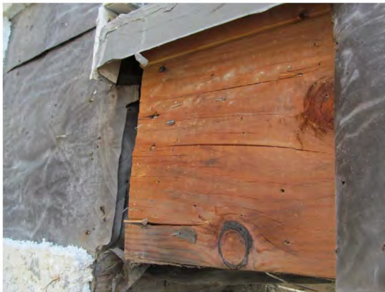
March 10, 2021, Disc IT8, Photograph 114, SSR, Building D, one layer of WRB over framing with visible stains.
