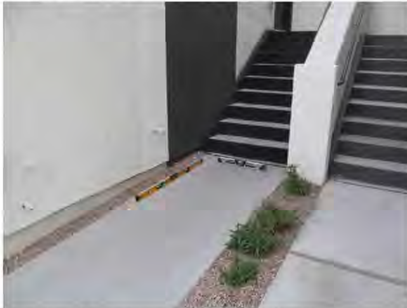
March 10, 2021 Disc OBS5, Photograph 97, SSR, Building B, north side, no landing constructed at bottom of stairs. Longitudinal slope of sidewalk is 4.7-percent.
