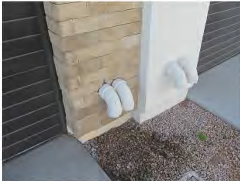
December 19, 2018, Disc OBS1, Photograph 52, JBF, Building C, roof drains from adjacent units discharge into undrained island area.
