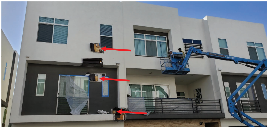
Figure 21. Taken by BSC of wood wall sheathing (i.e. shear walls) at front of Unit 3118 (arrows).
