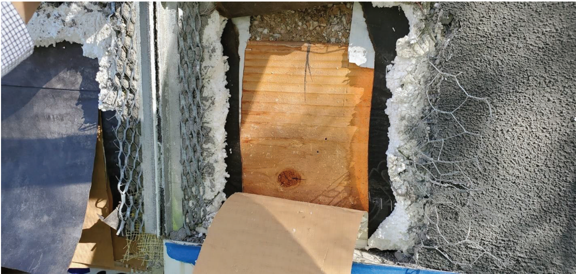
Typical view of destructive investigation work through the stucco cladding and water-resistant barrier (i.e. building paper).
