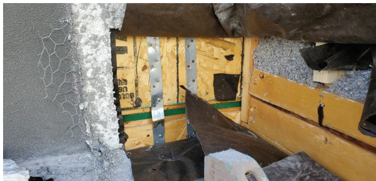
Figure 22. Taken by BSC of wood wall sheathing (i.e. shear wall) at front of Unit 3118.
