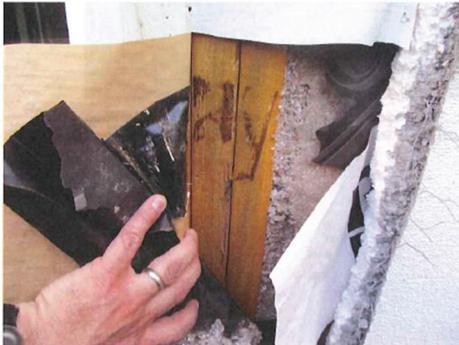
May 13, 2019, Disc IT1, Photograph 156, JBF, south elevation of Building C - Unit 3117, open stud framing with no exterior sheathing.
