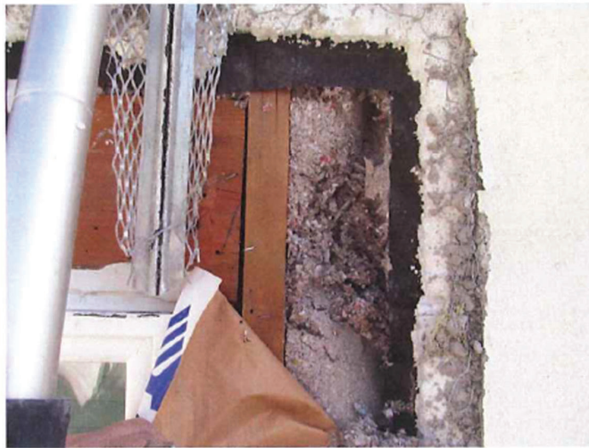
May 14, 2019, Disc IT3, Photograph 52, JBF, south elevation of Building B - Unit 3104, open stud framing with no exterior sheathing.
