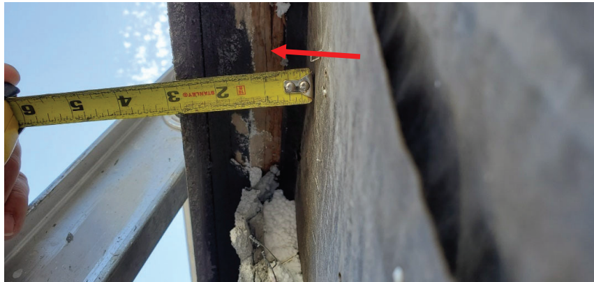
Figure 17. Photograph taken by BSC of the deck (i.e. terrace or balcony) plywood sheathing (arrow) extending to the backside of the metal drip edge.
