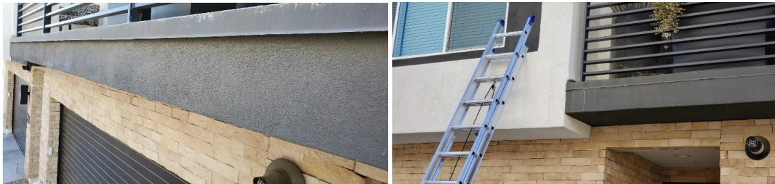
Figure 15. Taken by BSC of balcony condition with stucco installed behind the flashing (left), and stucco installed up against the bottom edge of the flashing (right).
