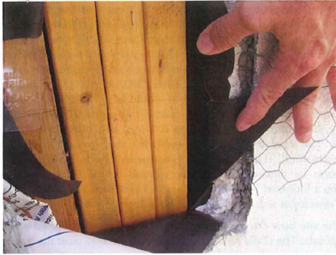
May 14, 2019, Disc IT3, Photograph 26, JBF, north elevation of Building A - Unit 3124, open stud framing with no exterior sheathing.
