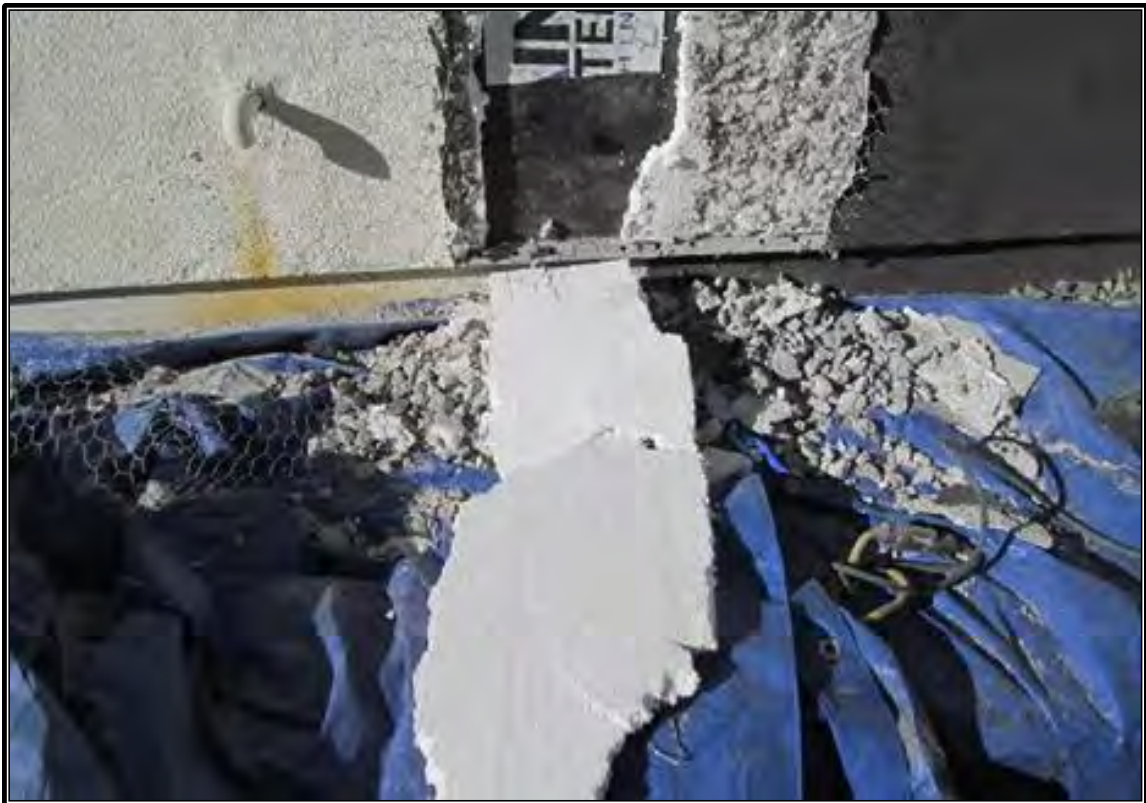
Photo #4 (Pltff Photo Disc IT7 Photo 279): EPS foam board exposed during DT.
