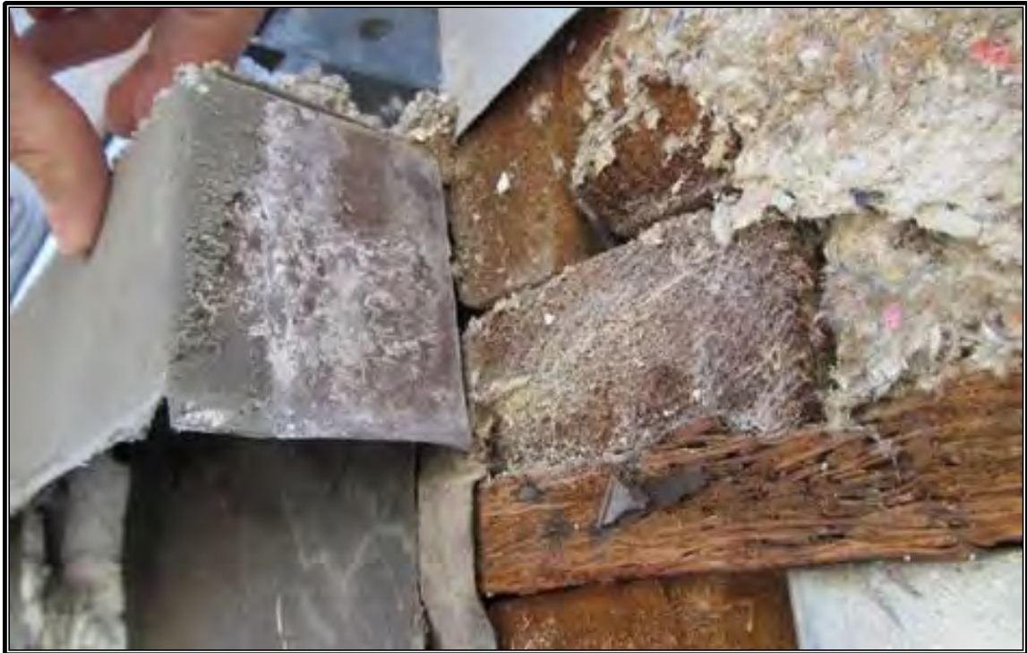
Photo #2 (Pltff Photo Disc ITS Photo 73): Minor staining at exposed framing.
