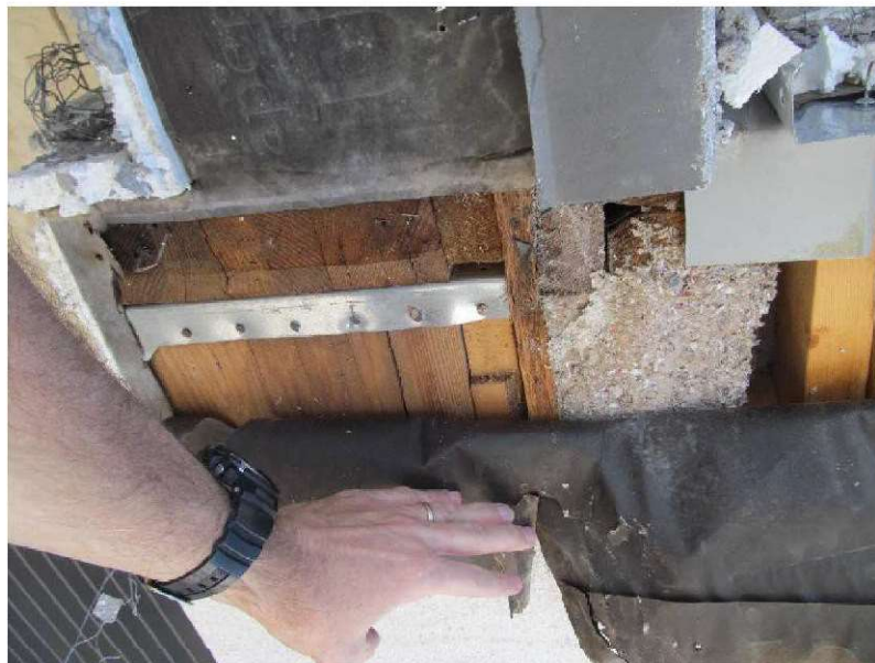
March 9, 2021, Disc IT5, Photograph 72, JFF, Building B, one layer of WRB over framing.
