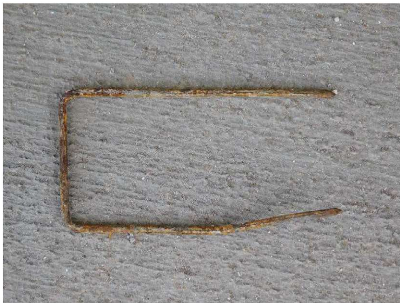
March 10, 2021, Disc IT9, Photograph 90, PER, Building C, rusted staples
