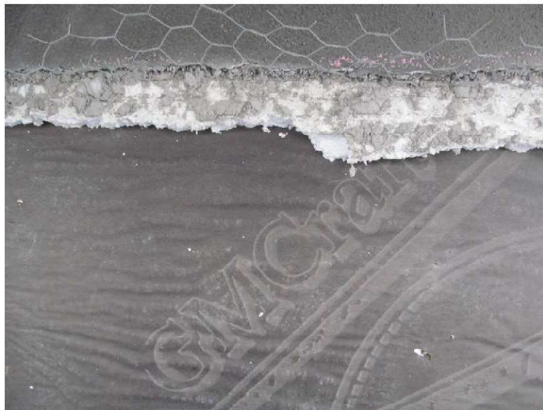
March 9, 2021, Disc IT6, Photograph 271, SSR, Building A, EPS foam board installed tight to GMCraft WRB and vertical grooves generally missing at the inner face.
