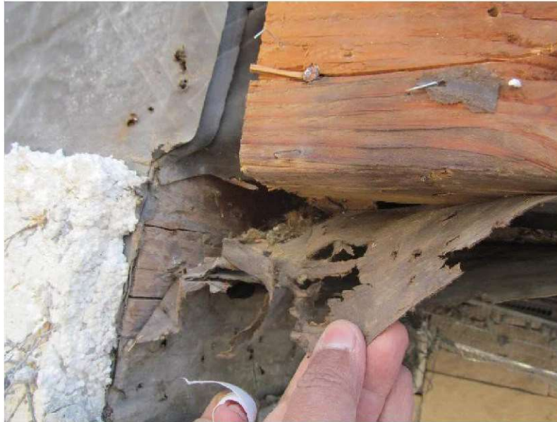
March 10, 2021, Disc IT8, Photograph 120, SSR, Building D, deteriorated WRB over framing with visible stains.
