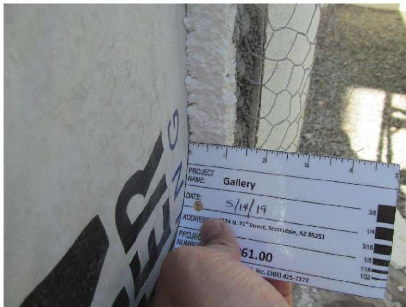
May 14, 2019, Disc IT3, Photograph 18, JBF, Building A, EPS foam board installed tight to WRB and vertical grooves generally missing at the inner face.
