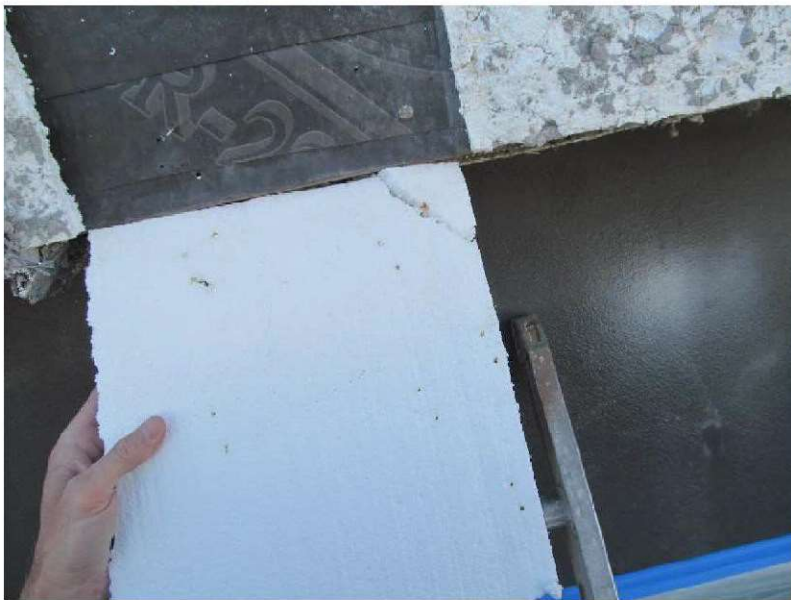
March 10, 2021, Disc IT7, Photograph 226, JJE, Building D, EPS foam board installed over WRB with vertical grooves generally missing at the back face.
