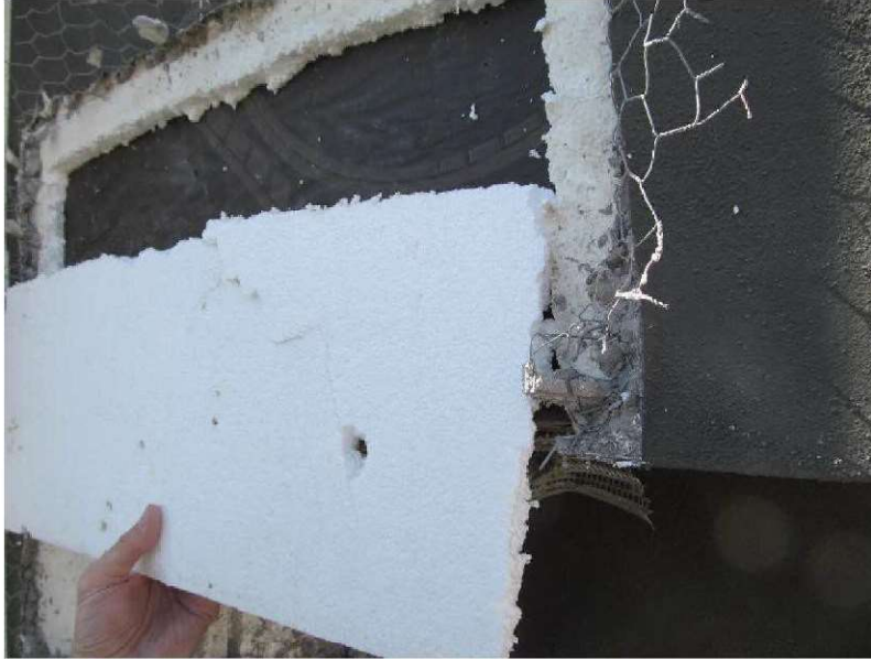
March 10, 2021, Disc IT7, Photograph 117, JJE, Building D, EPS foam board installed over WRB with vertical grooves generally missing at the back face.
