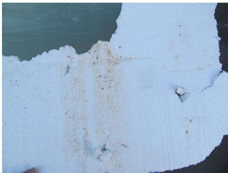
March 10, 2021, Disc IT7, Photograph 210, JJF, Building C, EPS foam board installed tight to WRB and vertical grooves generally missing at the back face.
