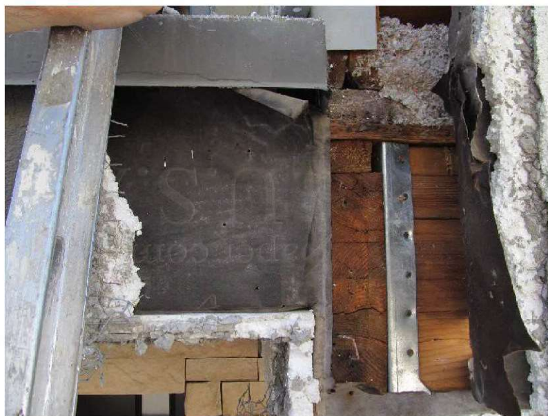
March 9, 2021, Disc IT5, Photograph 75, JFF, Building B, damaged framing due to water intrusion.
