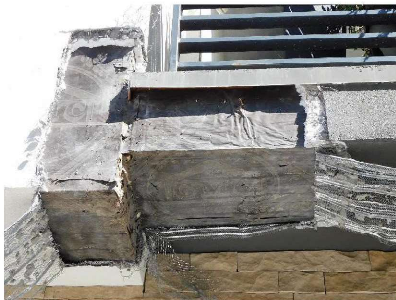
March 10, 2021, Disc IT8, Photograph 101, PER, Building C, deteriorated WRB over framing.
