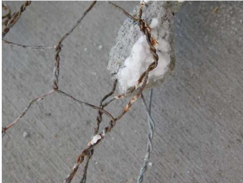
March 10, 2021, Disc IT9, Photograph 92, PER, Building C, rusted lath
