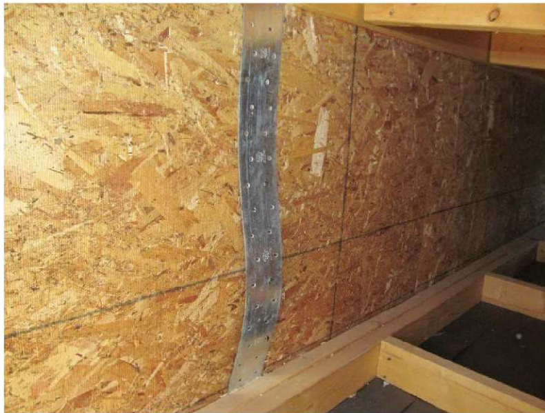
March 10, 2021, Disc IT8, Photograph 278, SSR, Building D - Unit 3111, CS-16 metal strap is disengaged and buckled.
