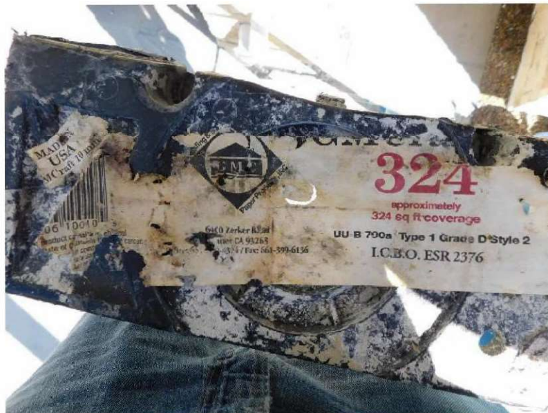
March 10, 2021, Disc IT9, Photograph 124, SSR, Building C, manufacturer's label shows the building paper is Type 1, Grade D, Style 2 building paper with 10-minute water resistance and references ESR 2376.
