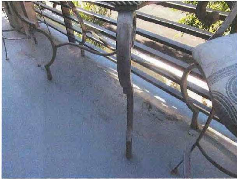
December 19, 2018, Disc OBS1, Photograph 167, JBF, Building A - Unit 3124, evidence of water ponding is present at leading edge of balcony.
