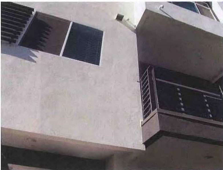
December 19, 2018, Disc OBS1, Photograph 82, JBF, east elevation of Building D - Units 3109 & 3111, no weep mechanism at base of stucco at soffits.
