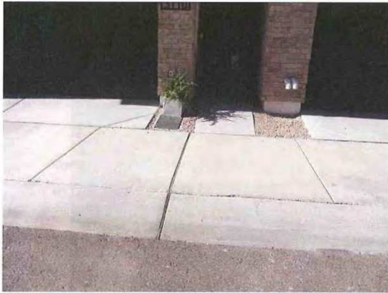
December 19, 2018, Disc OBS1, Photograph 154, JBF, east elevation of Building B, drainage adjacent to foundation bound by concrete flatwork.
