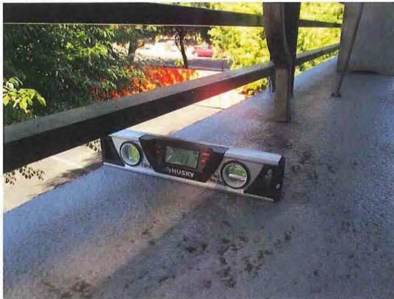
December 19, 2018, Disc OBS1, Photograph 163, JBF, Building A - Unit 3124, balcony slope measured to be 1.1-percent away from leading edge and evidence of water ponding is present.
