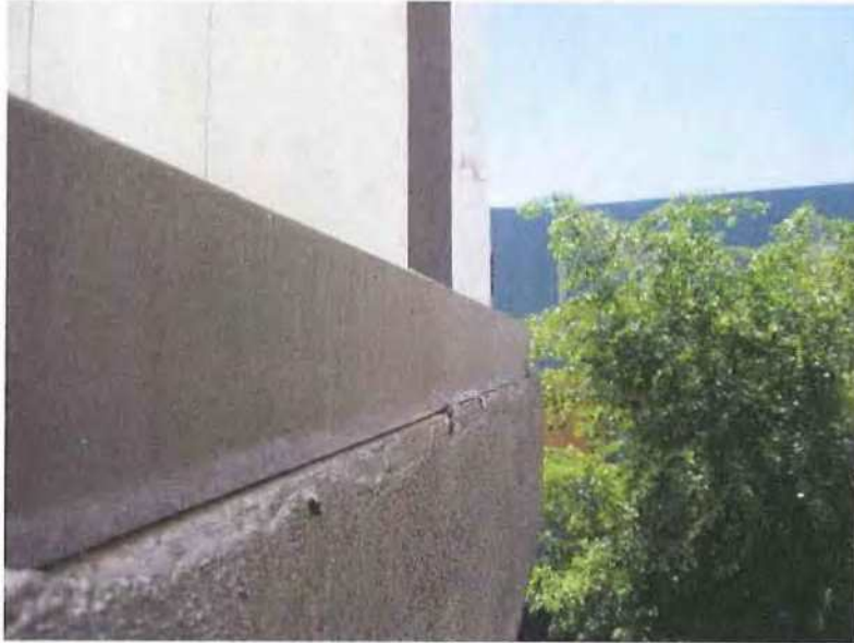
May 13, 2019, Disc IT1, Photograph 110, JBF, north elevation of Building B - Unit 3116, metal flashing at leading edge of roof is inset from stucco.
