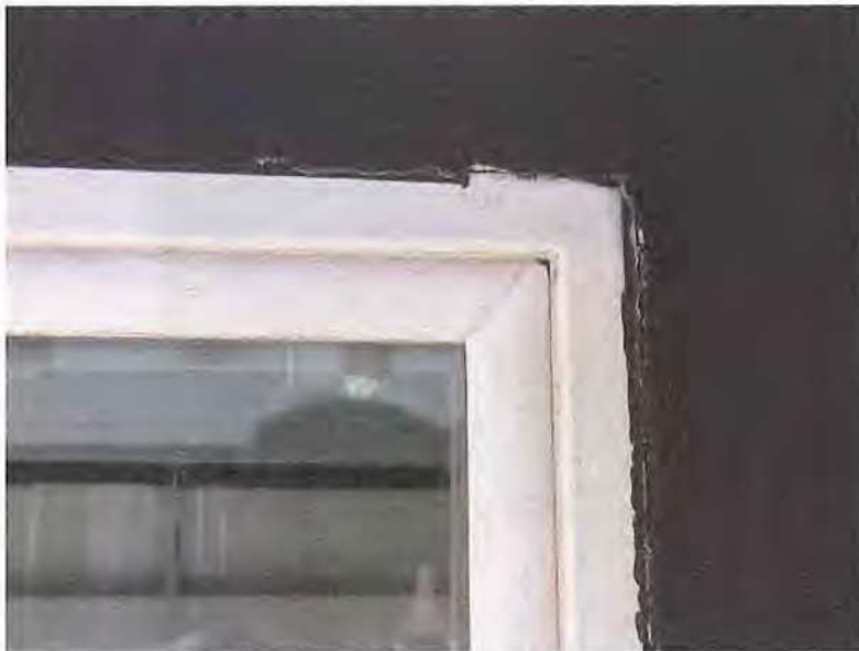
May 13, 2019, Disc IT2, Photograph 33, ELF, west elevation of Building D - Unit 3115, no expansion joints provided between stucco and window. Cracking is present at this interface.
