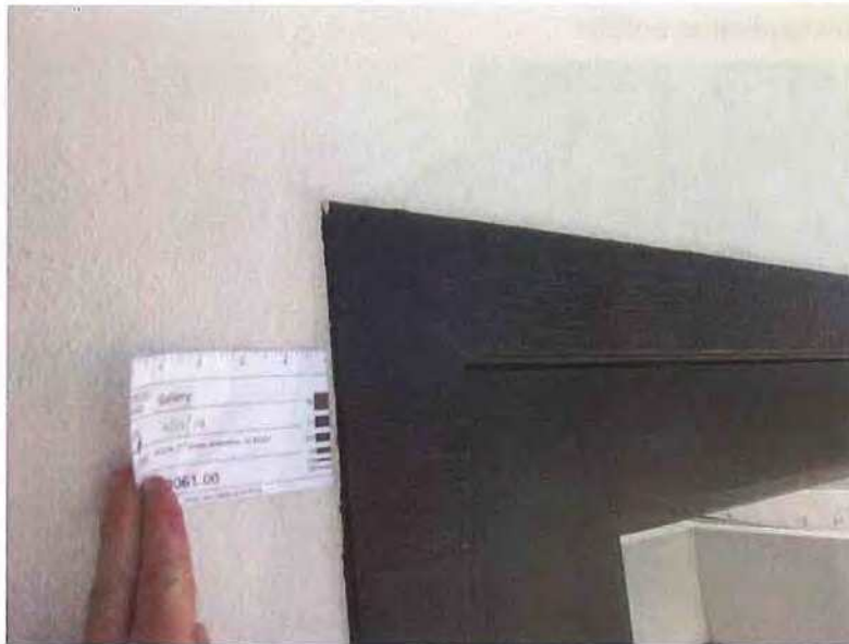
May 13, 2019, Disc IT2, Photograph 50, ELF, Building A - Unit 3122, no expansion joints provided between stucco and wood trim.
