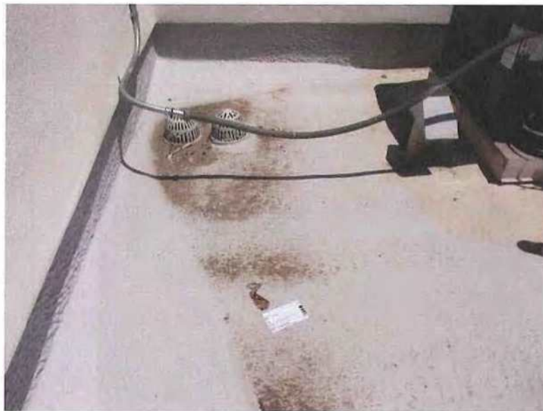
May 13, 2019, Disc IT2, Photograph 79, ELF, Building A - Unit 3122, insufficient slope of roof at drain resulting in ponding water.
