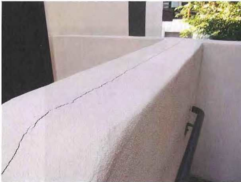
December 19, 2018, Disc OBS1, Photograph 134, JBF, west stairs between Buildings A and B, cracking and separation of stair wall indicative of differential movement.
