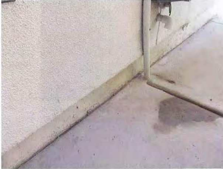
December 19, 2018, Disc OBS1, Photograph 136, JBF, south elevation of Building A - Unit 3118, no isolation joint between concrete flatwork and structural foundation.
