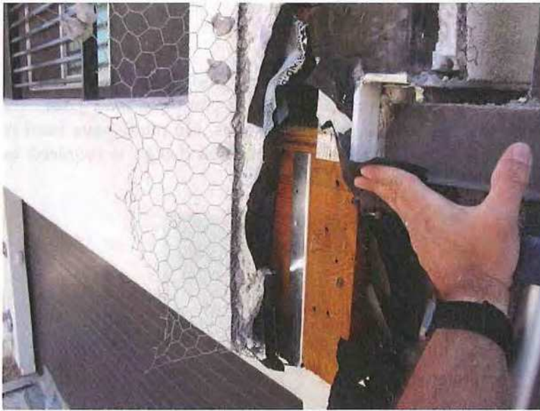
May 13, 2019, Disc IT1, Photograph 50, JBF, west elevation of Building D - Unit 3113, open stud framing with no exterior sheathing.
