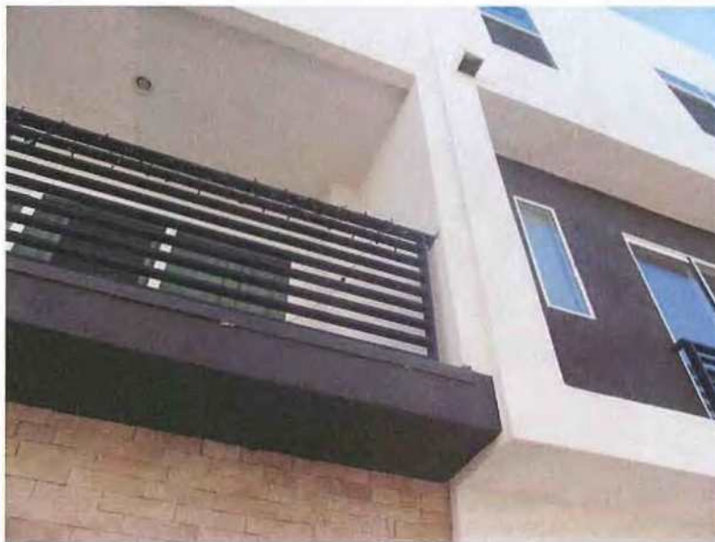
December 19, 2018, Disc OBS1, Photograph 24, JBF, west elevation of Building D - Units 3111 & 3113, no weep mechanism at base of stucco at soffits.
