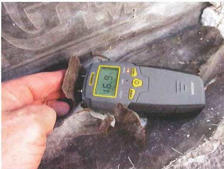
May 14, 2019, Disc IT4, Photograph 13, ELF, west elevation of Building C – Unit 3123, high moisture content in building paper below stucco over self-adhered membrane.
