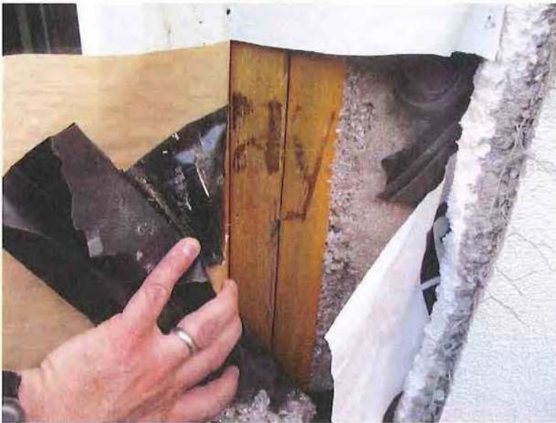
May 13, 2019, Disc IT1, Photograph 156, JBF, south elevation of Building C - Unit 3117, open stud framing with no exterior sheathing.
