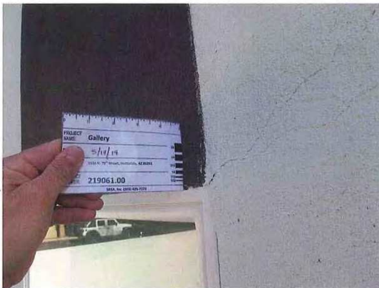
May 14, 2019, Disc IT3, Photograph 12, JBF, south elevation of Building B - Unit 3104, no expansion joints provided between stucco and window. A diagonal stucco crack is present at this location.
