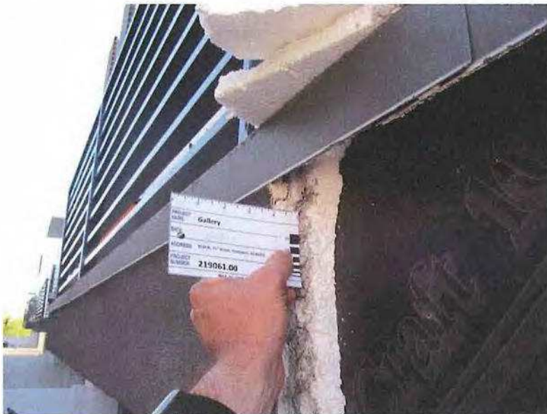
May 13, 2019, Disc IT1, Photograph 176, JBF, east elevation of Building C - Unit 3127, one layer of GMCraft 10 paper does not provide minimum water-resistance rating of 60-minutes in accordance with ESR-3529.
