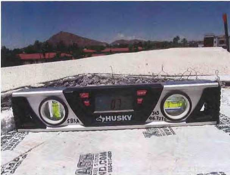
May 13, 2019, Disc IT1, Photograph 98, JBF, Building C - Unit 3125, stucco does not slope at parapet cap.
