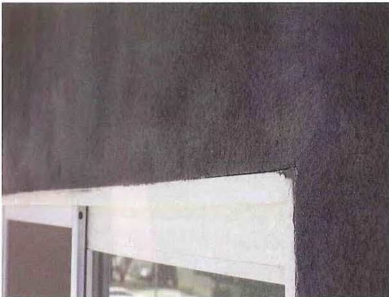
May 13, 2019, Disc IT2, Photograph 34, ELF, west elevation of Building D - Unit 3115, no sheet metal flashing at head of window opening.
