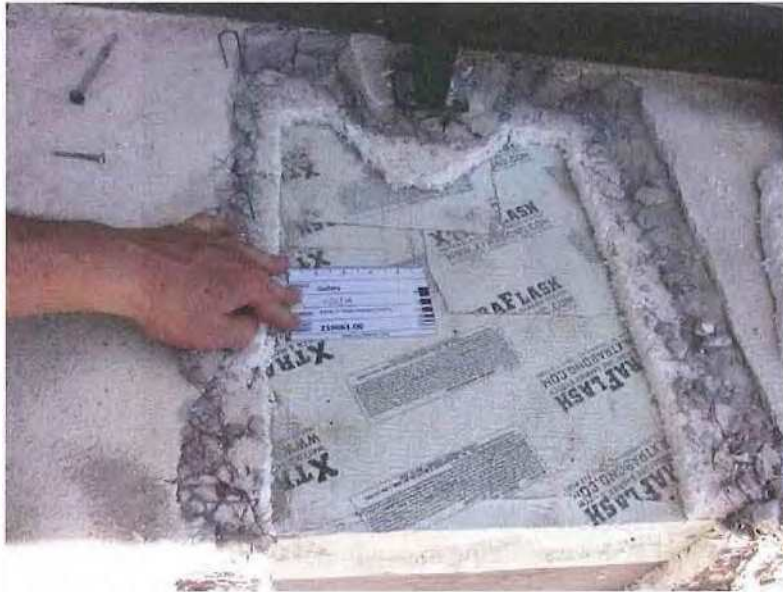
May 13, 2019, Disc IT2, Photograph 21, ELF, west elevation of Building D – Unit 3115, XtraFlash membrane under stucco. Stain through holes in membrane.
