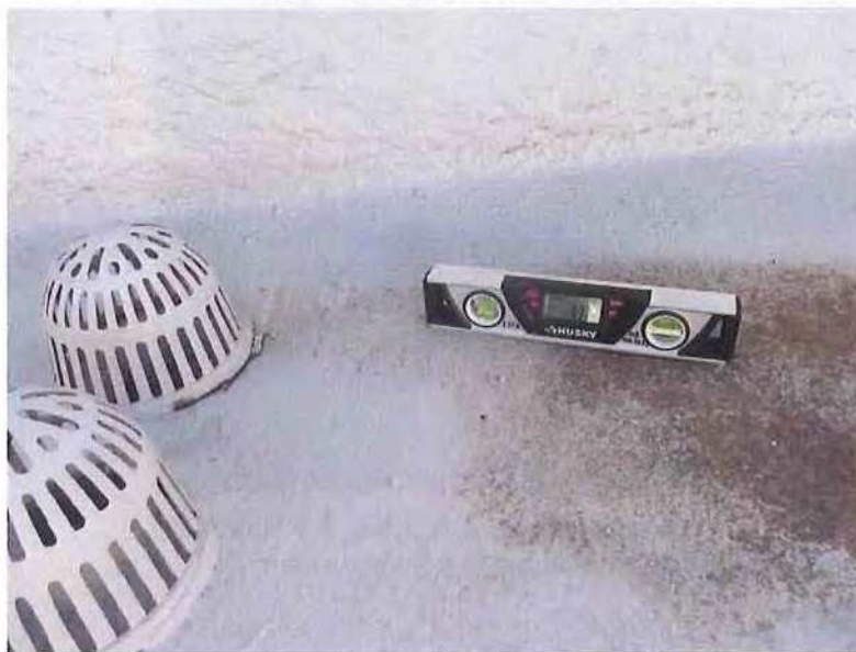
December 19, 2018, Disc OBS1, Photograph 176, JBF, Building A - Unit 3124, roof slope measured to be 1.7-percent away from drain and evidence of water ponding is present.
