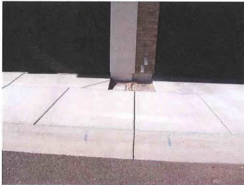
December 19, 2018, Disc OBS1, Photograph 157, JBF, east elevation of Building A, condensate from high efficiency units drain water adjacent to foundation bound by concrete flatwork into the electrical vault.
