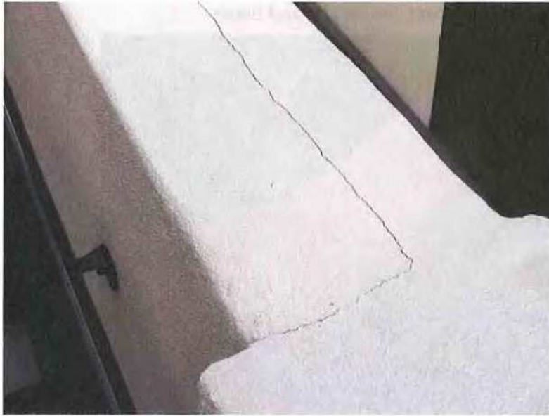
December 19, 2018, Disc OBS1, Photograph 132, JBF, west stairs between Buildings A and B, cracking and separation of stair wall.
