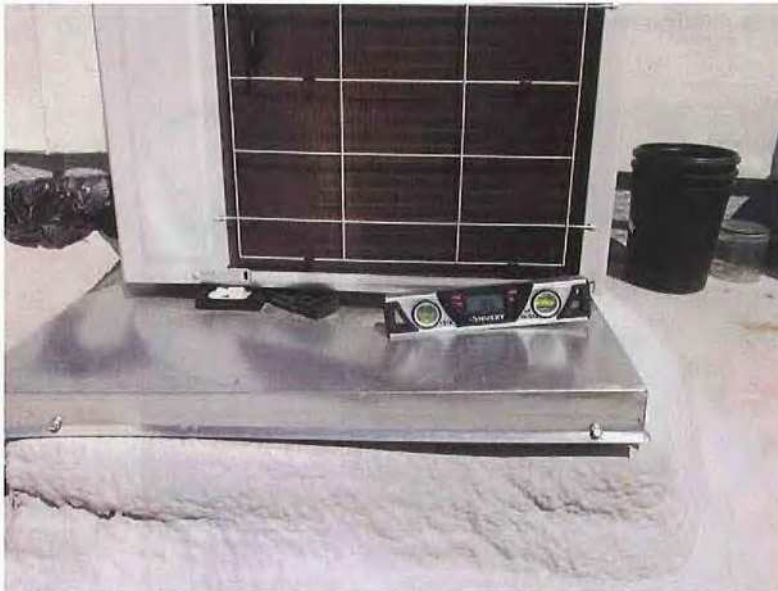
May 13, 2019, Disc IT2, Photograph 146, ELF, Building B - Unit 3110, roof built-up and flashing provided to accommodate additional air conditioner after original construction. Surface is uneven and inadequate for support of air conditioner unit.
