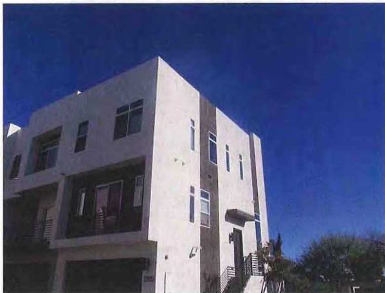
December 19, 2018, Disc OBS1, Photograph 5, JBF, south elevation of Building D, vertical control joint only provided at corners of windows. This was common of north and south elevations at all buildings.
