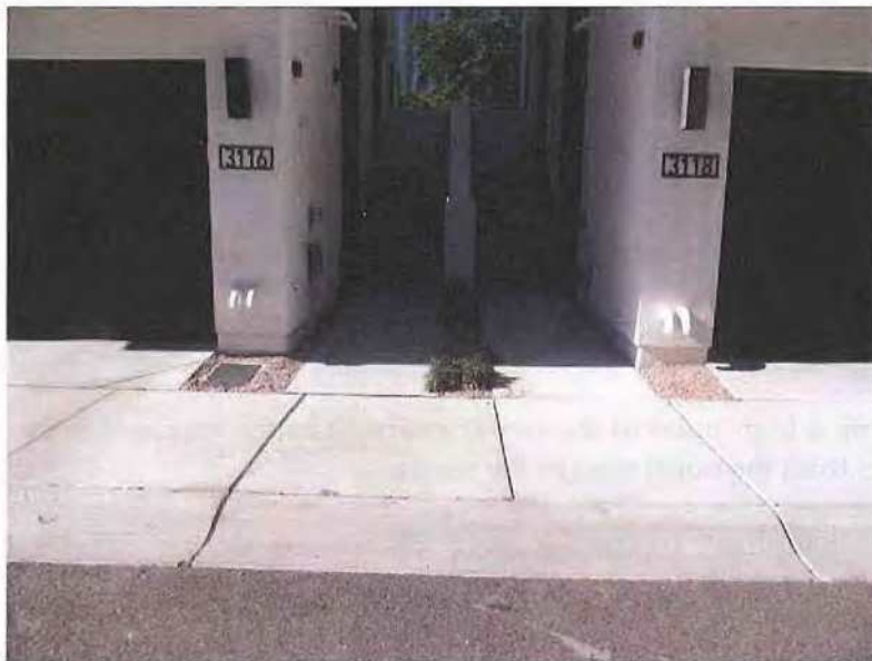
December 19, 2018, Disc OBS1, Photograph 156, JBF, west elevation between Buildings C and D, poor slope of grade between buildings.
