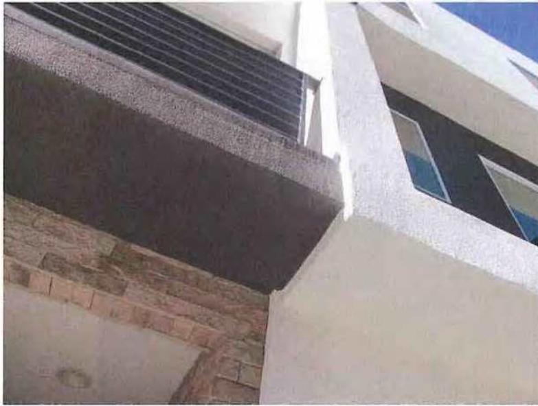
December 19, 2018, Disc OBS1, Photograph 129, JBF, east elevation of Building A - Units 3122 & 3124, no weep mechanism at base of stucco at soffits.
