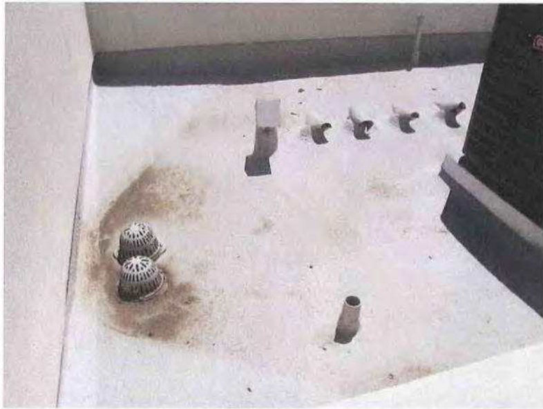
May 13, 2019, Disc IT1, Photograph 29, JBF, Building C - Unit 3125, insufficient slope of roof at drain resulting in ponding water.
