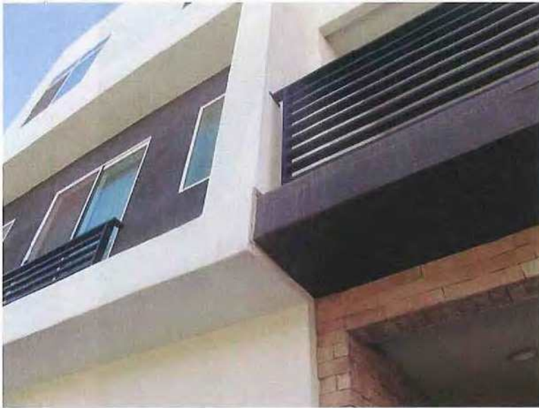
December 19, 2018, Disc OBS1, Photograph 61, JBF, west elevation of Building C - Units 3125 & 3127, no weep mechanism at base of stucco at soffits.
