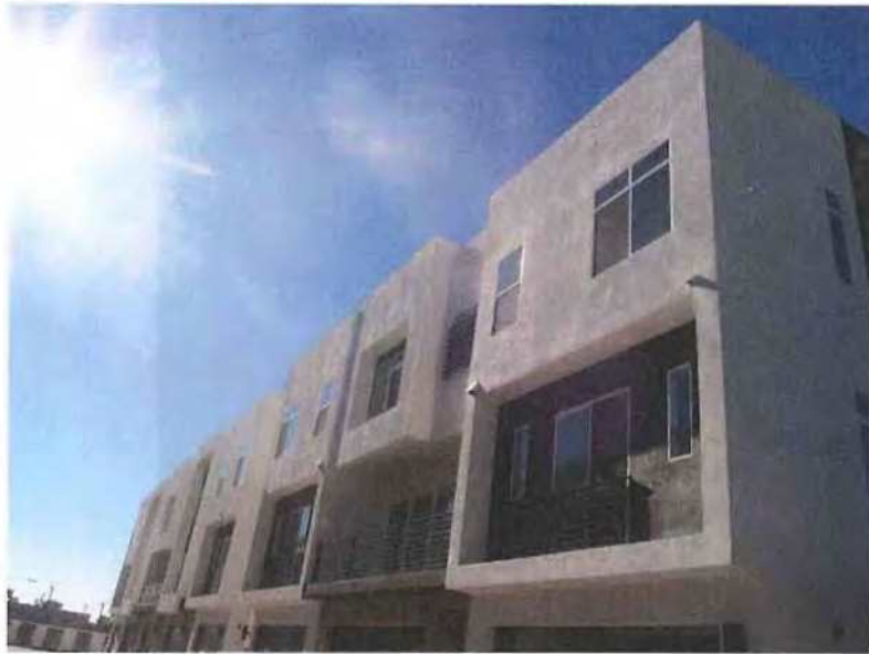
December 19, 2018, Disc OBS1, Photograph 110, JBF, east elevation of Buildings A and B, no control/movement joints provided.
