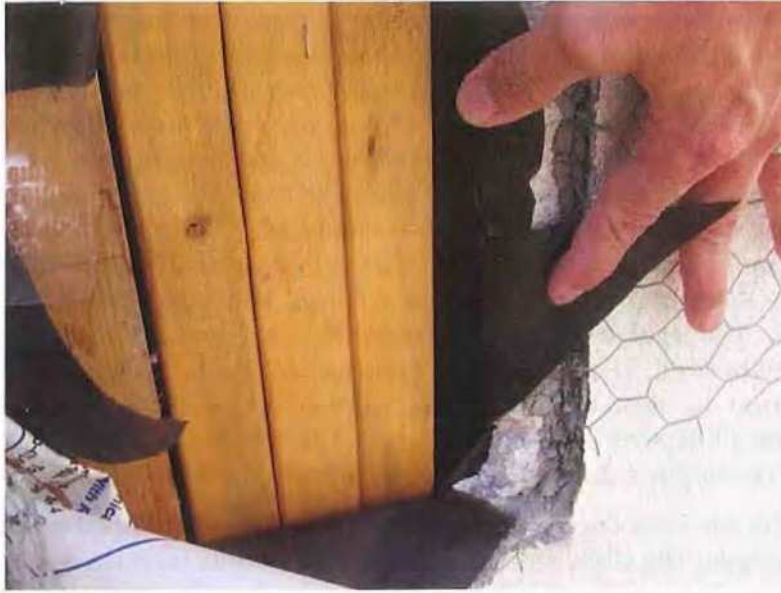
May 14, 2019, Disc IT3, Photograph 26, JBF, north elevation of Building A - Unit 3124, open stud framing with no exterior sheathing.
