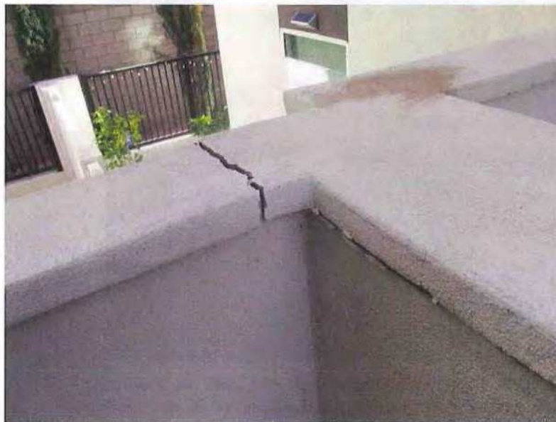
December 19, 2018, Disc OBS1, Photograph 47, JBF, east stairs between Buildings C and D, cracking and separation of stair wall indicative of differential movement.
