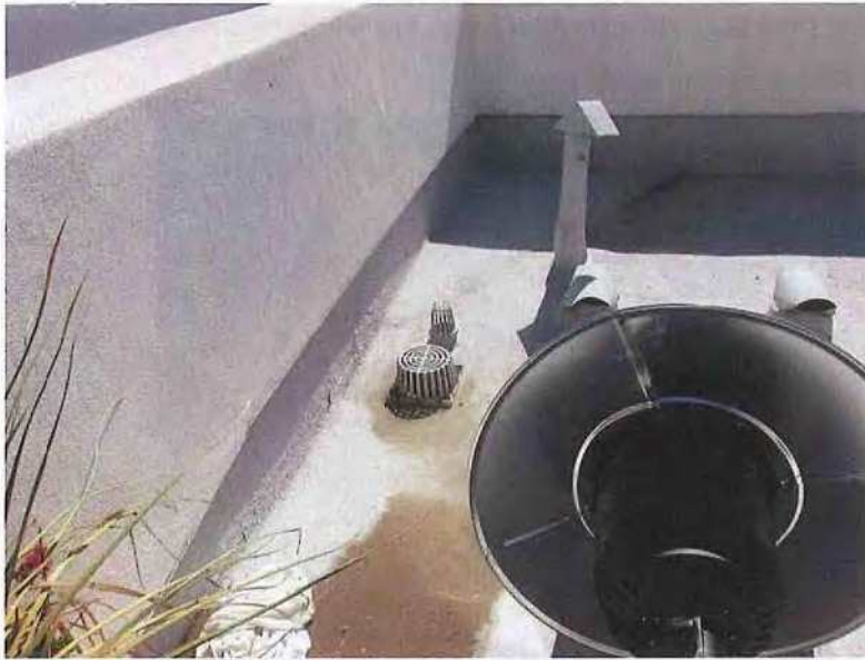
May 14, 2019, Disc IT4, Photograph 58, ELF, Building D - Unit 3113, insufficient slope of roof at drain resulting in ponding water.
