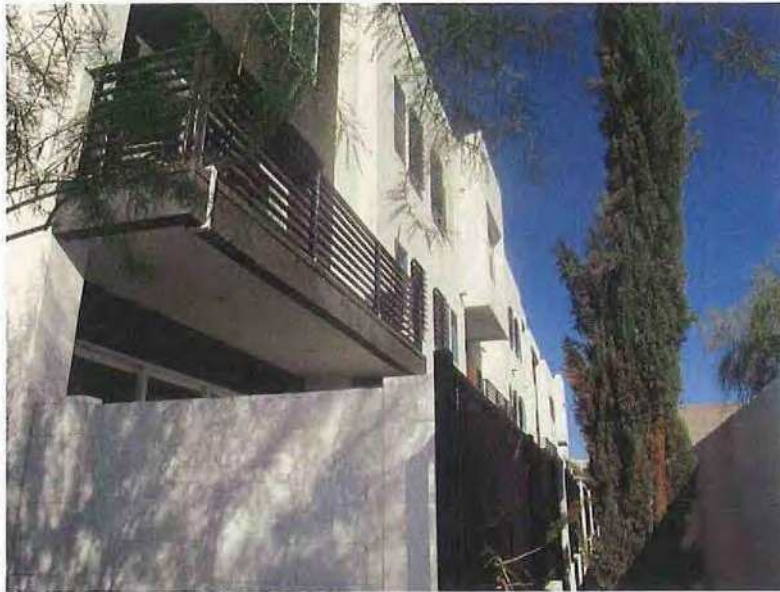
December 19, 2018, Disc OBS1, Photograph 13, JBF, east elevation of Buildings C and D, no control/movement joints provided.
