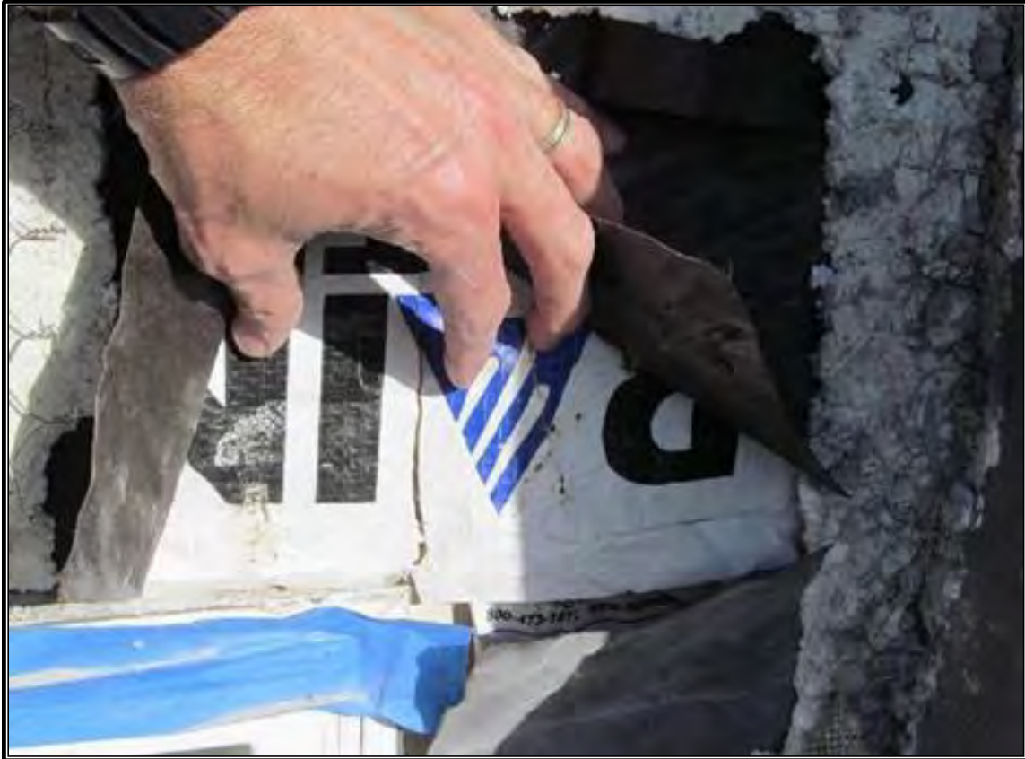
Photo #3 (Pltff Photo Disc ITS Photo 178): One layer of WRB over sheathing.
