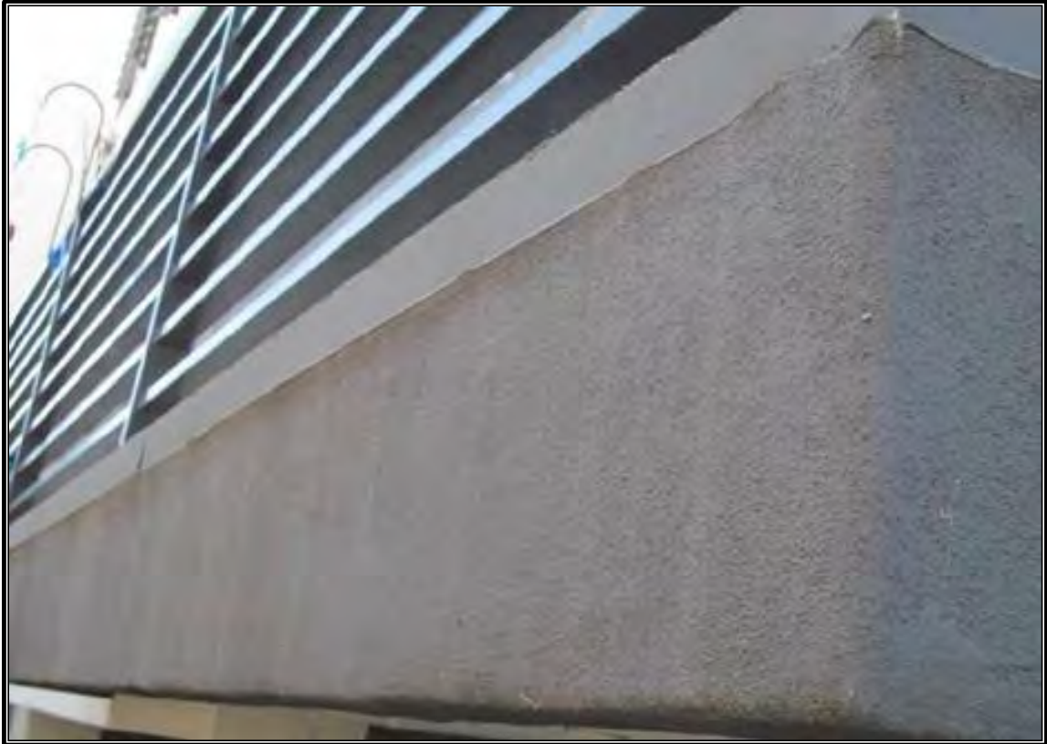
Photo #6 (Pltff Photo Disc IT7 Photo 182): Deck edge flashing at stucco.
