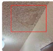
Water damage outside main entry in common hallway
