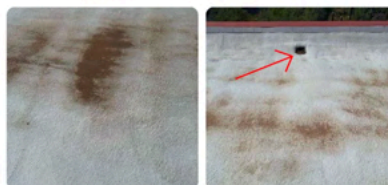
Partially clogged scupper drain
