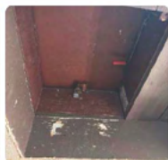
Locked roof access
