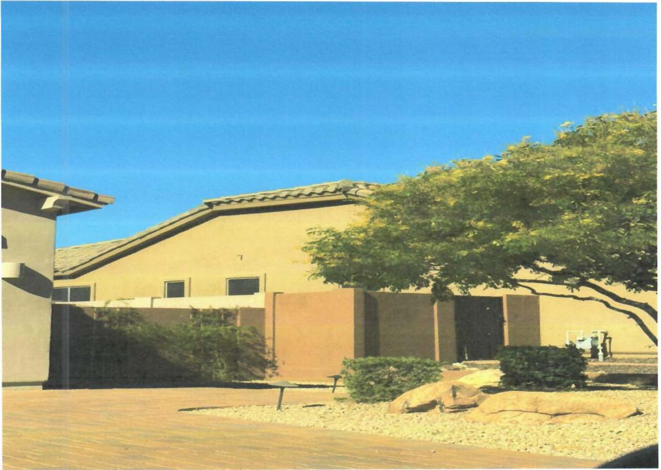
Fading and mismatched repaint areas contributing to an overall uneven appearance.
