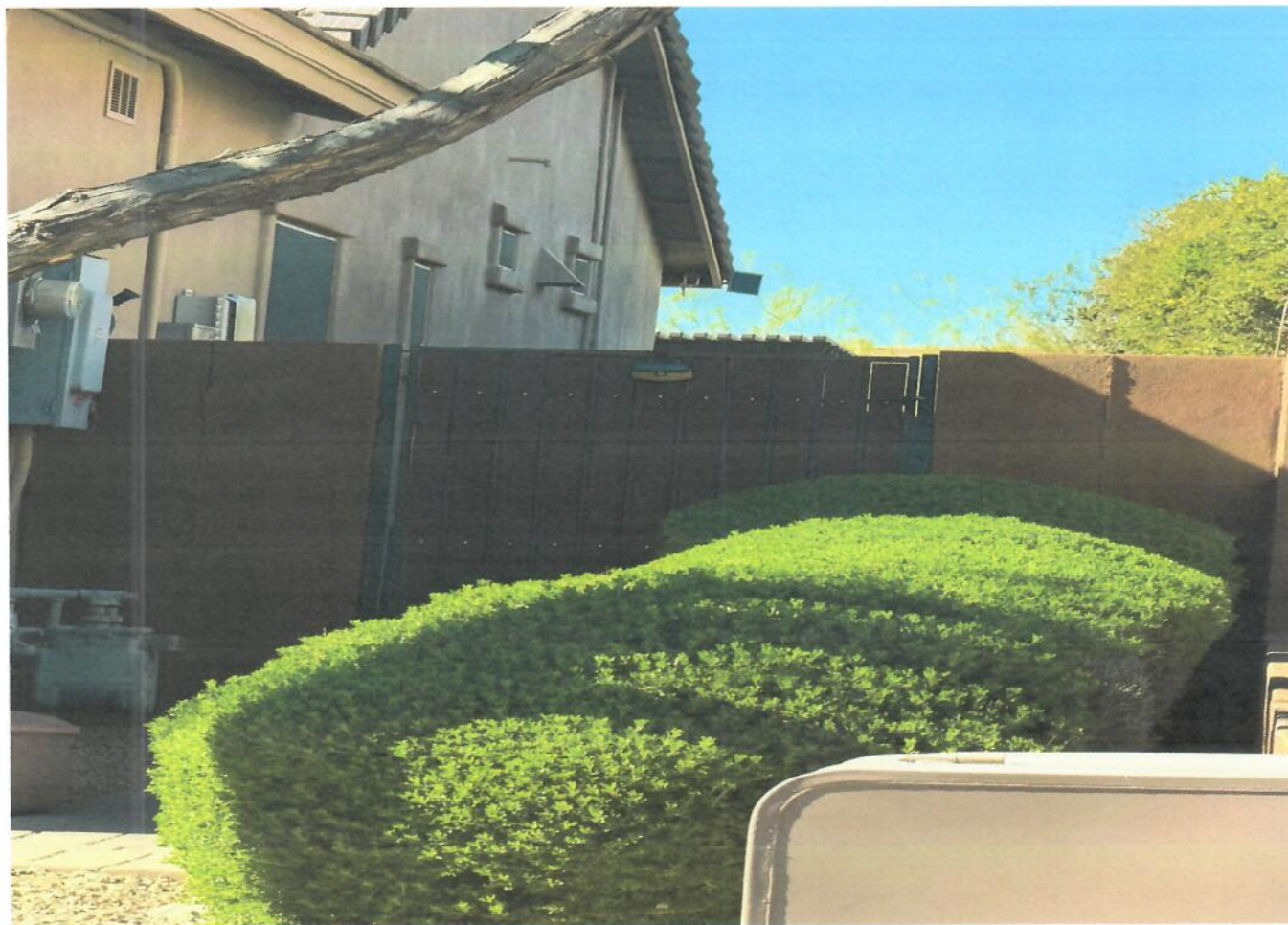
Uneven paint coverage and variation in finish quality across wall sections.
