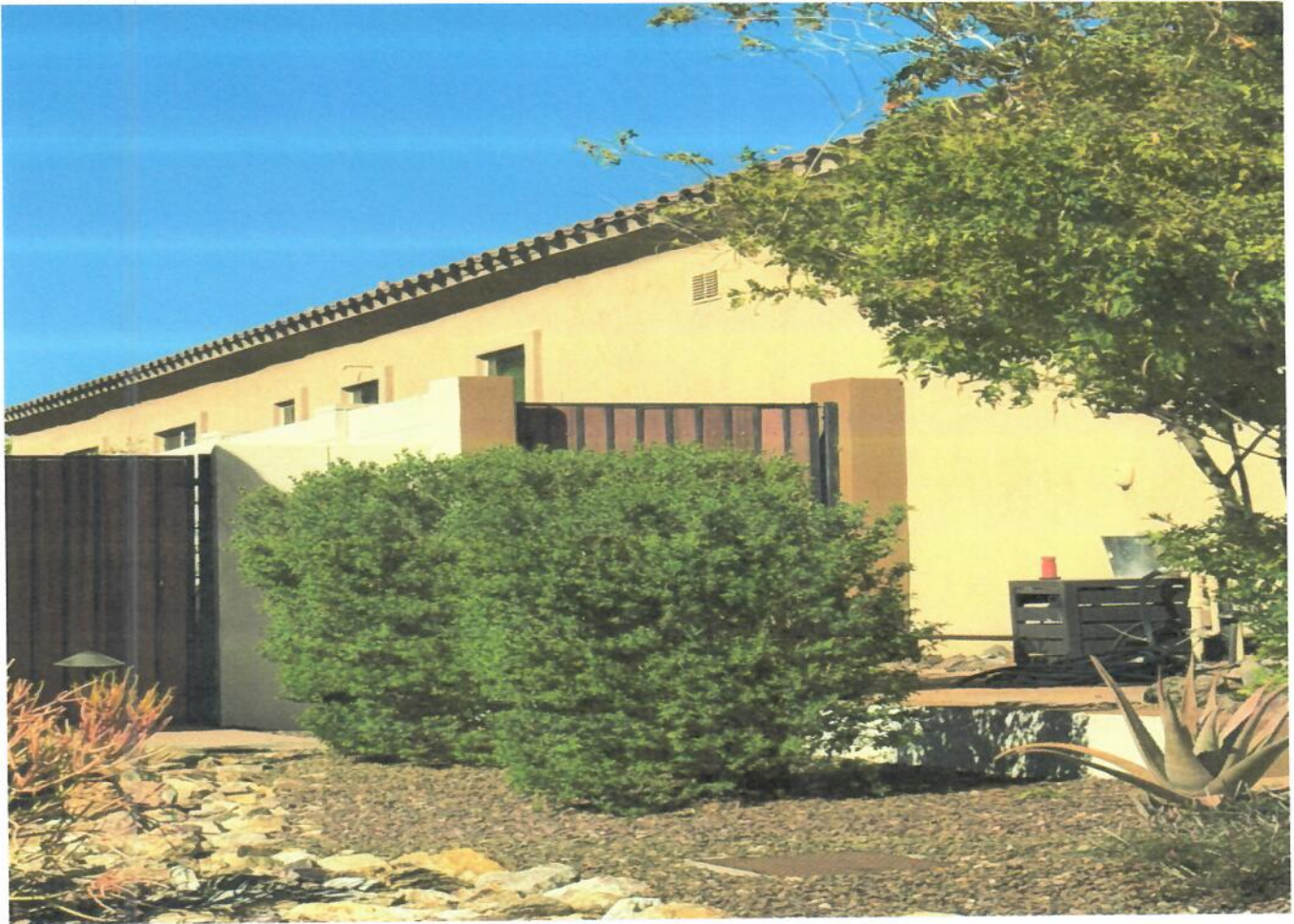
Visible variation in wall color tone between adjacent sections, demonstrating lack of uniformity.
