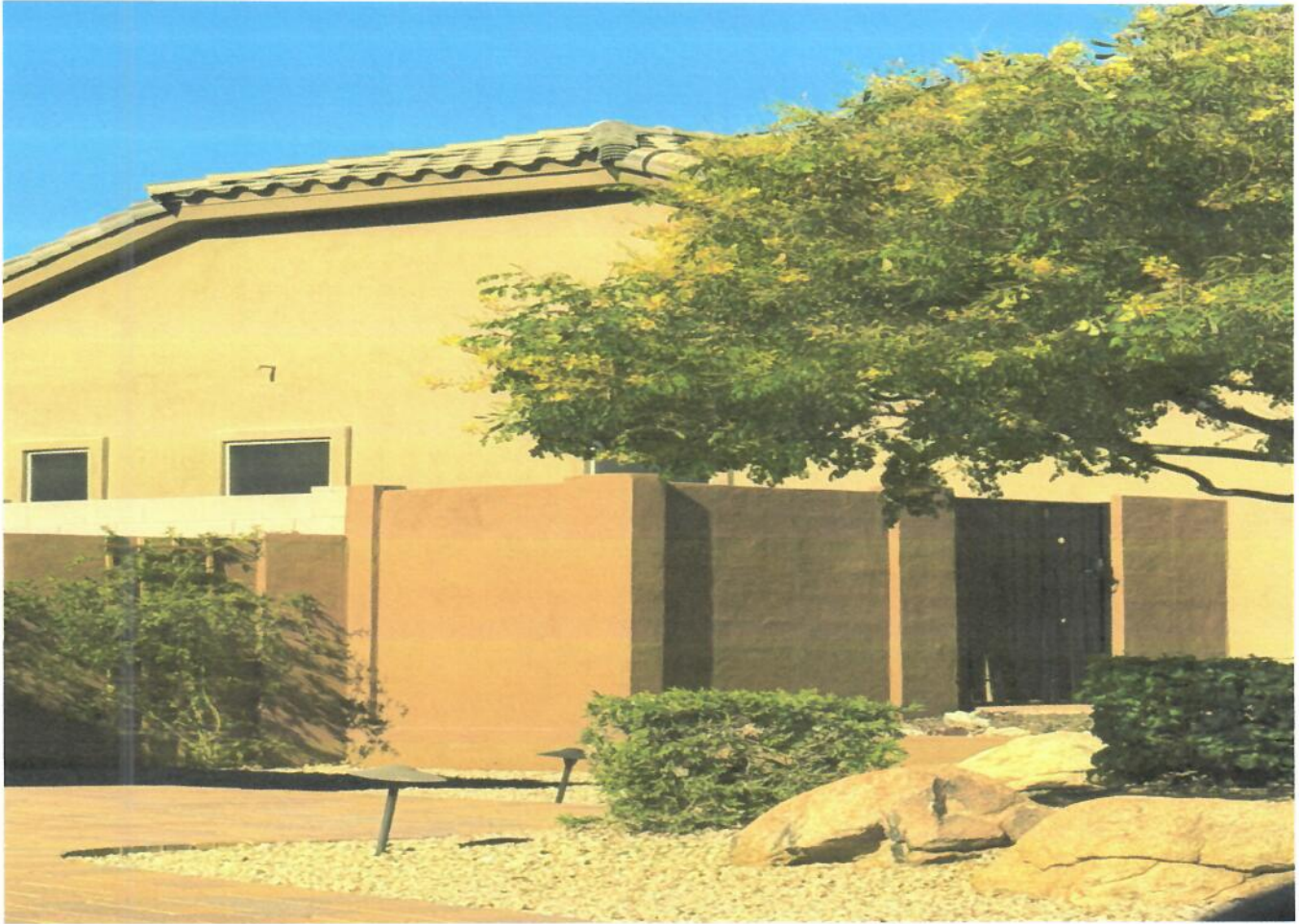
Adjacent properties displaying differing wall tones despite intended standardization.
