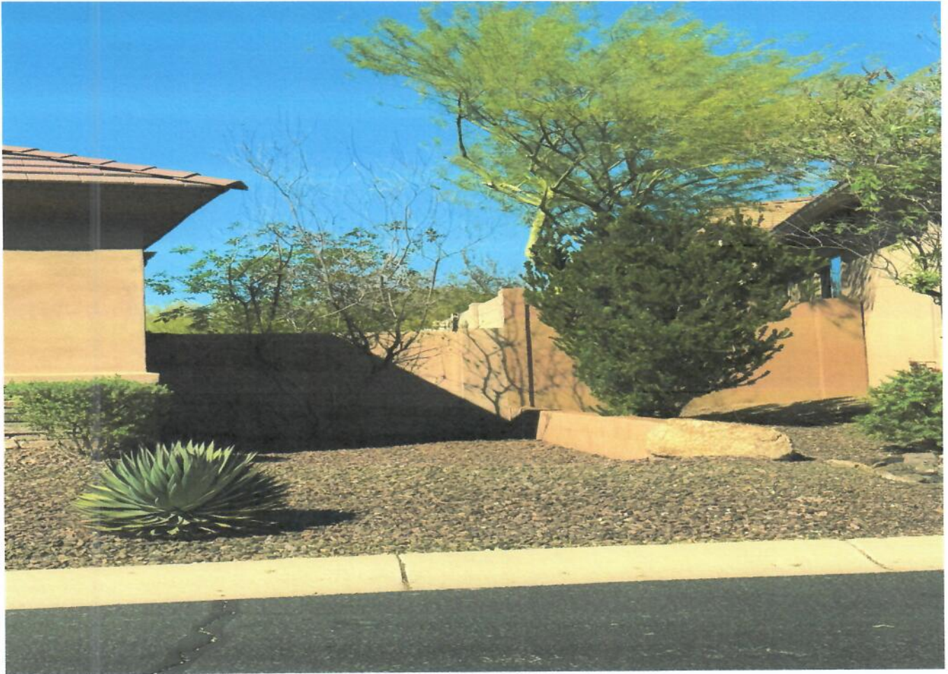
Patchwork effect where repainting does not match surrounding wall sections.
